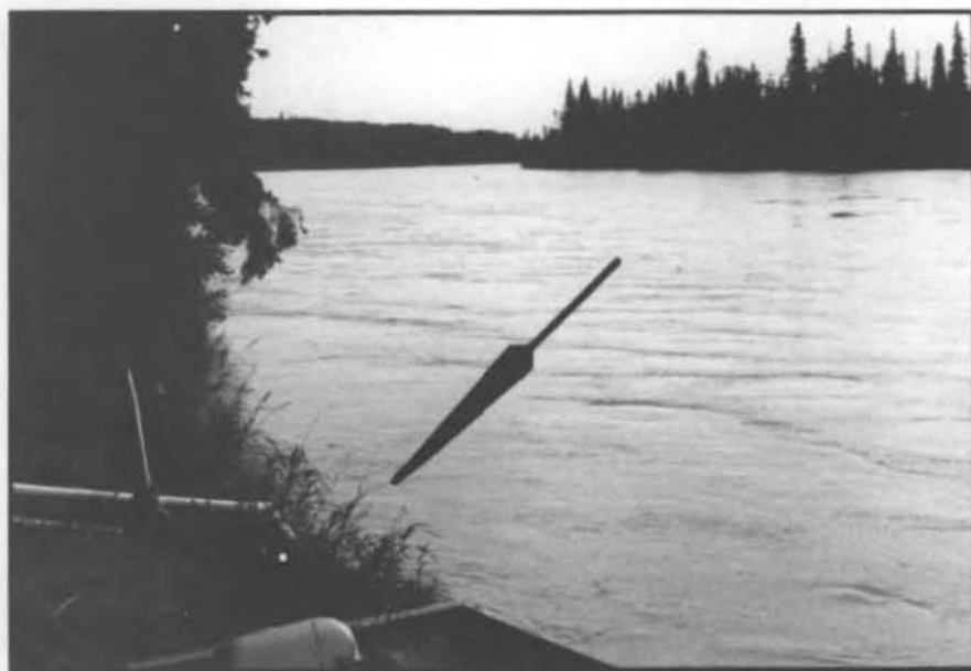
Figure 5. Intake piping (arrow) for pilot plant where it comes ashore.
