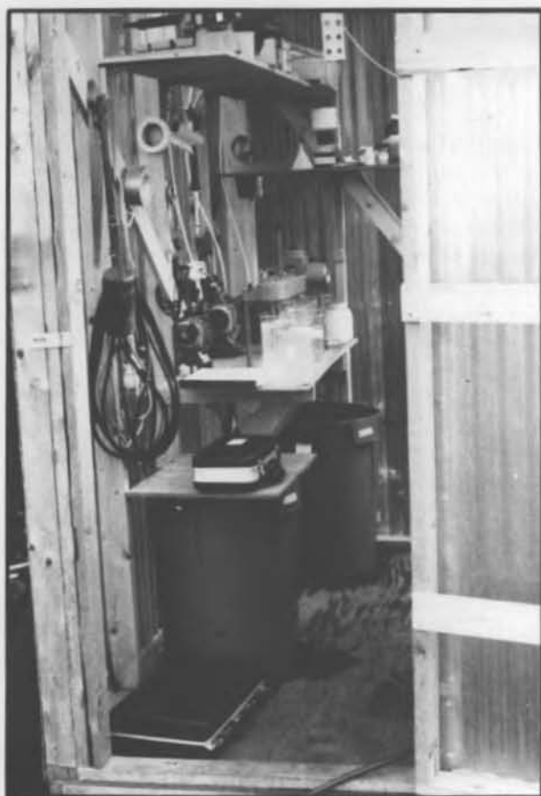
a. Metering pumps on bench above storage containers.
