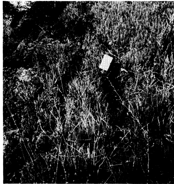
b. Crack formed on top of the ground surface delineating a future slump block.
