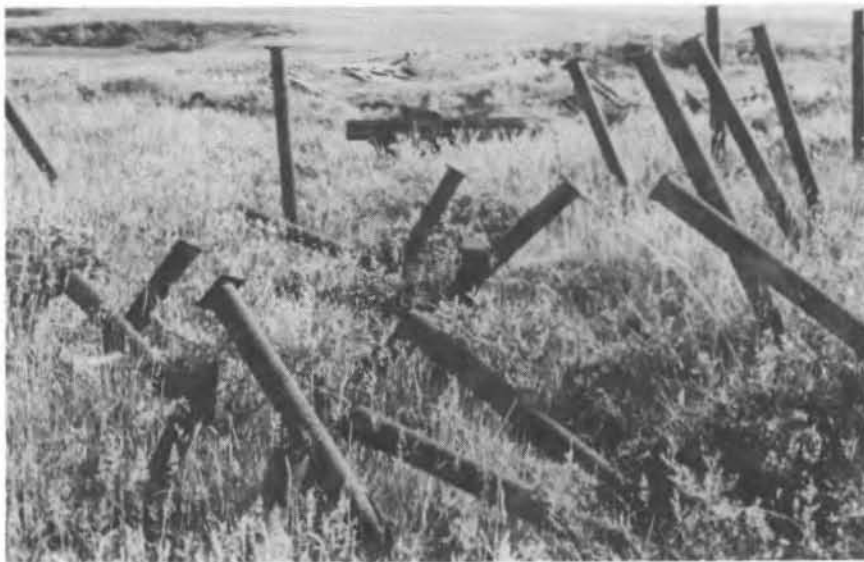
b. Tilted steel pilings that formerly supported a camp building (disturbance groups 3 and 2).
