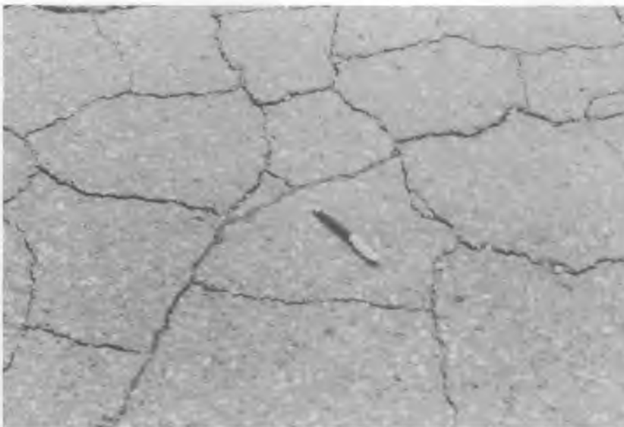
Figure 2. Alligator (or map) cracking.
