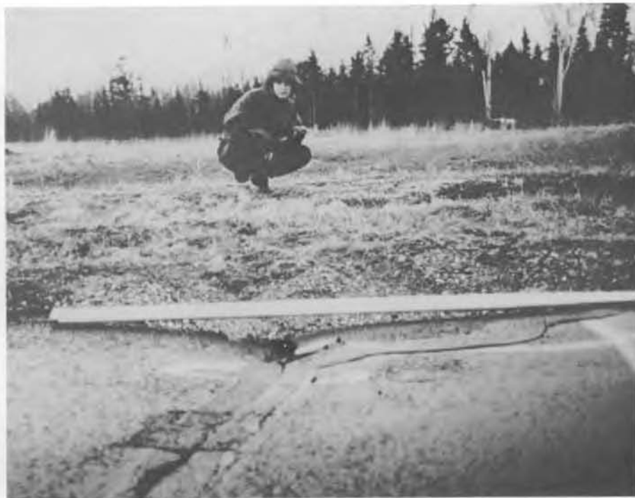
c. Settlement of pavement at station 29+95
