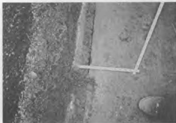
b. Gap between insulation panels
