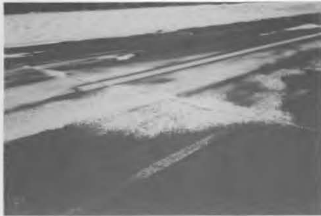
Figure 19. Variation in pavement surface temperature due to the presence of a crack.
