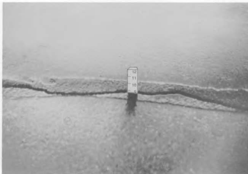
b. Crack at station 16+15.
