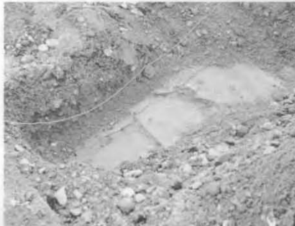
Figure 17. Overlapping and damaged insulation.
