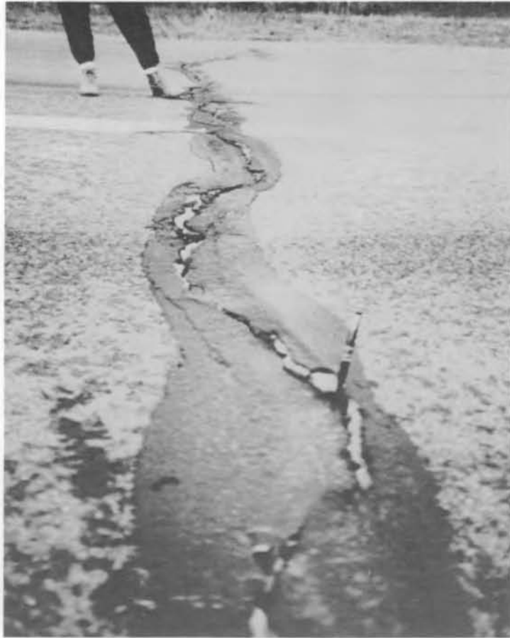
a. Crack at station 8+22 initially sealed with silicone, then with a rubberized crack sealer.
