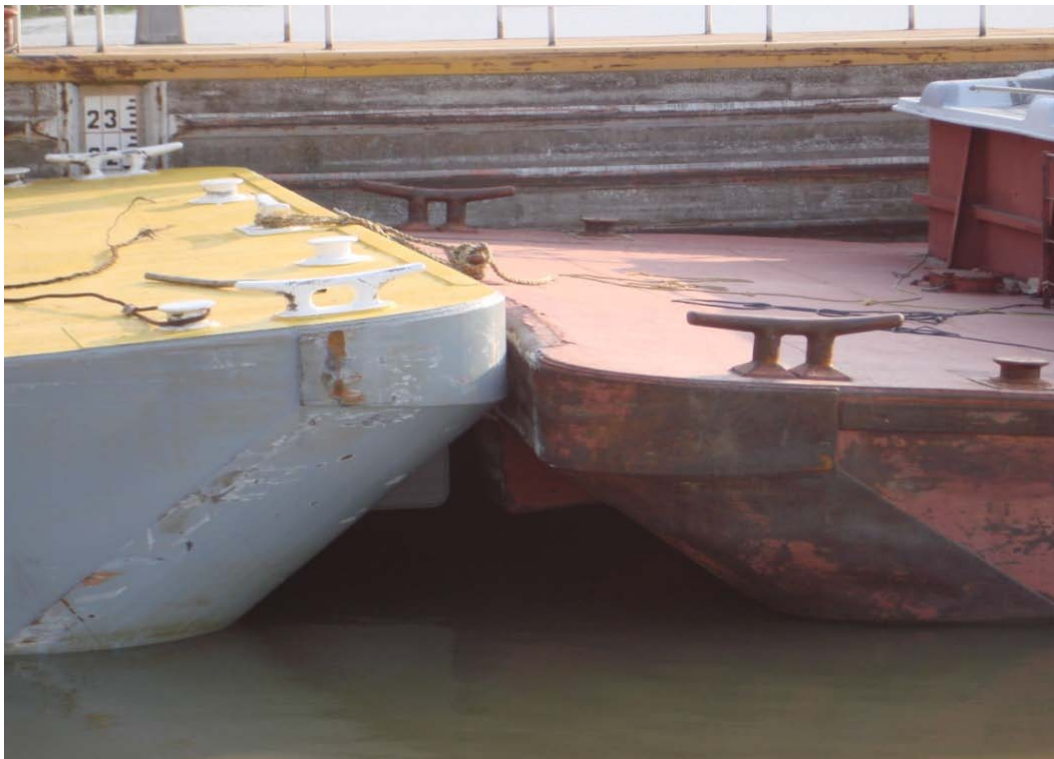
Figure 2.20. View of damage to barges that hit the guide wall at Newt Graham Lock and Dam 18.
