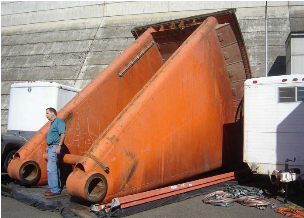
Figure 52. Double skin plate reverse tainter valve waiting for repair, The Dalles Lock.
