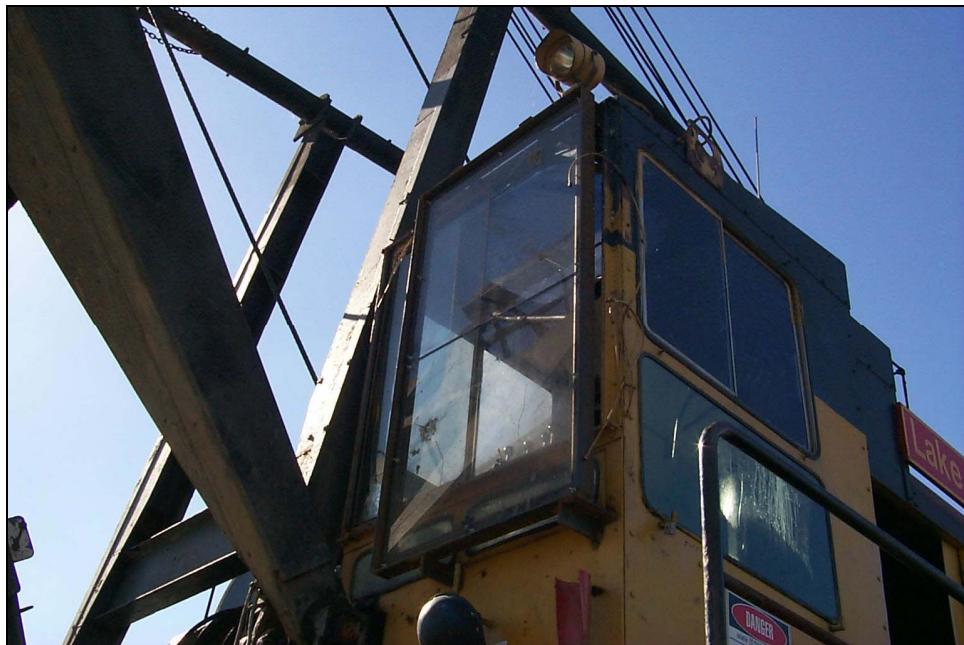
Figure 7. Crane operator's protective barrier
