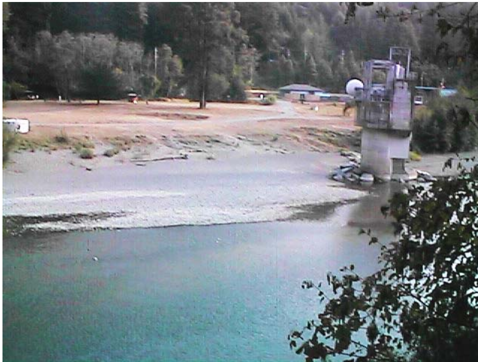
Figure D11. Raney collector near HBMWD operations building, Sept. 17, 1999
