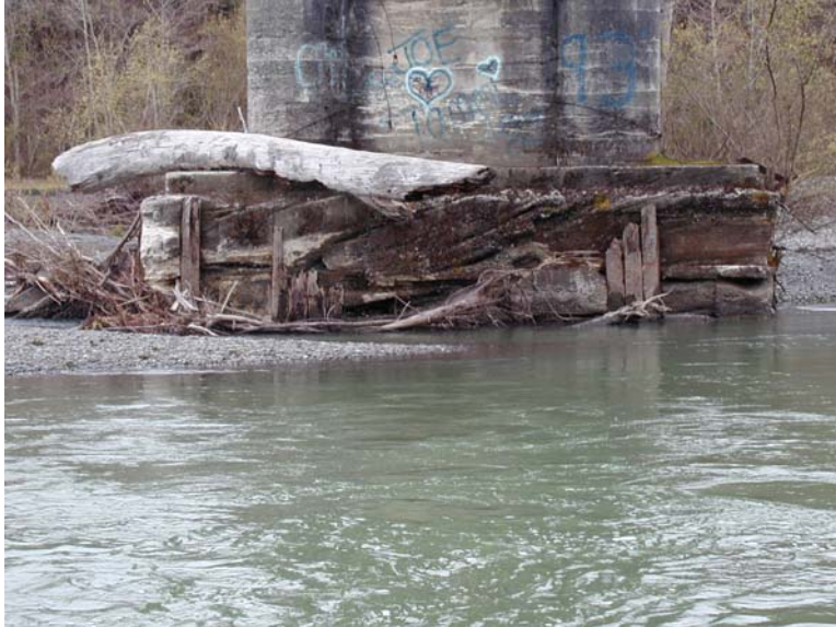
Figure C42. XC21 (right bank) - Looking at degradation near pier
