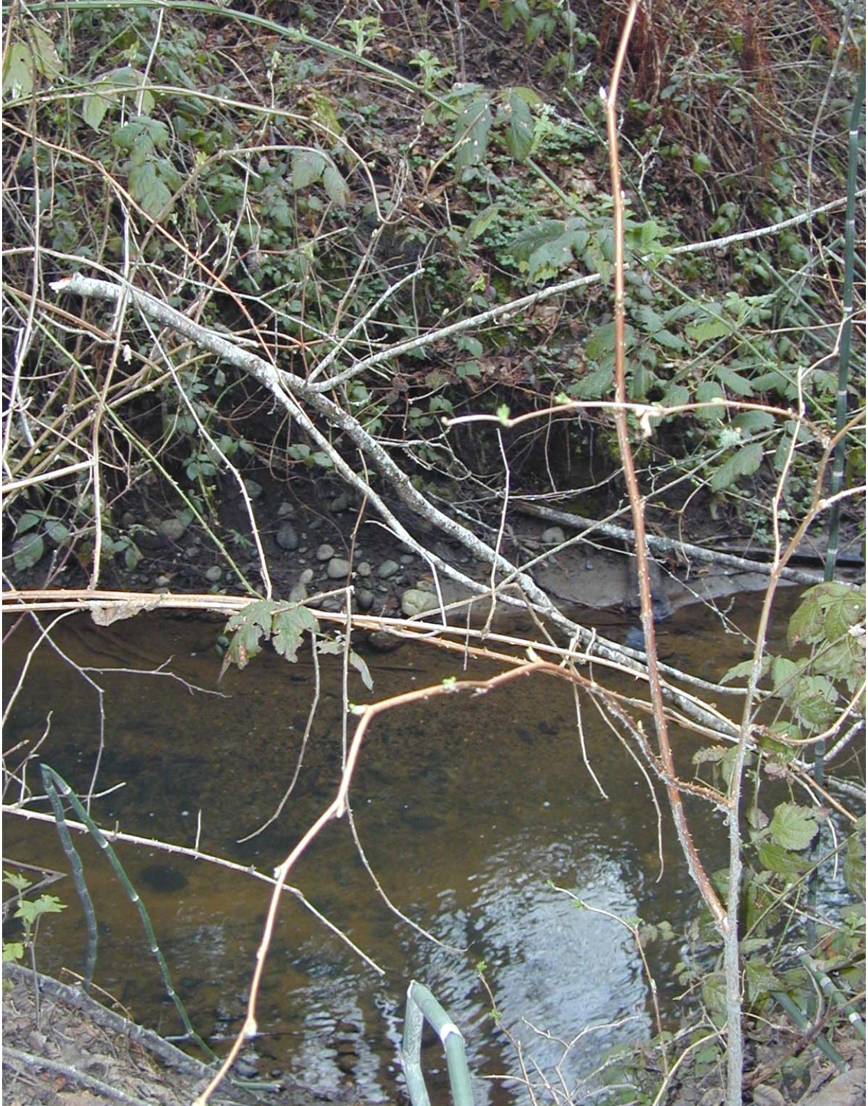
Figure C29. XC19 (left bank) – approximately 3 ft of incision on Warren Creek downstream of AMRR crossing
