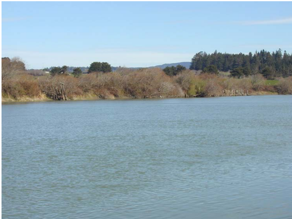
Figure C7. XC4 - Upstream of cross section looking at old protection on right bank
