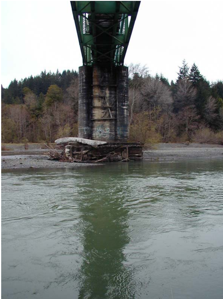
Figure C41. XC21 (right bank) - Looking at degradation near pier
