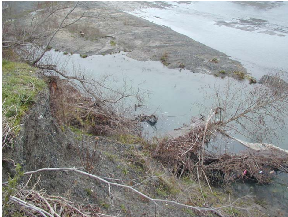
Figure C52. XC24 (right bank) - Erosion on right bank
