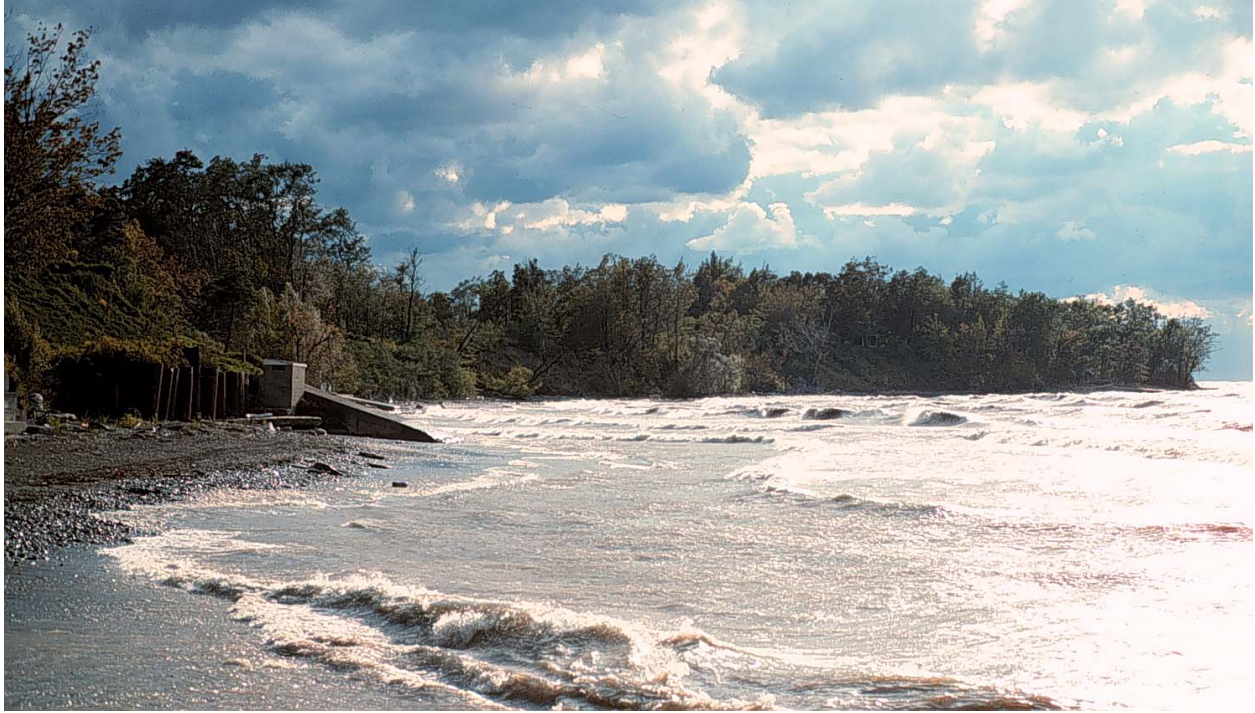
Figure 23. Seawall made of concrete-filled tanks west of North East Marina, November 1991. Most of the ramp and over two thirds of wall are now covered with sand and gravel. In 1991, beyond the walls, there was essentially no beach and waves broke directly at base of bluffs
