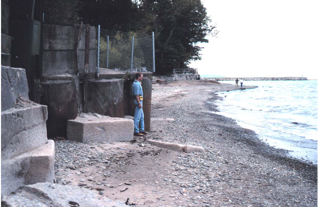
Figure 20. Gravel and sand beach below same structures shown in Figure 19. Beach is about 4 m wide. North East Marina east wall is in distance to right. Photograph taken 11 August 1999, before the autumn bypassing
