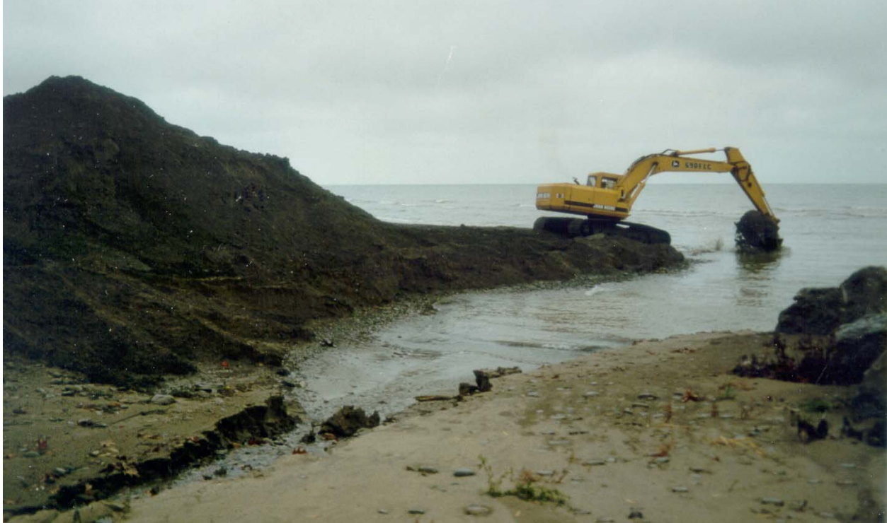
Figure 26. Backhoe removing sand and gravel from updrift fillet, 17 November 1998. A temporary road allows backhoe to proceed out into lake over 30 m
