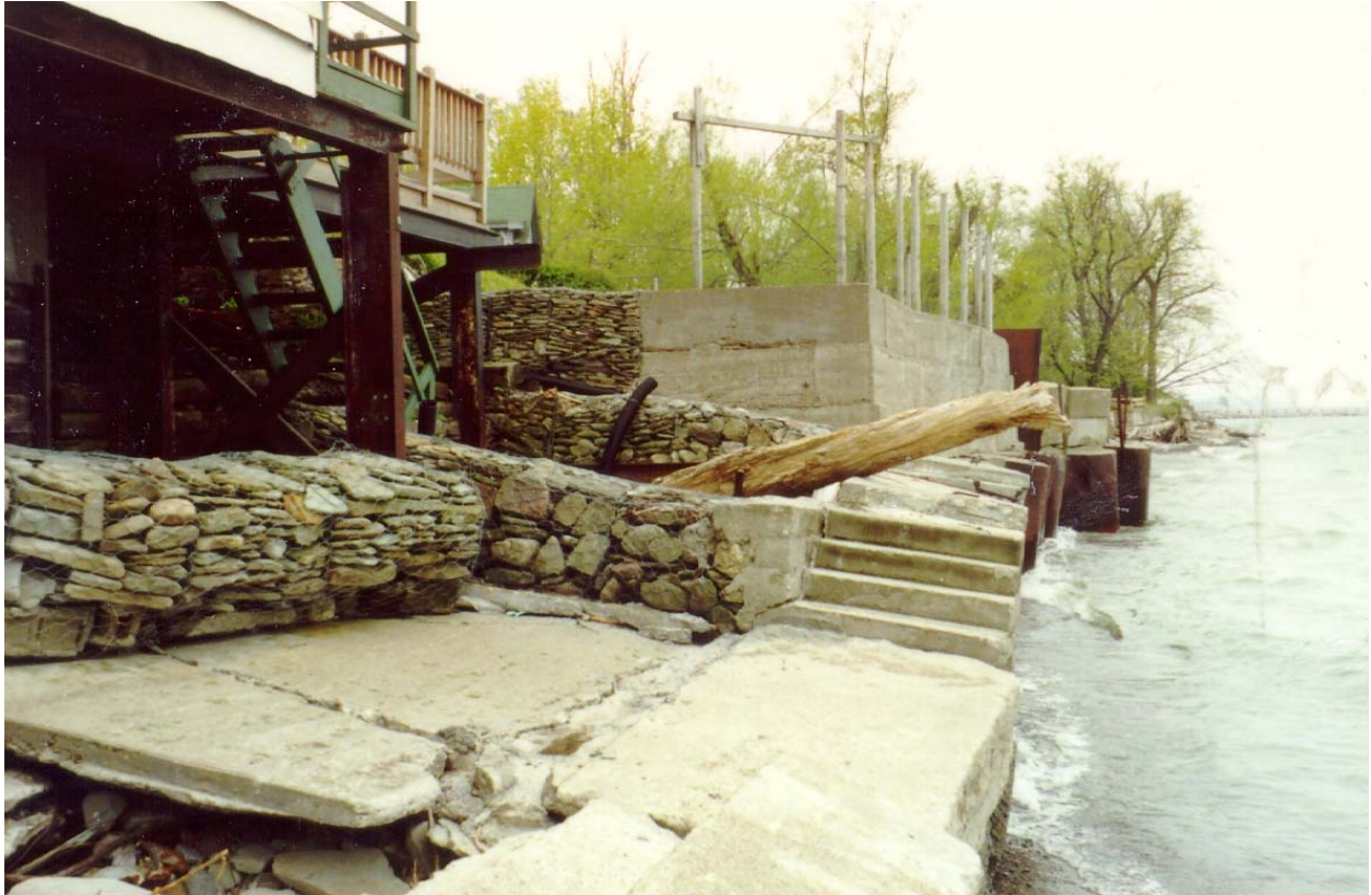
Figure 19. House protected with gabions, concrete, and concrete-filled tanks, May 1991. These structures are about 500 m east of marina's east wall (visible in right side of photograph). Notice tree trunk resting on wall next to steps, evidence of power of storm waves. When this photograph was taken, there was no beach at base of concrete slabs. Photograph from Buffalo District archives
