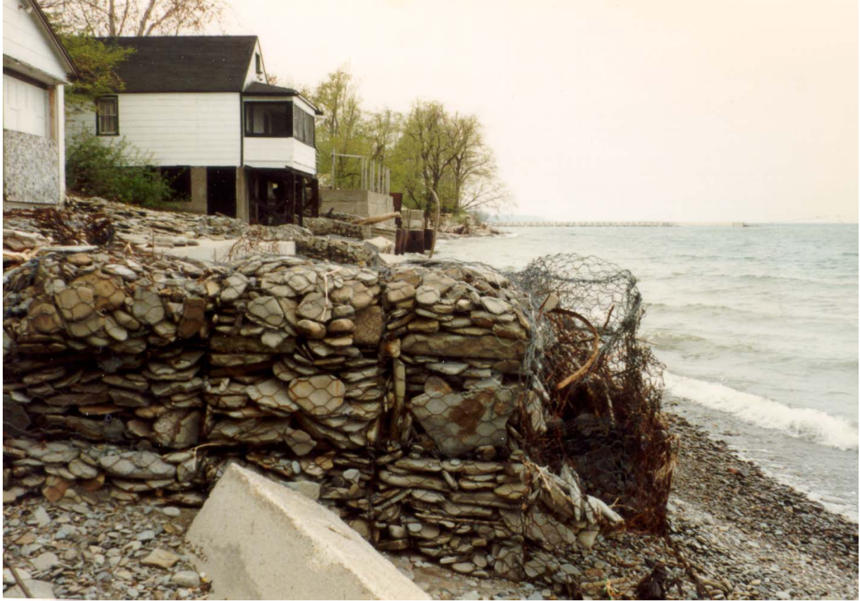
Figure 21. Gabion wall east of property shown in previous photographs, 17 May 1991. Leaning tree where concrete block walls are found is in distance. Photograph from Buffalo District archives
