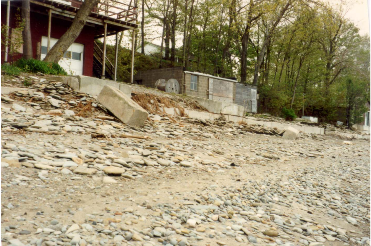
Figure 22. Cottage with protective concrete blocks east of the location shown in previous figures, 17 May 1991. Note the block that has been moved by storm waves. The three properties in the foreground are vulnerable to storm waves because they were built on the beach rather than up on the bluff like the house in the background. Photograph from Buffalo District archives
