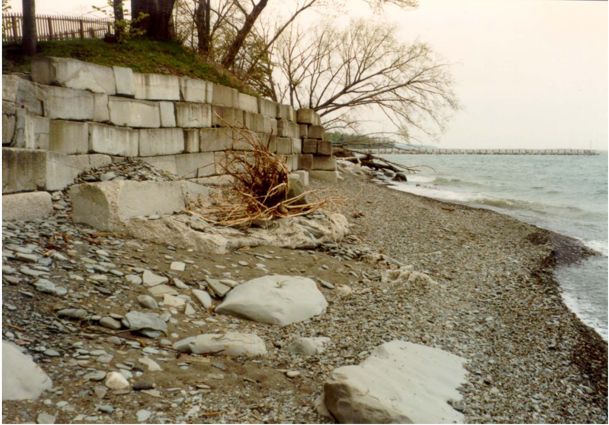
Figure 17. Concrete block wall about 200 m east of marina, 17 May 1991. Leaning tree is seen in subsequent figures
