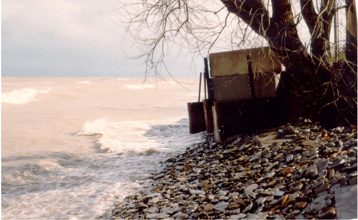
Figure 18. Exposed seawall March 1991, view east. Original photograph label states, "High water from storm just east of Kelley property" (Buffalo District archives)
