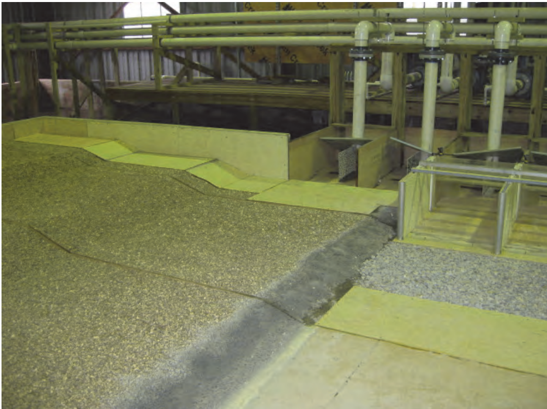
Figure 20. View looking downstream of east bank at two unused pump bays, which are in the location of the sluices.
