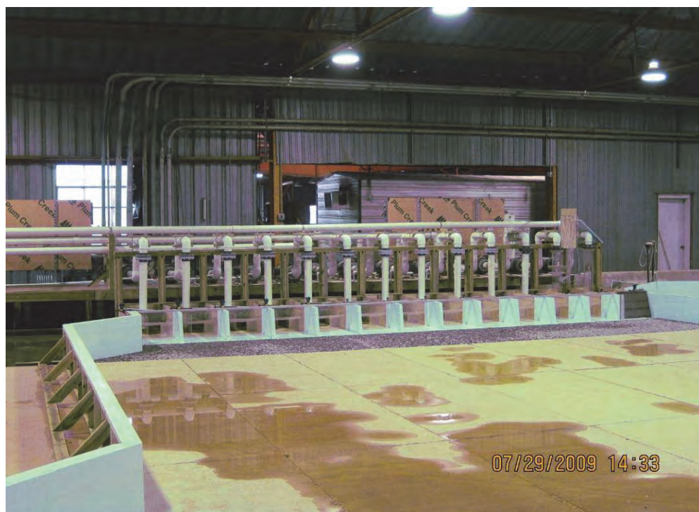
Figure 13. View of original design station with 13 pumps looking downstream.
