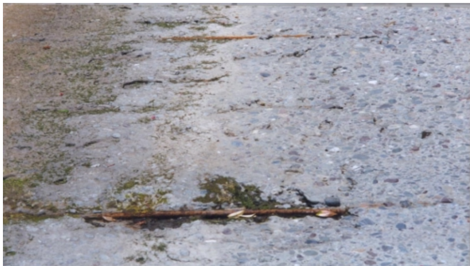
Figure 5. Degraded channel invert
