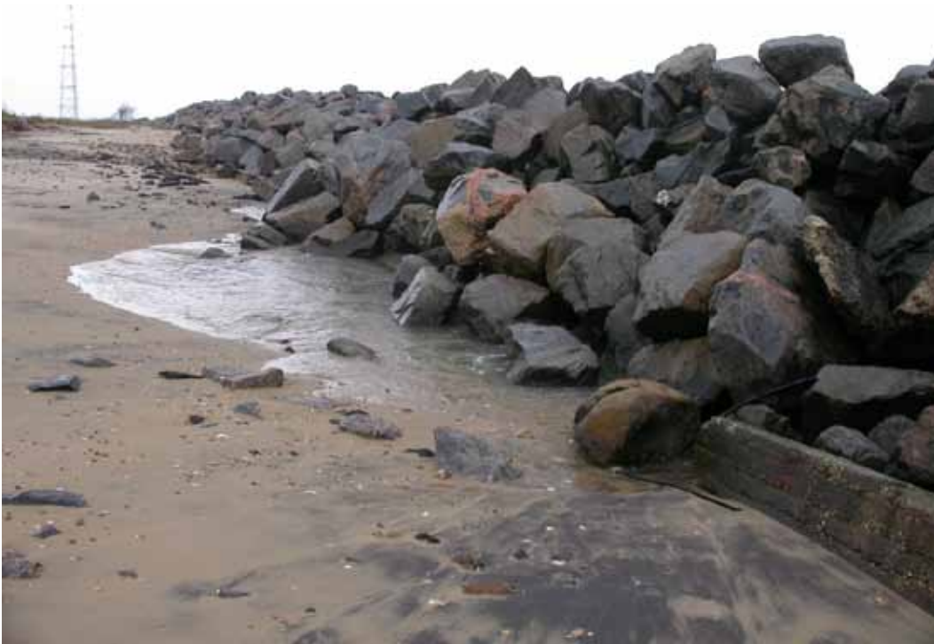
Figure 3-16. Water flowing through seawall by wave action.
