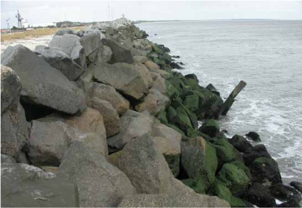
Figure 3-12. Steep seaside face on seawall.
