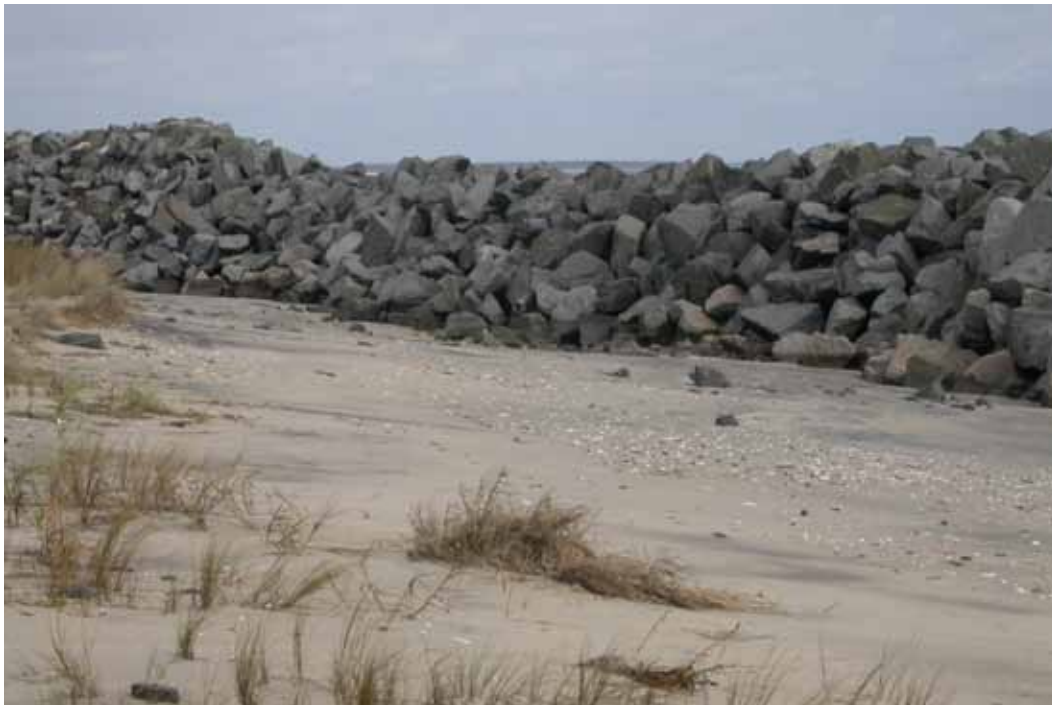
Figure 3-11. Area of decreased crest elevation on seawall.
