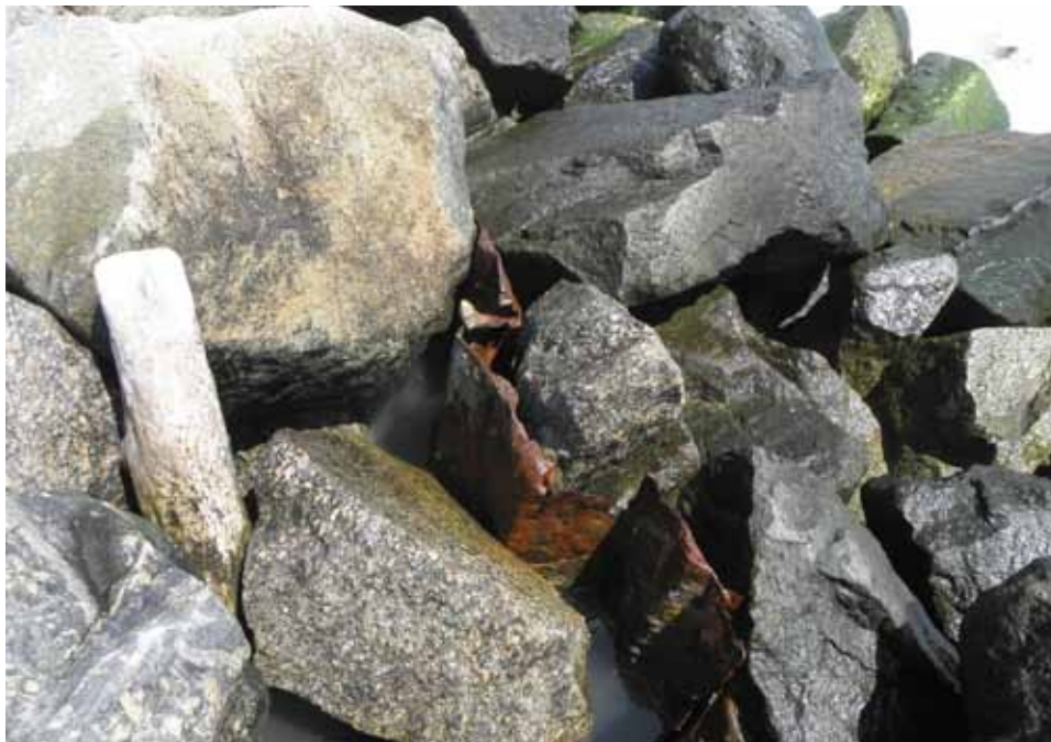
Figure 2-13. Remnants of wooden, steel sheet pile, and concrete seawalls can all be found within and adjacent to the rock seawall in the vicinity of building Y35B.
