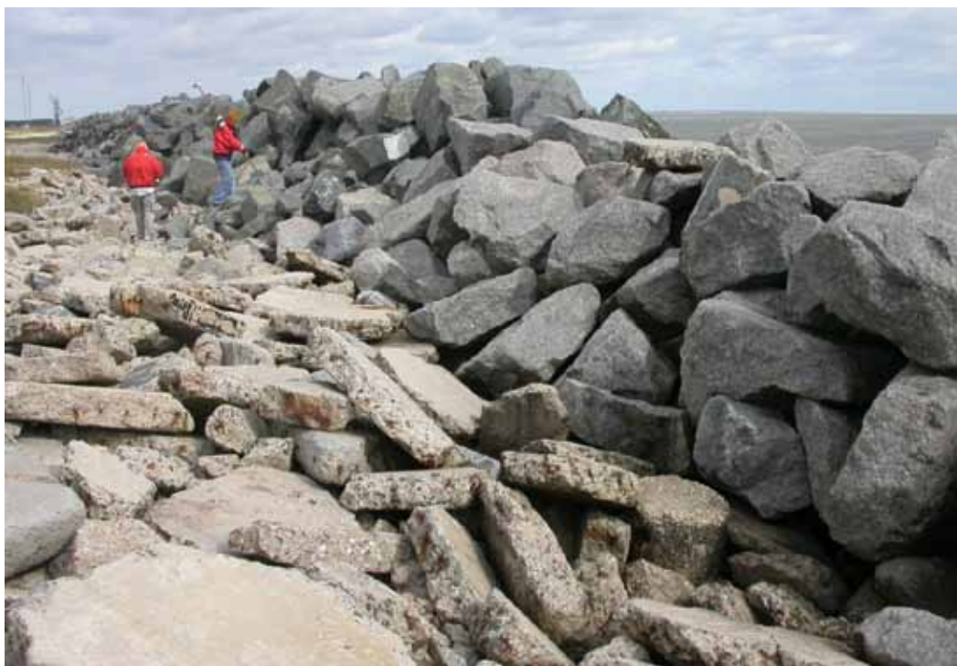
Figure 3-17. Rubble pile behind seawall, presumably to fill scour hole.
