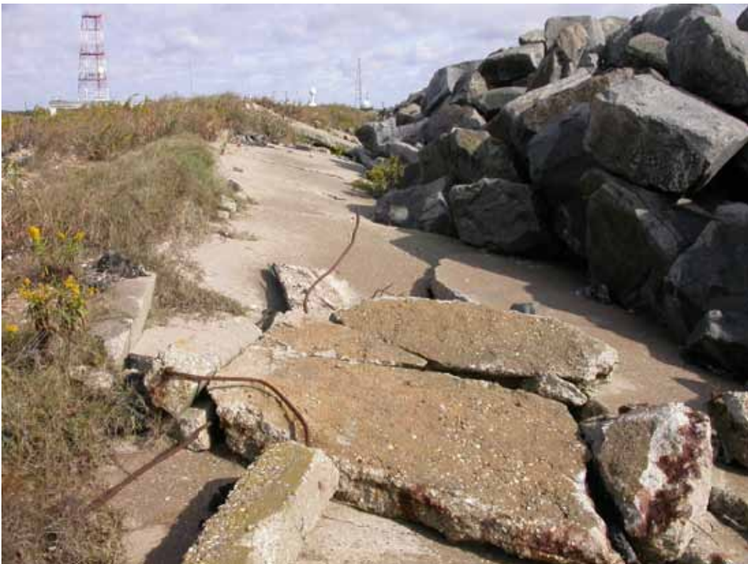
Figure 3-13. Washout under the concrete apron causing cracking and tilting.
