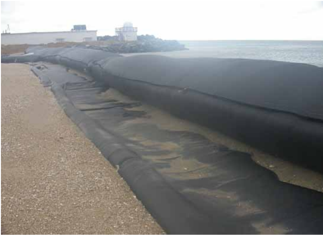
Figure 3-9. Scour apron exposed on landward side of geotextile tube at northern end of structure.
