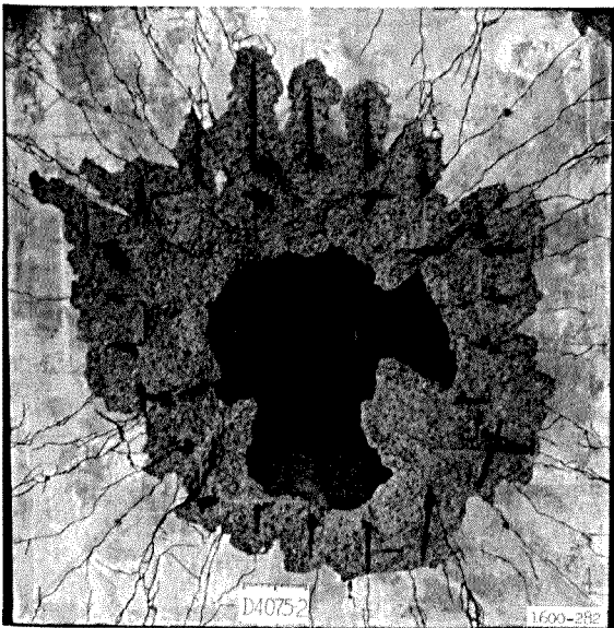
f. Slab with column removed, cracks marked.
