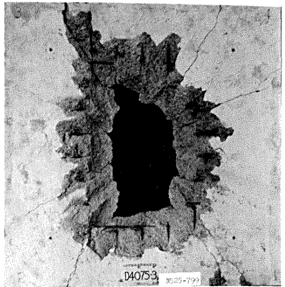
d. Slab with column removed.
