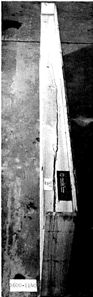
b. Top joist failure (bottom plywood removed).
