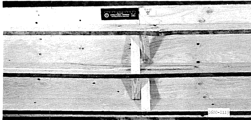
c. Close-up of joist failures
