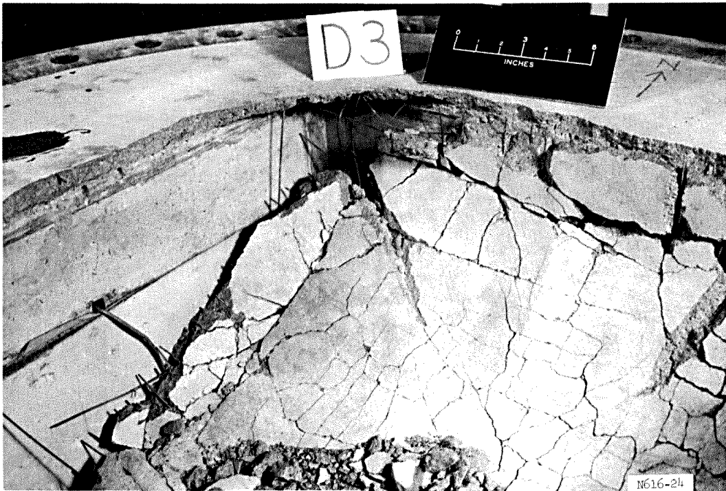
t. Slab ID3, steel rupture.
