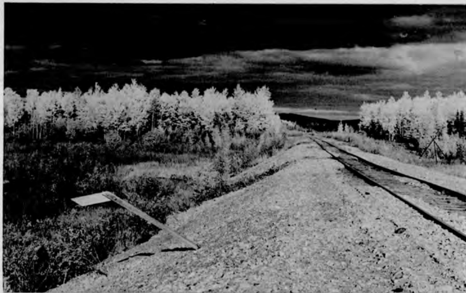
(a) Settlement of a fill near Goldstream
