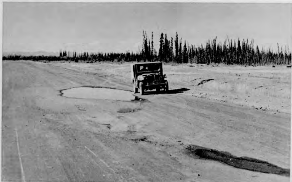
(c) Severe settlement
