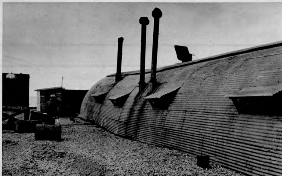
(a) Settlement beneath the stoves
