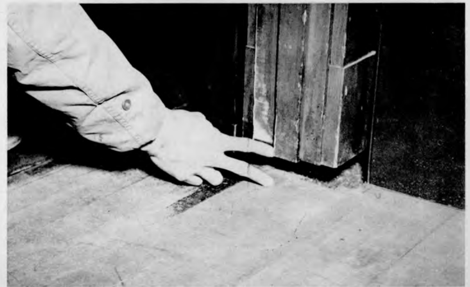
(d) The floor has pulled away from the door jam
