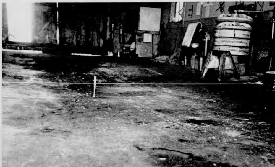
(c) Settlement in a garage
