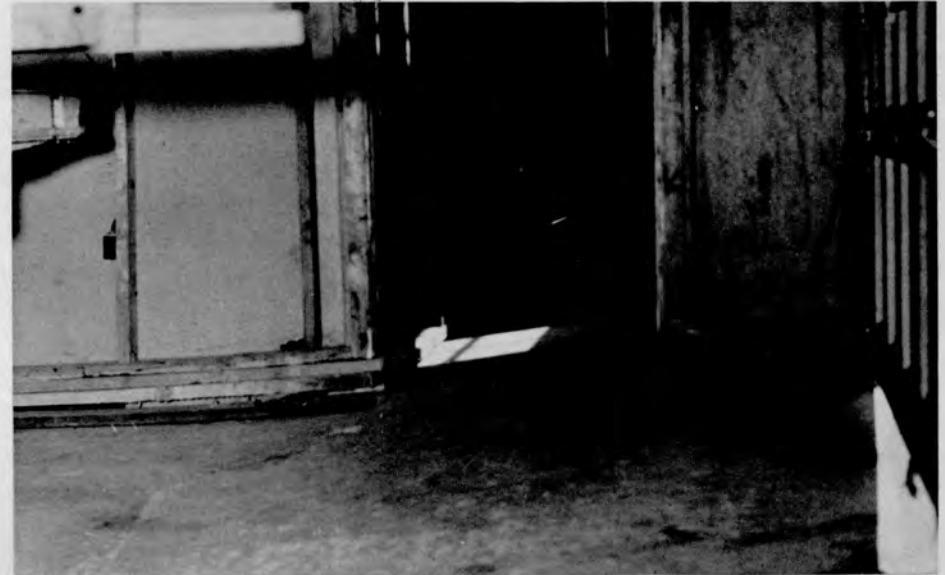
(d) Floor settlement as indicated by the door alignment
