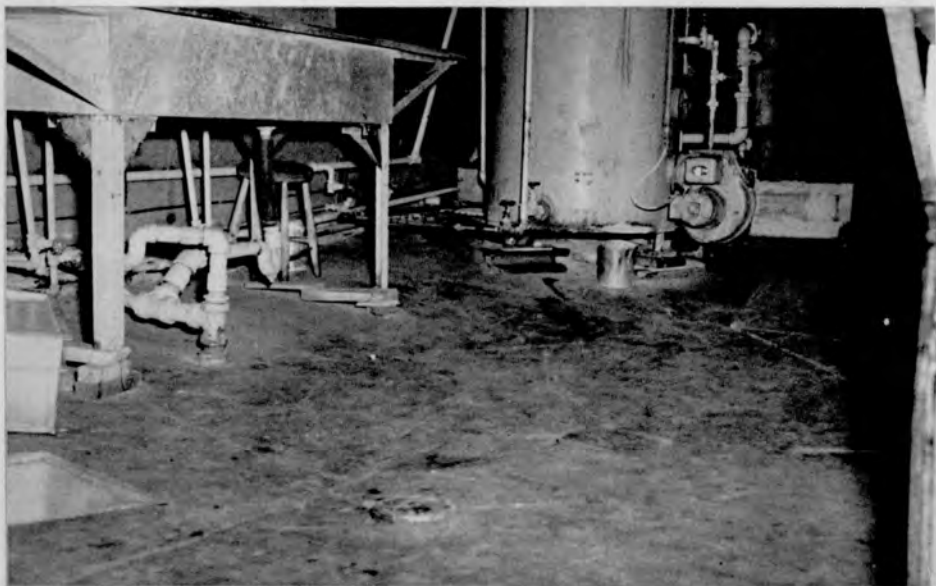
(c) Leaning and propped-up utilities
