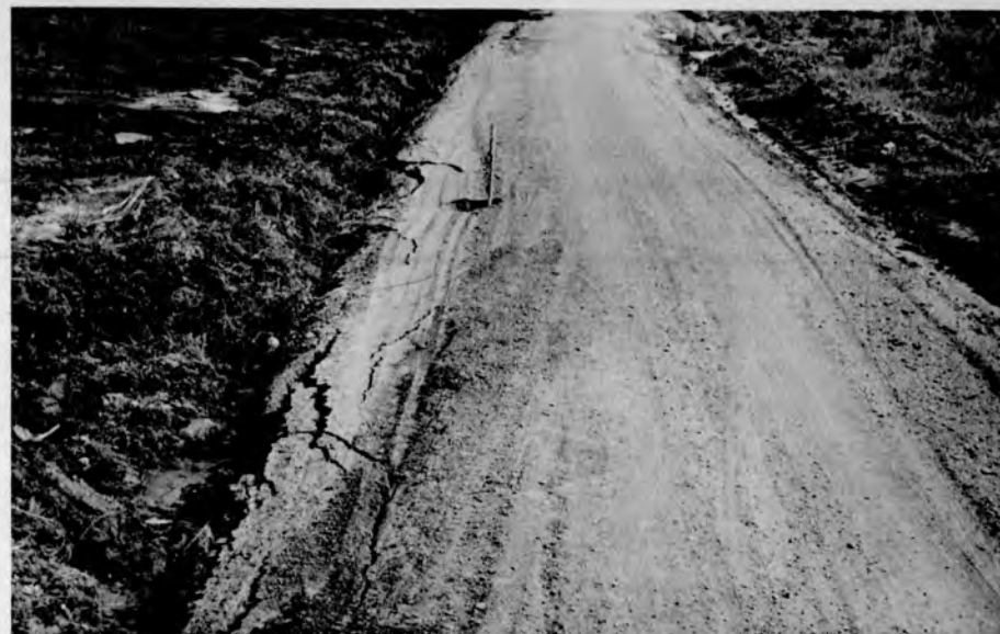
(b) Thaw and poor subgrade support, Steese Highway
