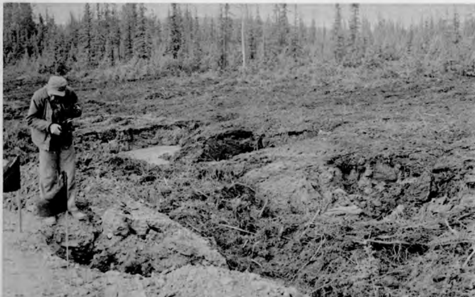
(c) Thaw caused by ditch, Steese Highway
