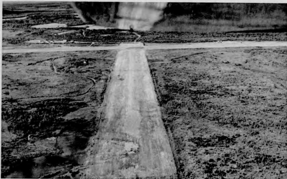
(a) Soft and wet spots in a gravel surface
