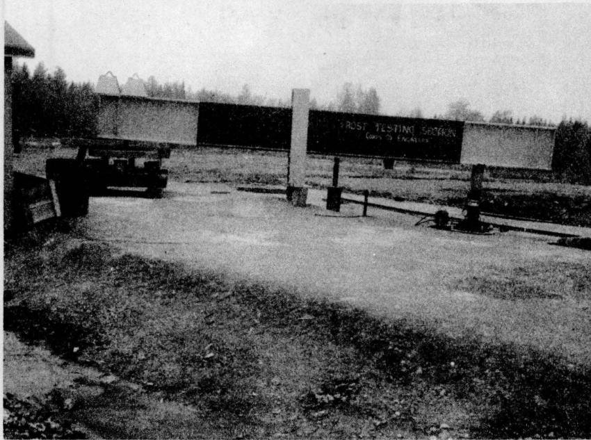
FIG. 1 GENERAL VIEW OF TEST AREA SHOWING REACTION BEAM AND PLATE BEARING TEST SET UP.
