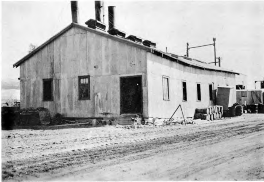
Fig. 57. Settlement of boiler plant at Norman Wells, built on short piles embedded in permafrost. New building being constructed at rear is supported on 30-ft piles that extend to shale bedrock.
