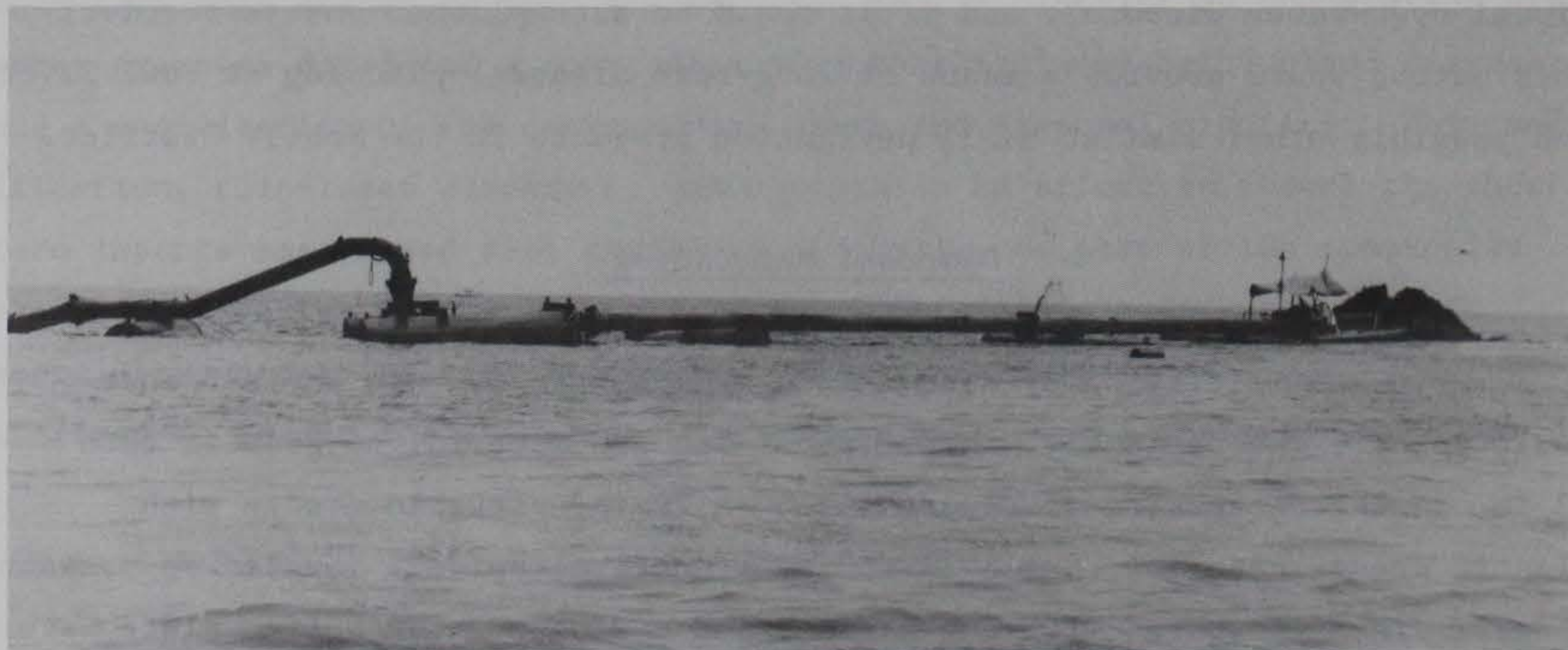
Figure 2. Swivel joint, discharge barge, and baffle spreading device
