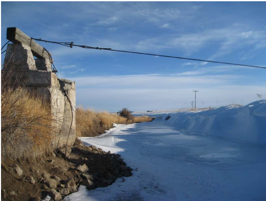
Figure 7. Ice cover in place upstream of 115 th St. Bridge prior to release.
