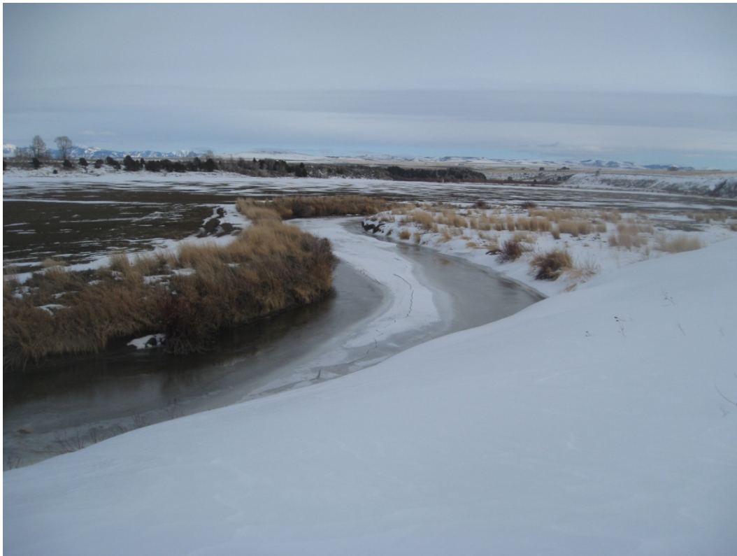
Figure 34. Ice cover upstream of the 115 th St. Bridge after passage of the IRW. Note portions near banks flooded and central longitudinal crack.
