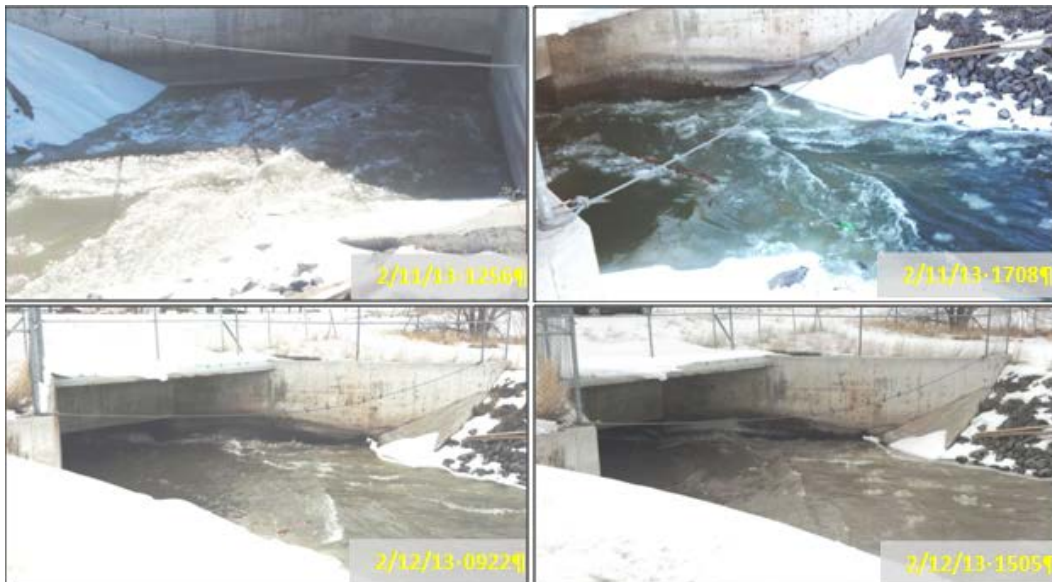
Figure 37. Ice upstream of the siphon.
