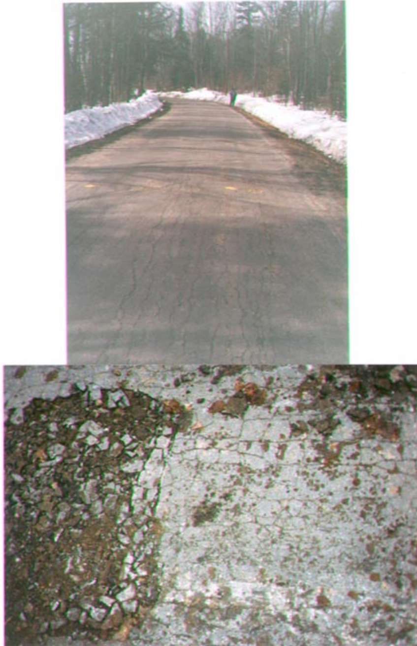
Figure 1. Low volume road with traffic-induced pavement distress during spring thaw.
