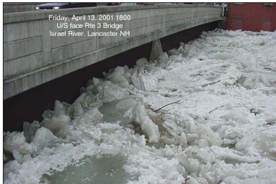
Figure 14. Ice building up on the upstream face of the single-span Main Street Bridge in April 2001. (From USA CRREL Ice Jam Database.)
