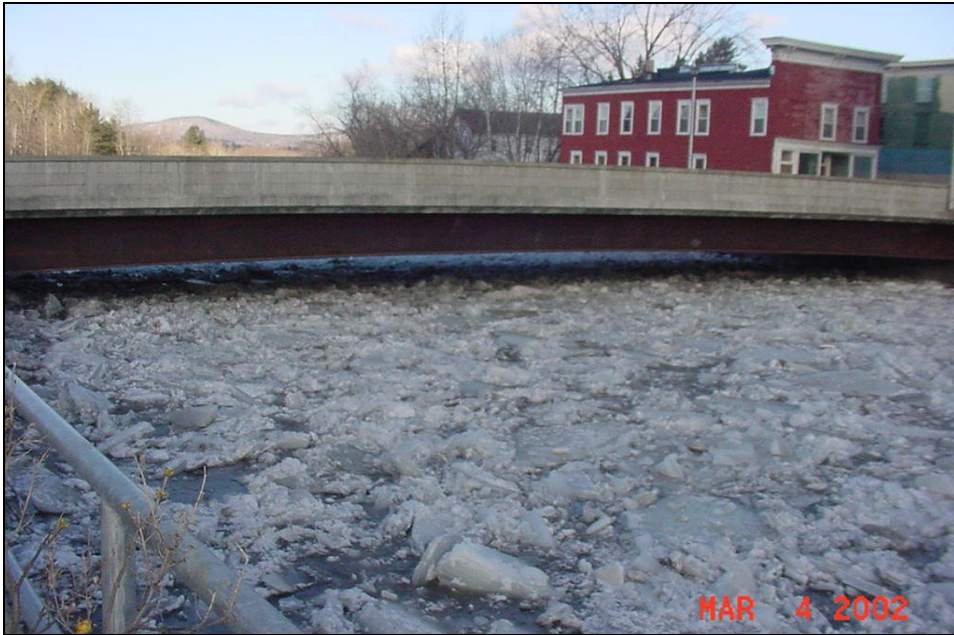
Figure 11. Ice jam of 4 March 2002 (looking downstream toward the Main Street Bridge).
