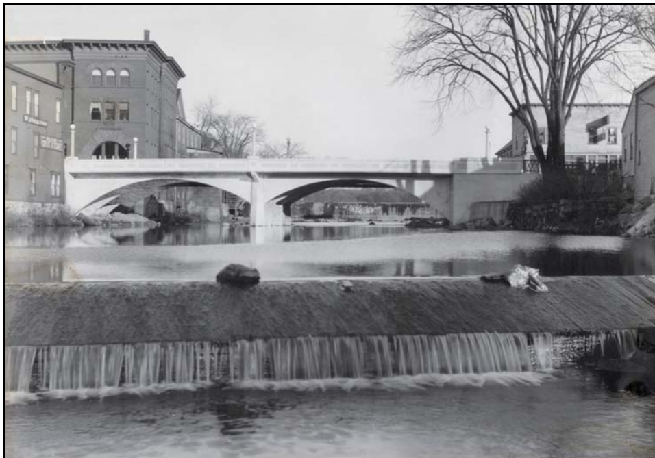
Figure 12. Double-arch Main St. Bridge circa 1928, replaced in 1989-90. Dams #131.01 and 131.02 are visible in the foreground and background, respectively. (Photo courtesy Town of Lancaster.)
