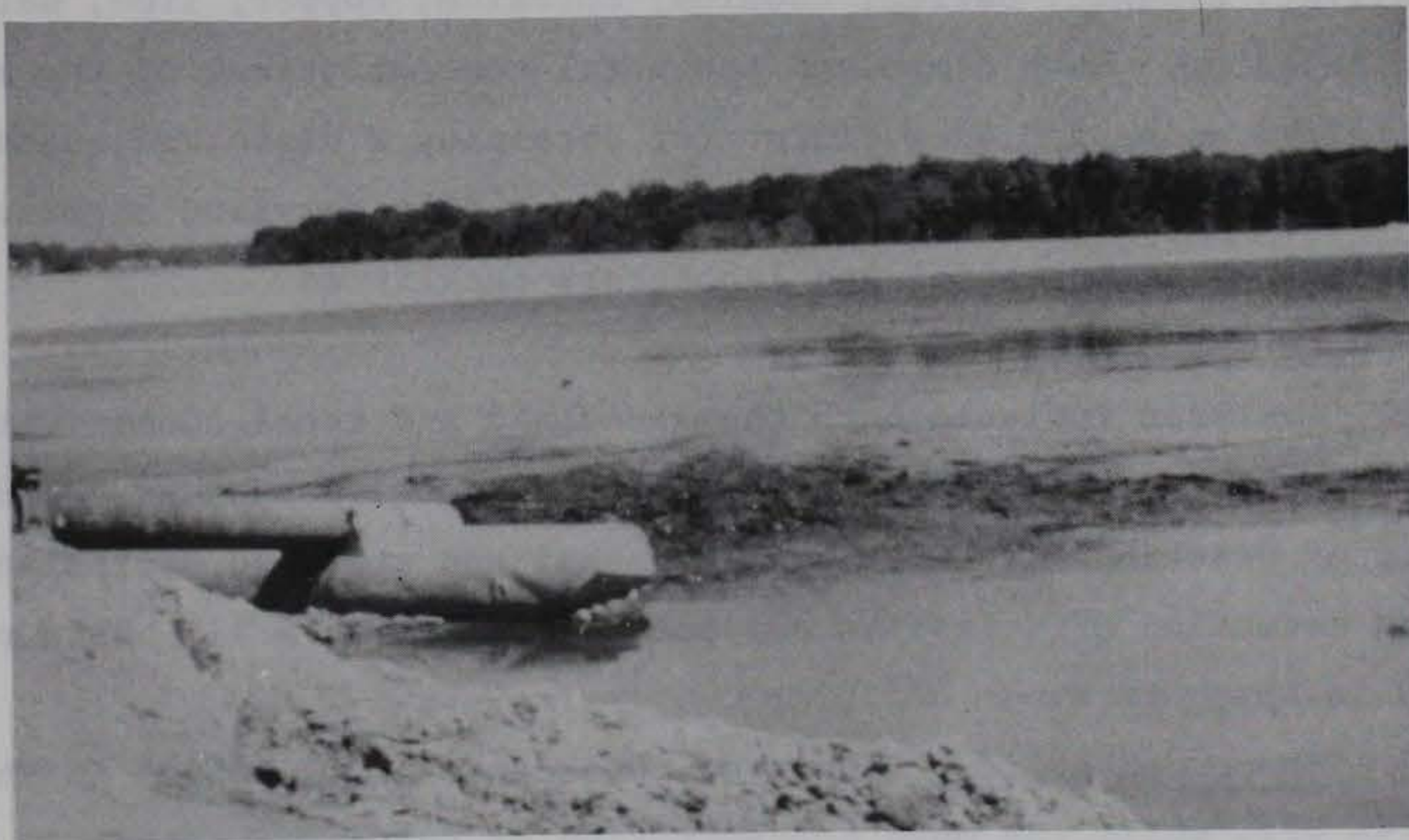
Figure 31. Influent pipe, Hart Miller Island field evaluation
