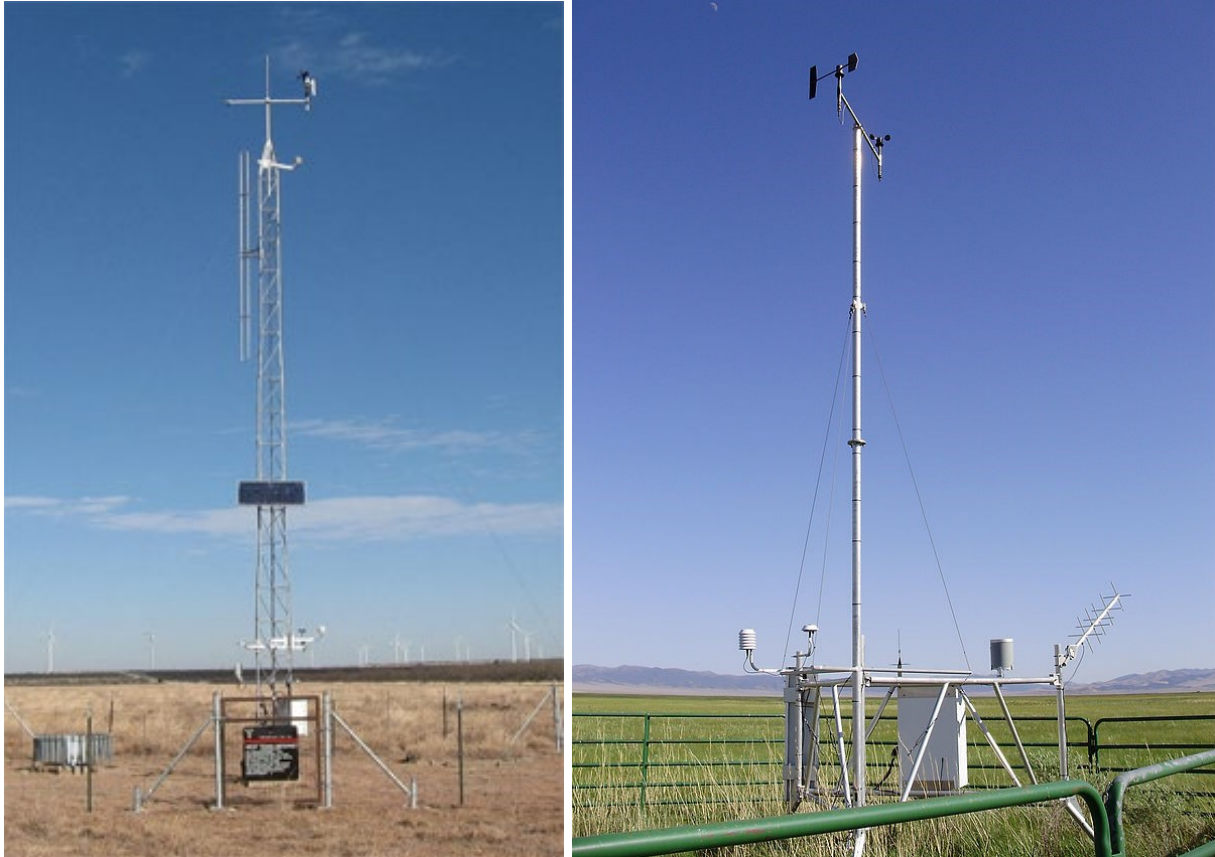
Figure 3. Left photograph: truss-style tower; right photograph: quick-deploy tripod tower, also note the fencing around this tower is the desired corral panel fencing. Photos courtesy of Nathan Edwards, SDSU.
