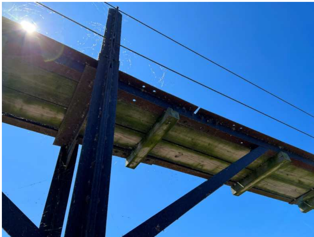
Photo 9 – Decking and Associated Connections to Structure Could Not Be Observed Due to Limited Access
