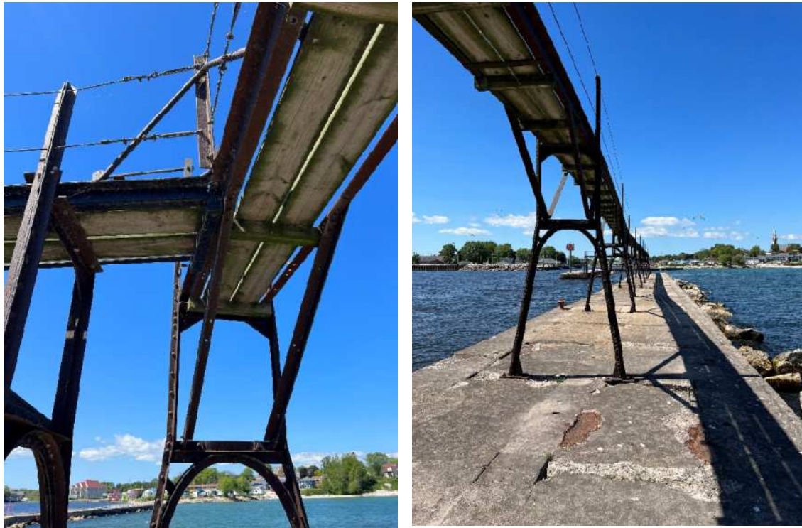
Photo 7/8 – Advanced Corrosion of Members Consistent Along Structure Length
