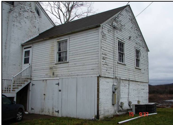
Figure 8. Addition looking northwest, showing juncture with original building and use of stone blocks salvaged from demolished outbuildings. (author)
