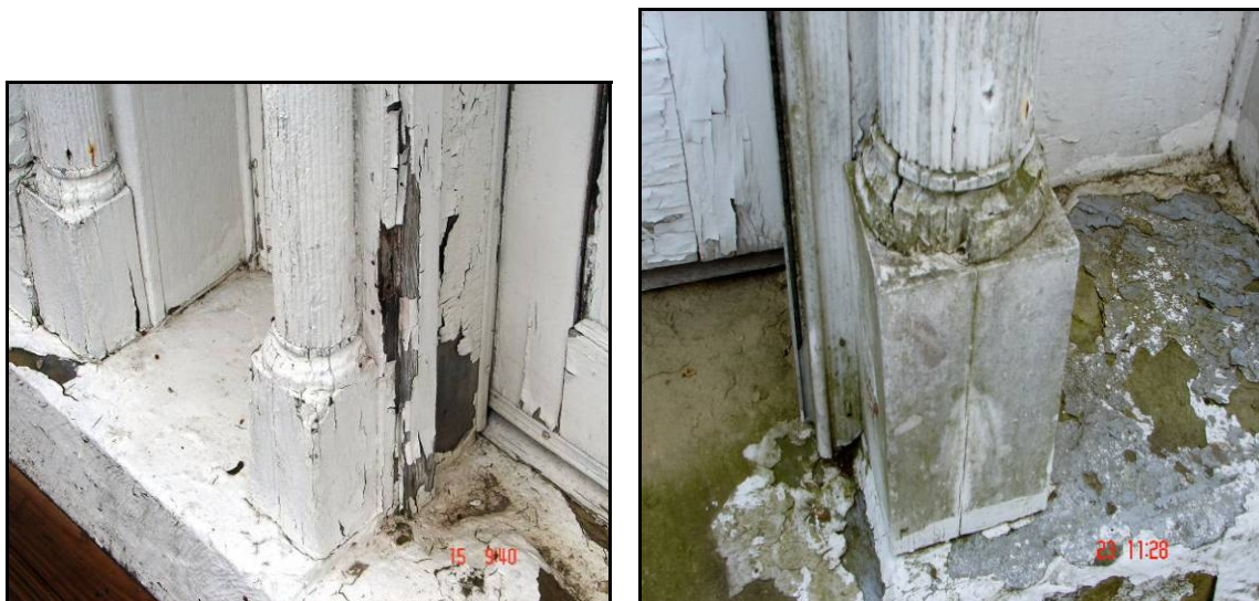
Figure 14. Deteriorated front and rear entrance details such as these pilasters should be documented to guide the authentic replacement of these features. (author)
