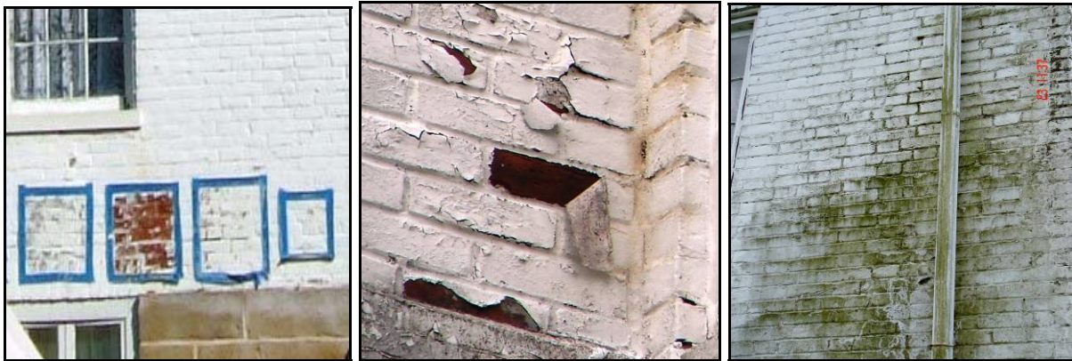
Figure 5. Masonry analysis conducted in August 2007 identified problems associated with painted brick, and involved several test patches to determine the most successful paint removal solution (left, center), and also noted mortar damage from water erosion and leaking downspouts. A suggested mortar formulation for re-pointing is included, with recommendations for preparation and application. (author)
