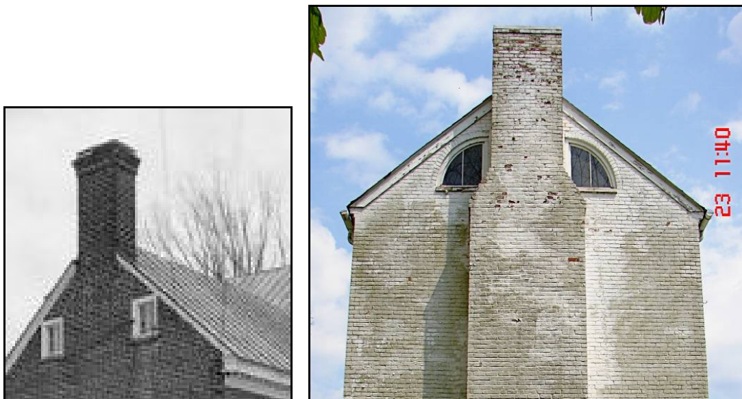
Figure 6. An end chimney on Green Hill Plantation House, Virginia terminates in a typical Federal style corbelled cap (left). Similar capping reconstruction is recommended for both chimneys on the Jenkins House (right) in order to deflect water away from brick surfaces below.
