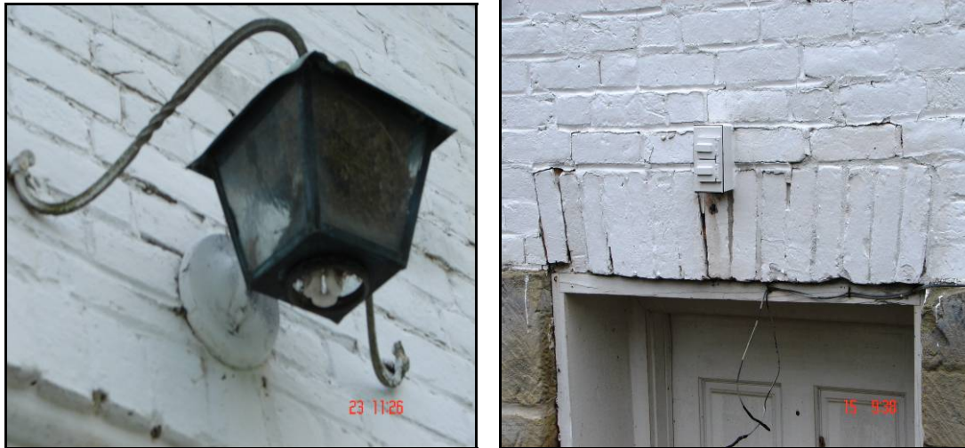
Figure 15. The front entrance light fixture and rear basement door outlet should be removed to prevent water migration through openings, and oxidation staining and mortar deterioration. (author)
