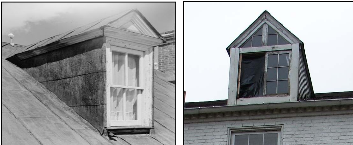
Figure 2. Side by side comparison of a typical Federal style dormer (Green Hill Plantation, Virginia) and a Jenkins house dormer, right. The Jenkins dormer has uncharacteristically crude framing and pediment glazing, and the gable lacks strong classical moldings expected of Federal style buildings. Poor construction allows a number of cracks and openings where water penetrates.
