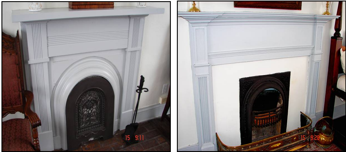
Figure 11. The first floor, east fireplace surround (left) was salvaged from a local property and installed in the 1990s. 8 However, because it lacks the delicate classical proportions of the home's other Federal fireplaces (right), the unit should be replaced, based upon drawings prepared for original surrounds. (author)
