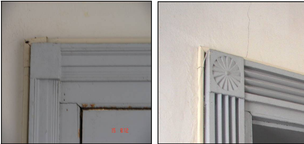
Figure 13. The anachronistic door framing detail (left) suggests that some first floor moldings have been replaced; while others (right) survived as representative of original design. Such original moldings and framing details should be captured in measured drawings. (author)
