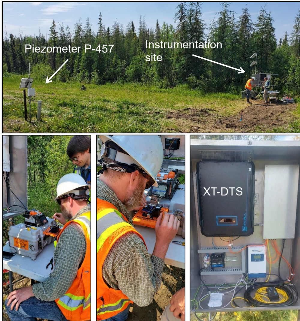
Figure 13. Distributed temperature sensing (DTS) monitoring site and installation.
