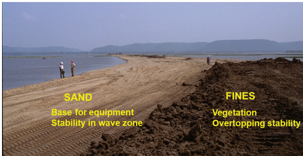
Figure 5. Example of island design with sand base and soft sediment (i.e., fines) to provide substrate for vegetation and stability during overtopping.
