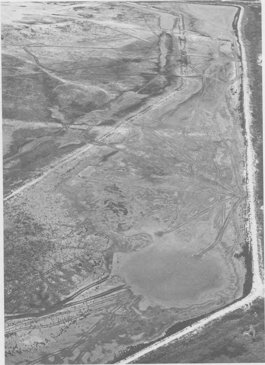
Figure 21. Aerial view of sequential radial trenching procedure used when interior cross dikes are encountered; South Blakeley Island Disposal Site of the Mobile District
