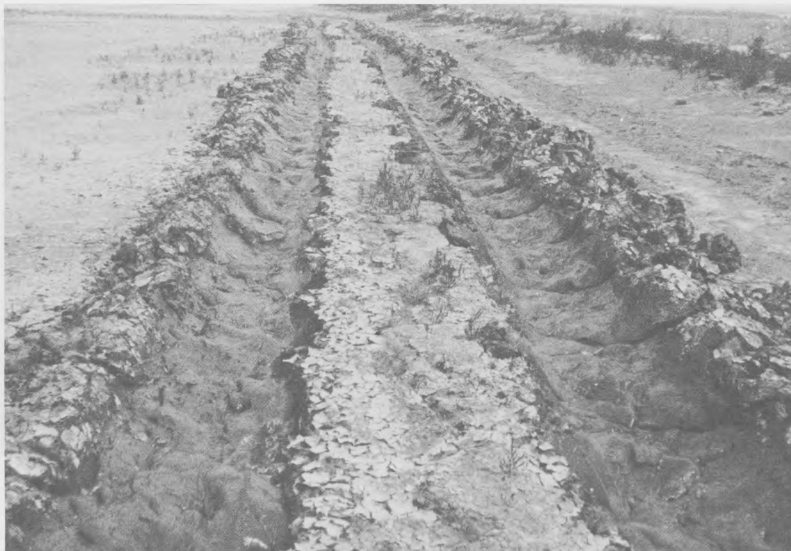
Figure 17. Drainage trenches produced by the RUC when surface desiccation crust is approximately 2 in. thick
