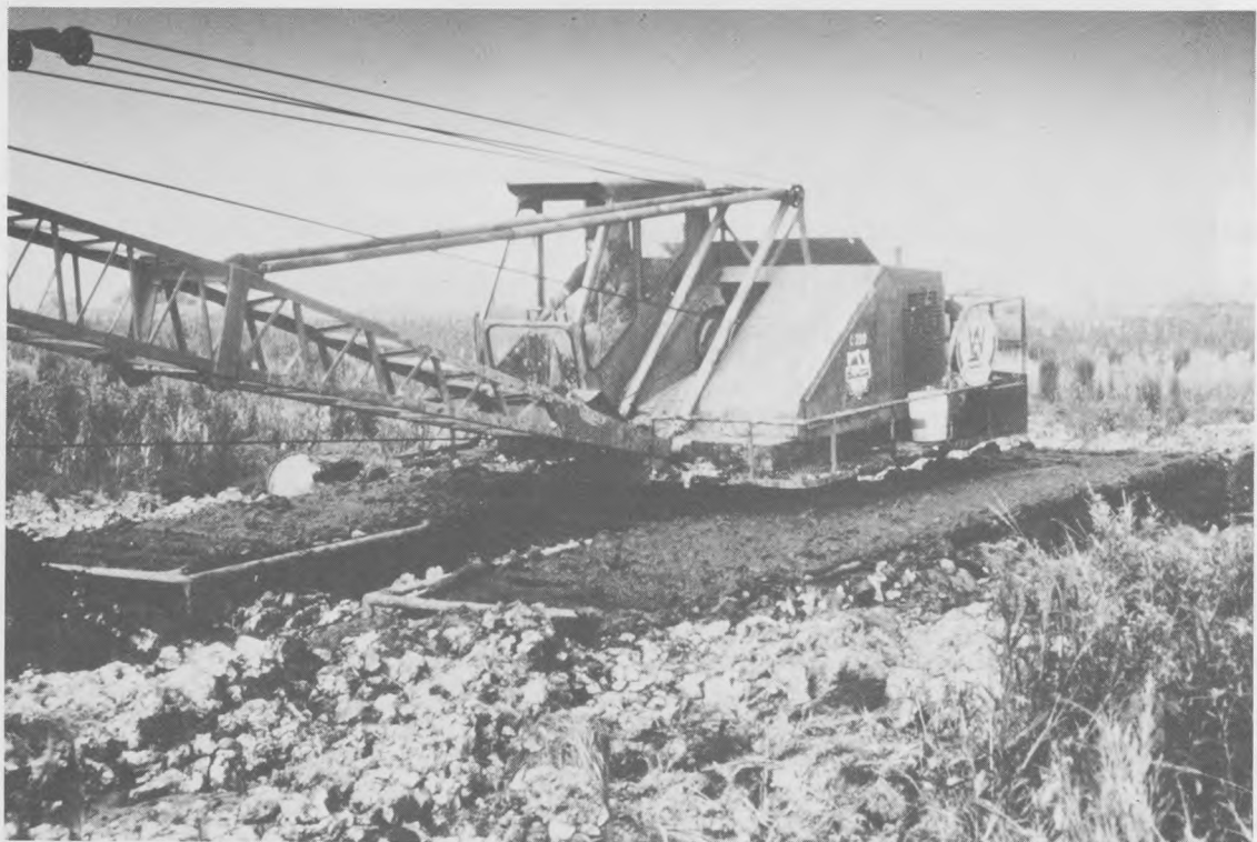
Figure 32. Amphibious low-ground-pressure dragline immobilized after breaking through 4-in. surface desiccation crust
