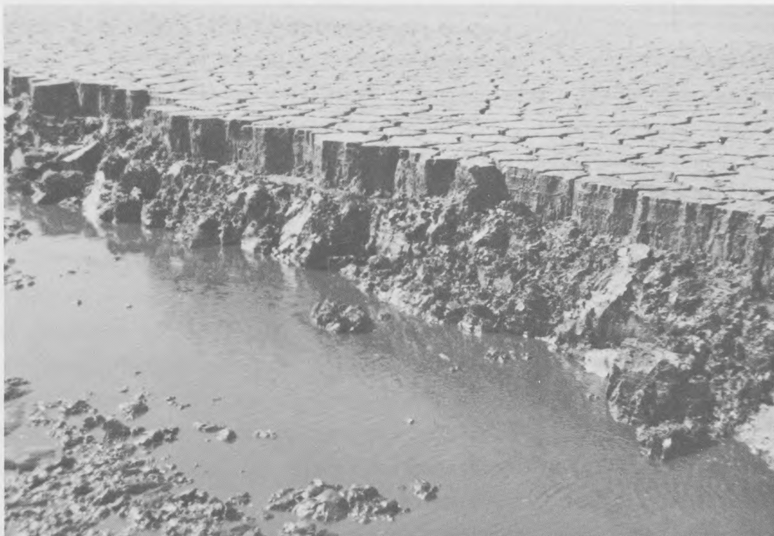
Figure 9. Desiccation crust adjacent to perimeter 3.5-ft-deep drainage trench
