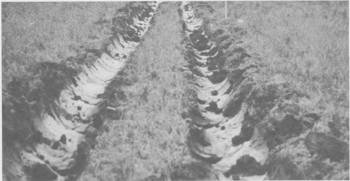
b. Completed and well-formed RUC drainage trench produced on second trenching pass
