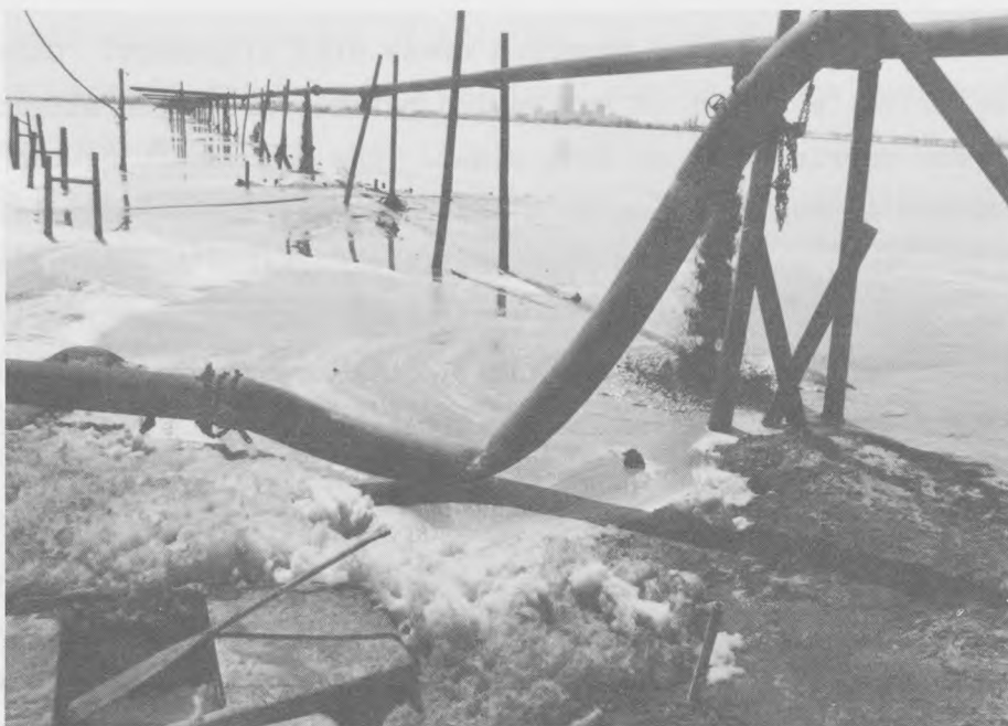
a. Creation of interior cross dike by controlled deposition of coarse-grained material along proposed dike alignment
