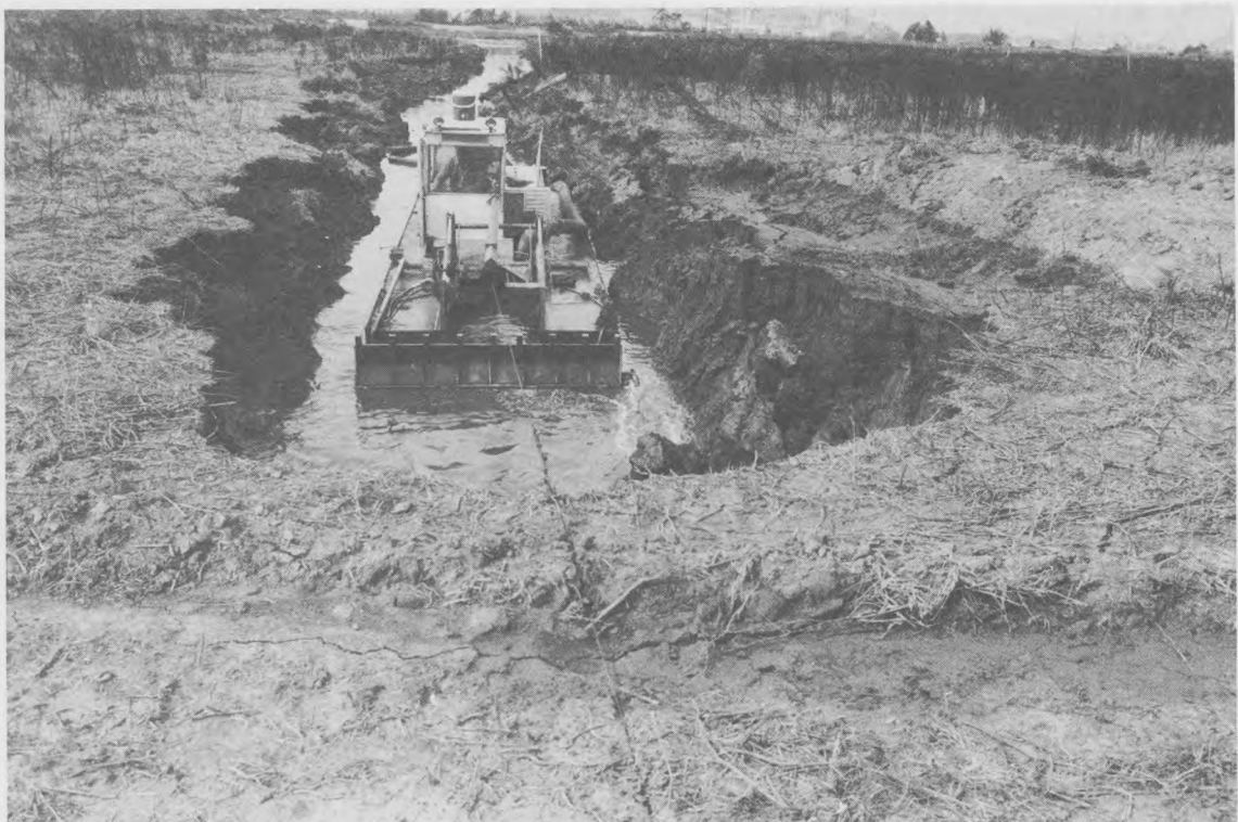
Figure 29. Mudcat dredge trenching operation in progress at disposal site location with approximately 18 in. of surface crust
