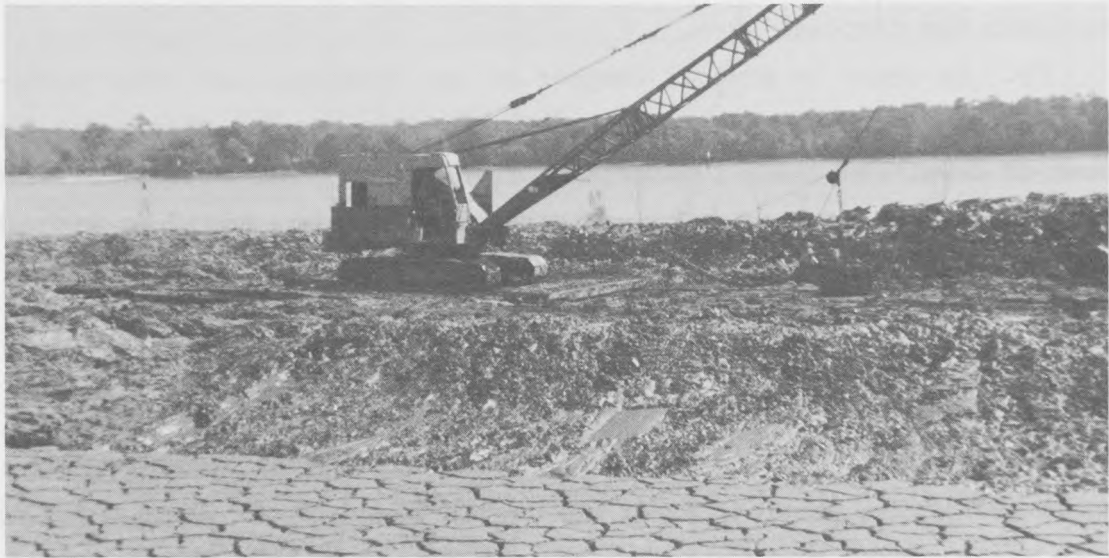
a. Small dragline on mats working on berm deepens shallow perimeter drainage trench
