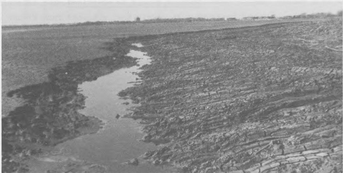
b. Deepened perimeter trench constructed by dragline working on berm Figure 6. Trenching from berm inside perimeter dike
