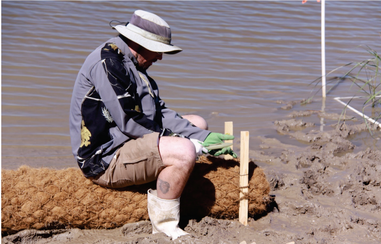
Figure 4. ERDC staff demonstrates the installation techniques for coir during the Engineering With Nature® (EWN®) workshop.
