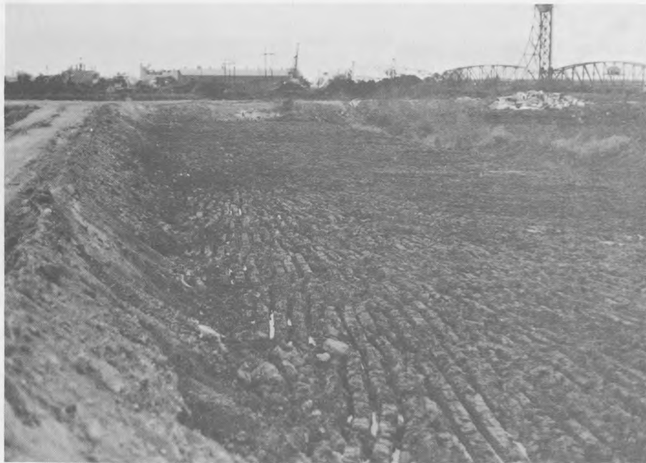
Figure 13. View along edge of spur haul road after dredged material crust had been removed. No evidence of subgrade bulging, foundation bearing failure, or mud waves is seen in the photograph
