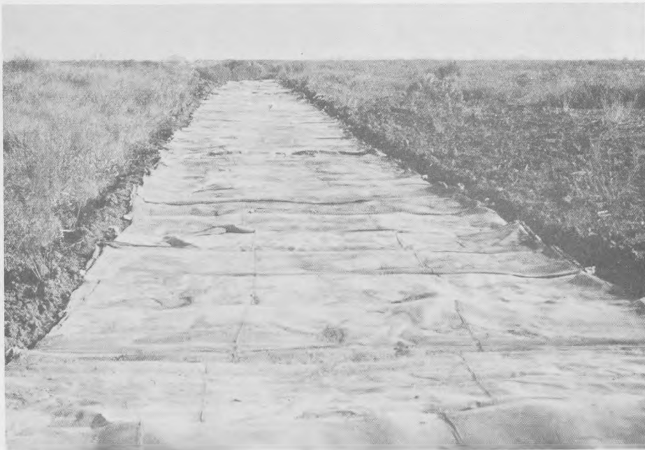
b. After the pad was complete, 12-ft-square sheets of filter fabric were laid on the pad and overlapped
