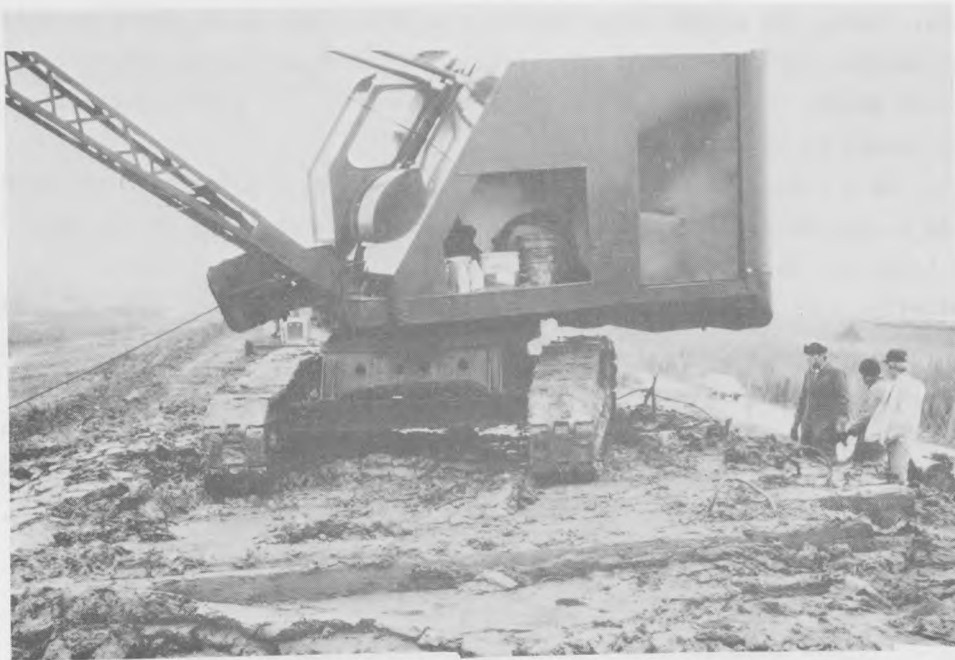
Figure 21. Dragline in mobility trouble on east dike caused from precipitation ponding and infiltration into previously place first lift
