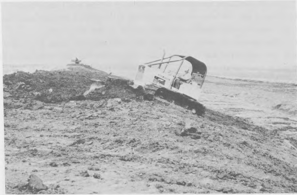
Figure 18. Small wide-track dozer shown constructing first lift while dragline in background of photograph constructs second lift and dresses the crest and side slopes
