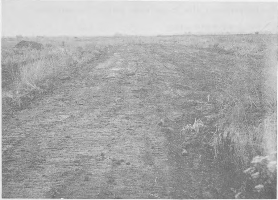
a. Mounded subgrade for interior haul roads was constructed with the small wide-track dozer. Material was bladed from the right of the photograph and semicompacted to form the haul road pad shown in the center of the photograph
