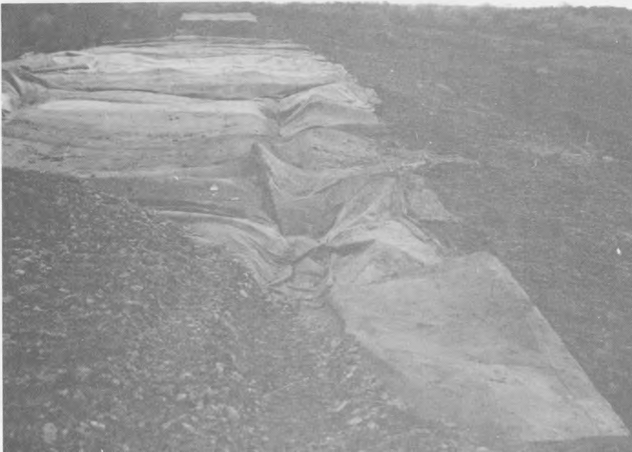
Figure 10. Rutting in the fabric-supported subgrade occurred when trucks backing down the haul road spreading shell continued to back after their load was exhausted. The photograph illustrates the need for fabric cover to obtain desired roadway performance
