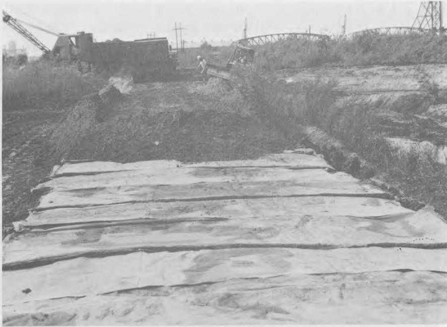
a. Cement waste evaluated as road surfacing is shown being placed on the fabric-covered subgrade. Note the resemblance of the partially hydrated cement waste to sand
