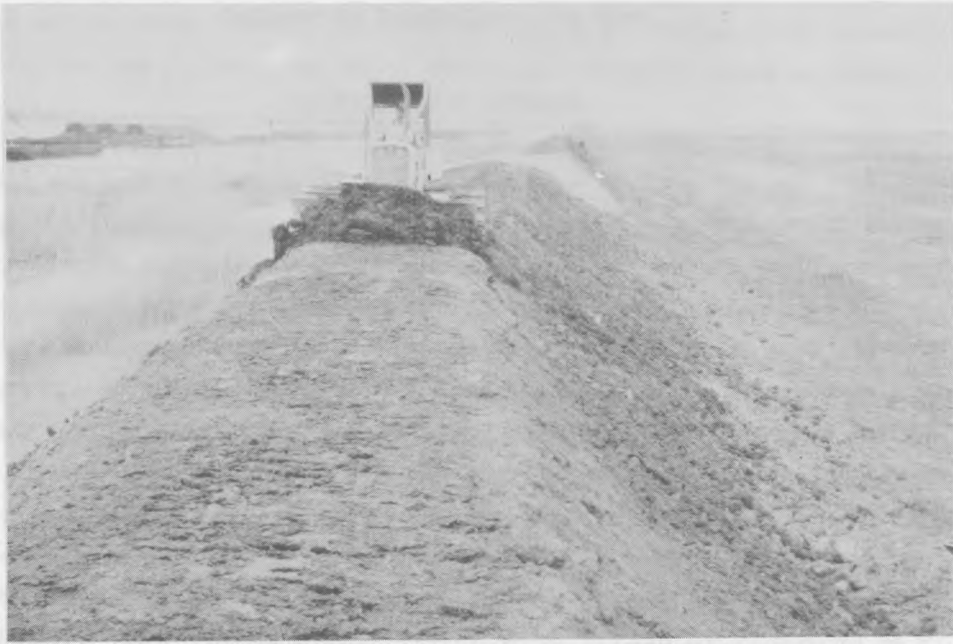
a. As the last construction operation, the small wide-track dozer bladed the dike to 8-ft crest width at El. 24 MSL
