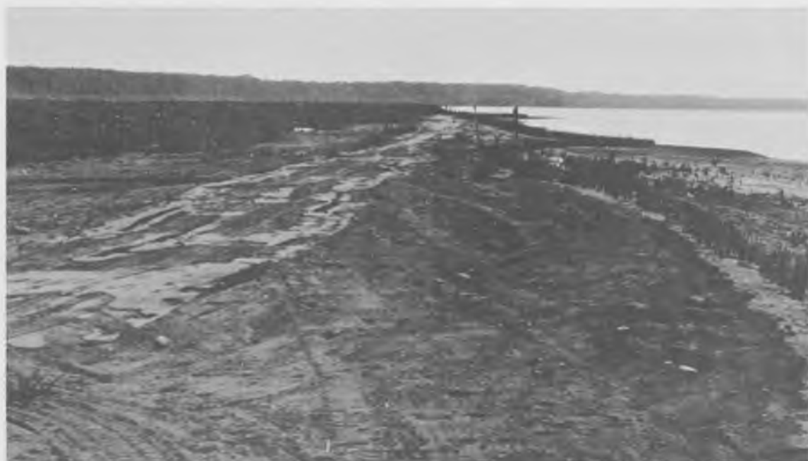
Figure 18. Northeast corner of the dike looking west along the north side on 31 July 1975 just following seeding (after Garbisch 1978).
