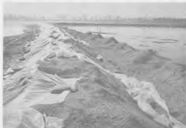
c. DAMAGED POLYETHYLENE SHEETING - WEST DIKE ALIGNMENT 28 JAN 1975
