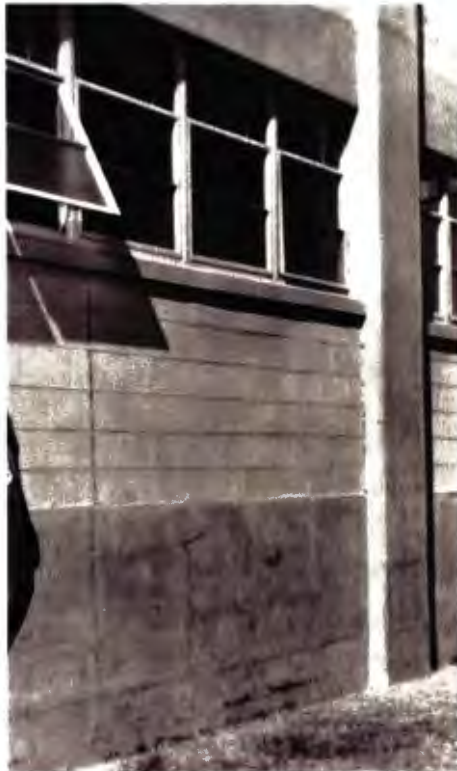
Original unpainted exposed concrete and concrete block with original steel awning windows
