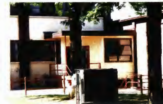
Building 2379 - north entrance between the head and handle portions, with original steel awning window and asbestos siding
