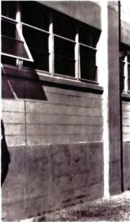
Original unpainted exposed concrete and concrete block with original steel awning windows
