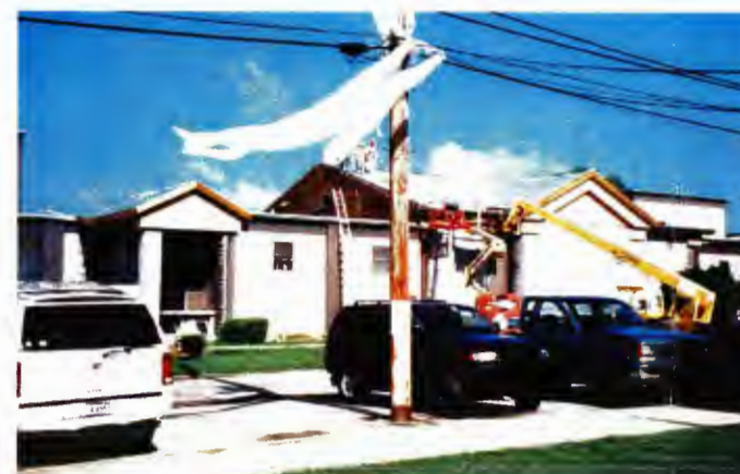
East elevations of Building 6556-right and Building 6557-left with addition in between
