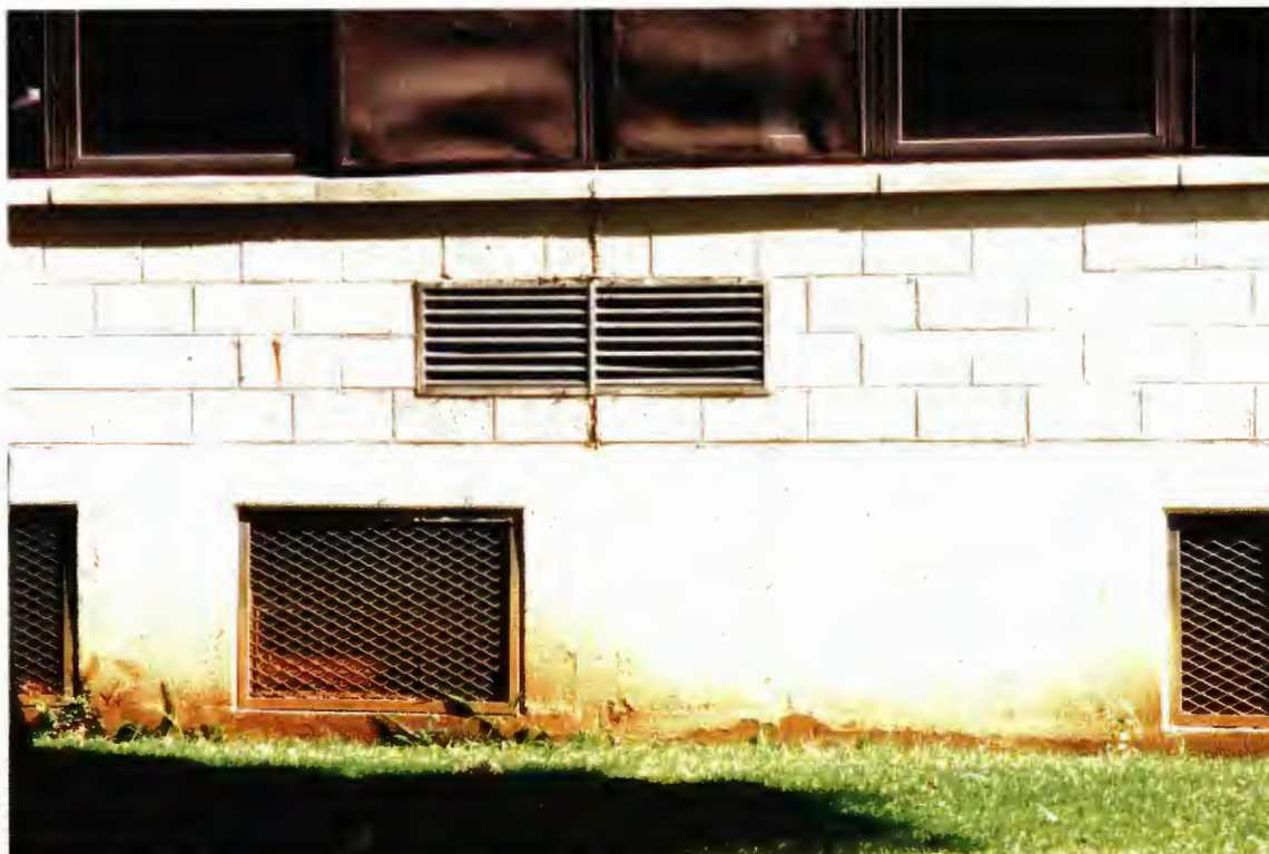
Building 1480 – air conditioning unit installed in the concrete block exterior wall
