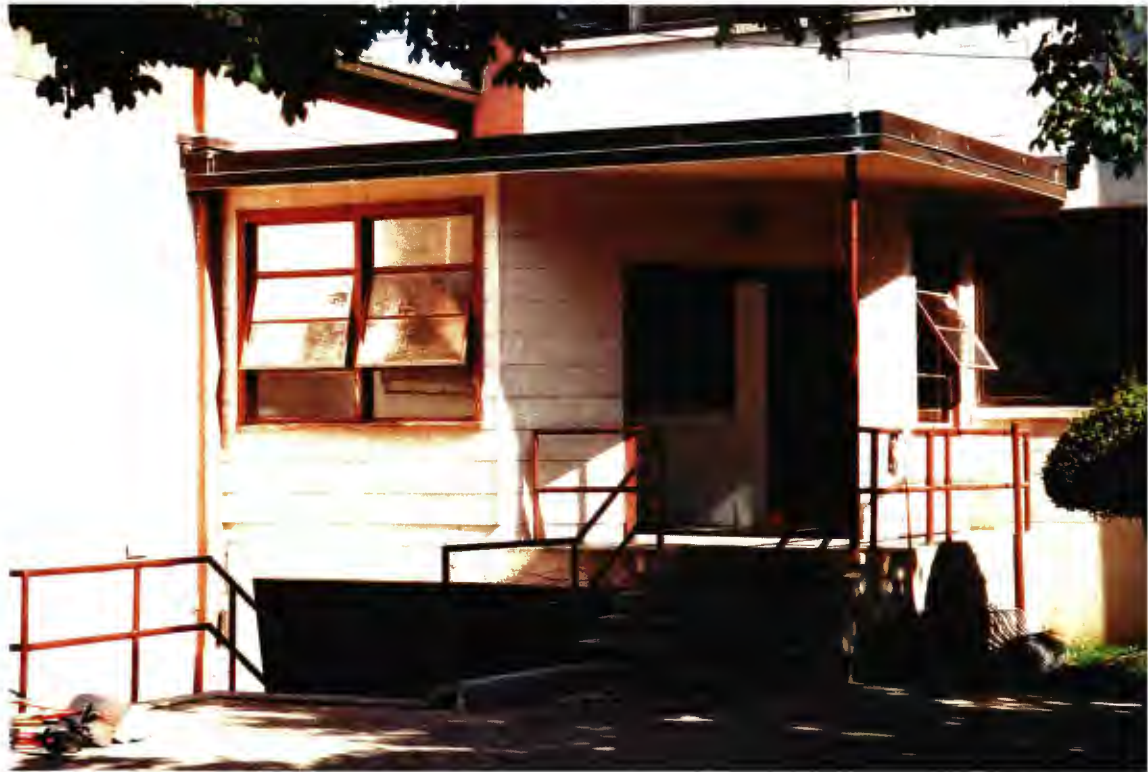
Building 1476 – south entrance between handle and head with asbestos siding and original steel awning windows
