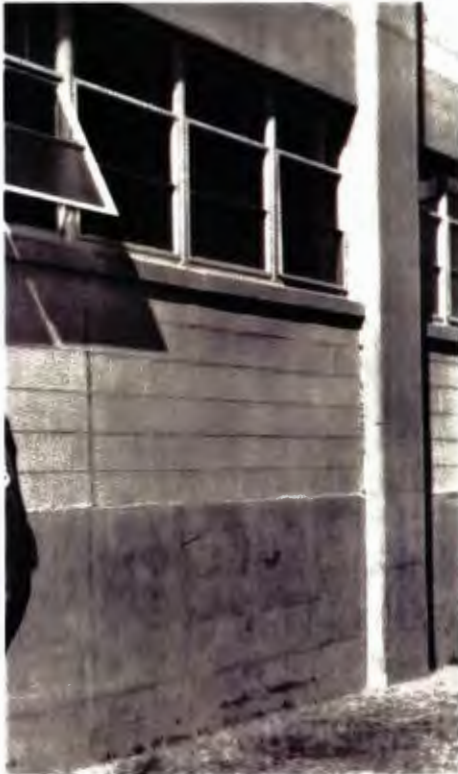
Original unpainted exposed concrete and concrete block with original steel awning windows
