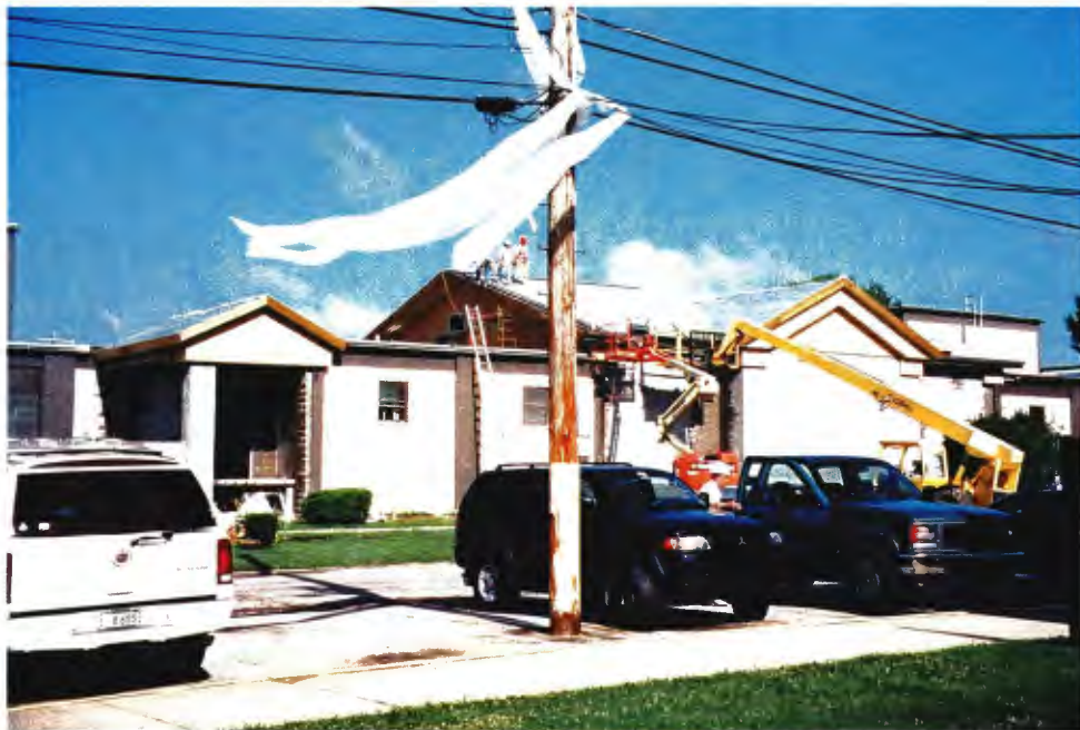
Figure 39: In 2004, new additions were constructed between the head and tail portion of a few hammerhead barracks, altering the exterior appearance of the barracks (ERDC-CERL).
