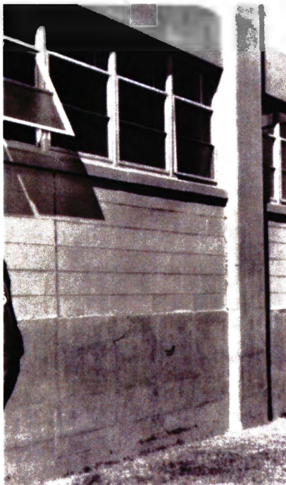
Original unpainted exposed concrete and concrete block with original steel awning windows
