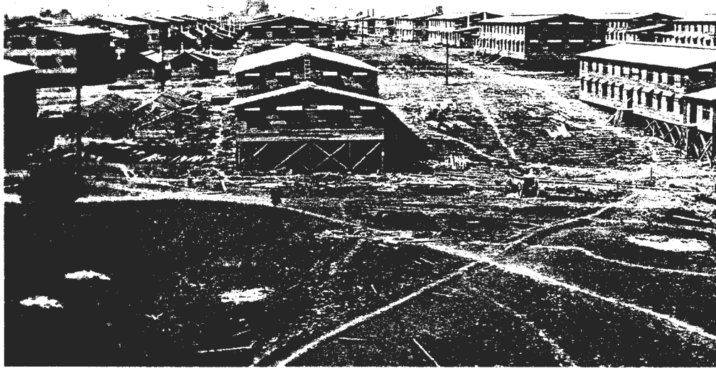
Figure 13: Construction of temporary World War I barracks at Camp Knox (Images of America: The Land Before Fort Knox).
