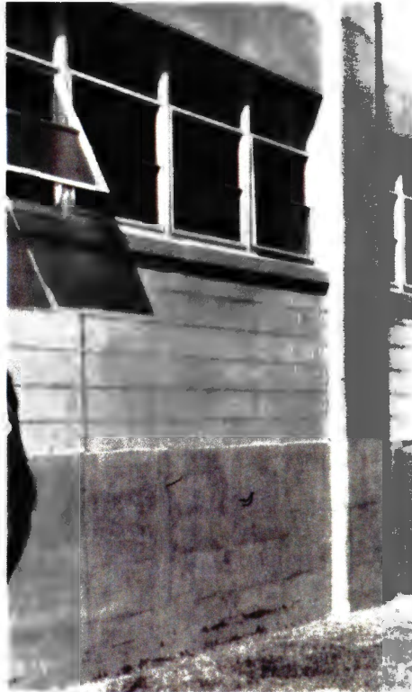
Original unpainted exposed concrete and concrete block with original steel awning windows
