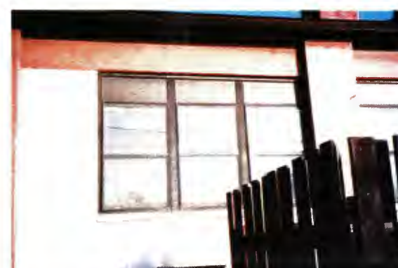
Building 297 - replacement anodized bronze window located on the southeast elevation of the kitchen wing
