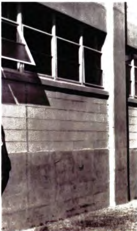
Original unpainted exposed concrete and concrete block with original steel awning windows
