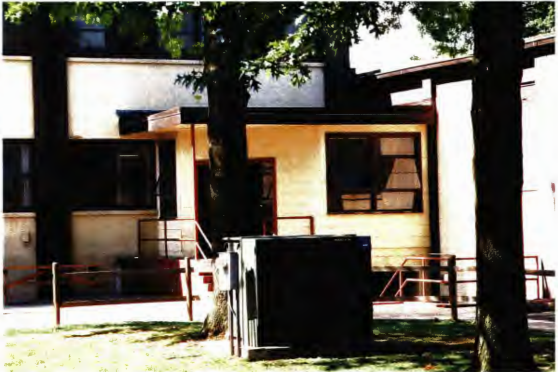
Building 2379 – entry located between the handle and the head on the north elevation
