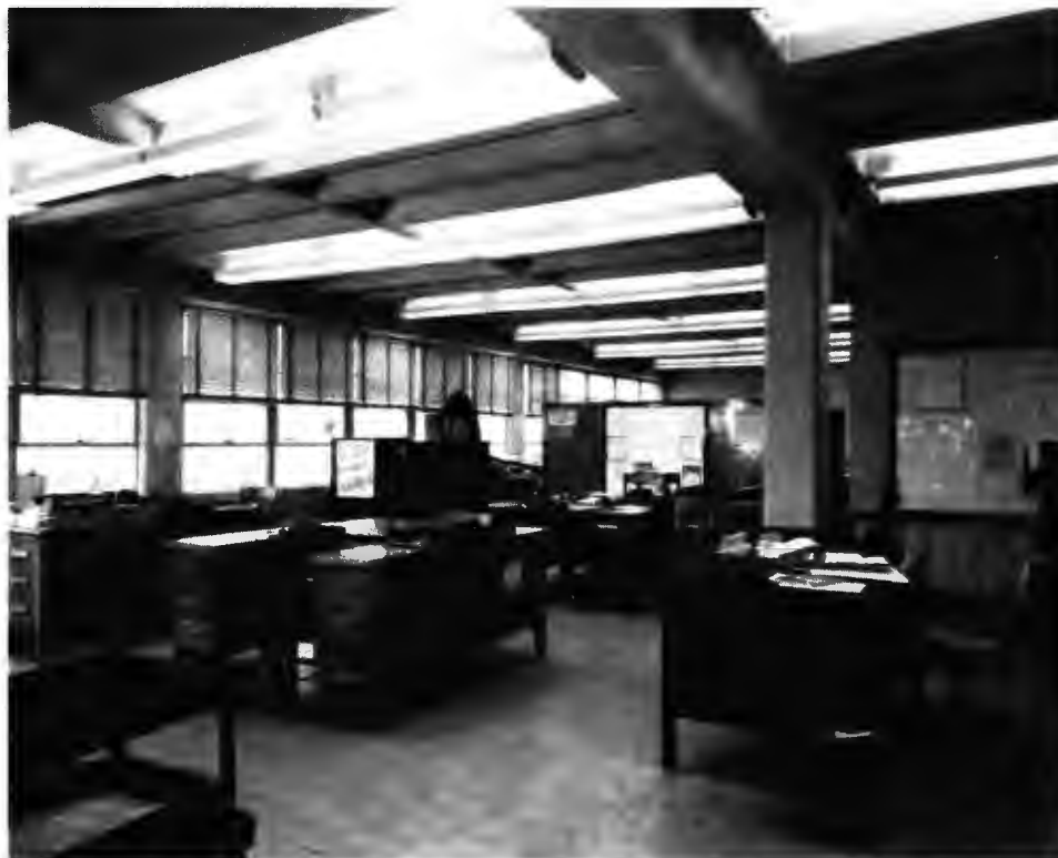
Interior view of Building 2370 depicting the concrete frame supports; similar to Building 1481 12 February 1957 (National Archives College Park)
