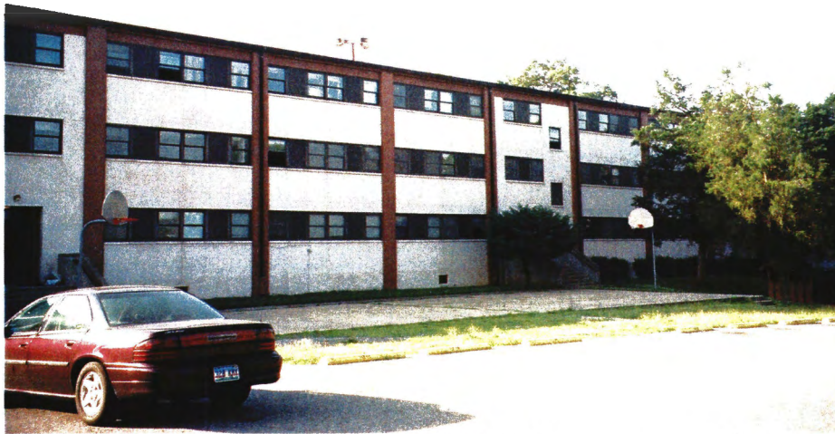
Figure 37: One of the modifications from the VOLAR program resulted in the removal of original steel awning windows being replaced with anodized bronze aluminum windows (ERDC-CERL).
