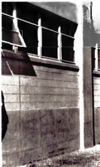
Original unpainted exposed concrete and concrete block with original steel awning windows
