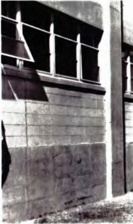
Original unpainted exposed concrete and concrete block with original steel awning windows
