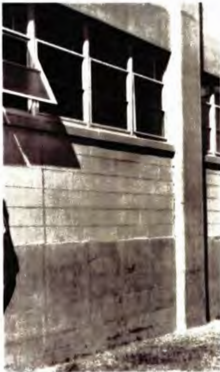
Original unpainted exposed concrete and concrete block with original steel awning windows
