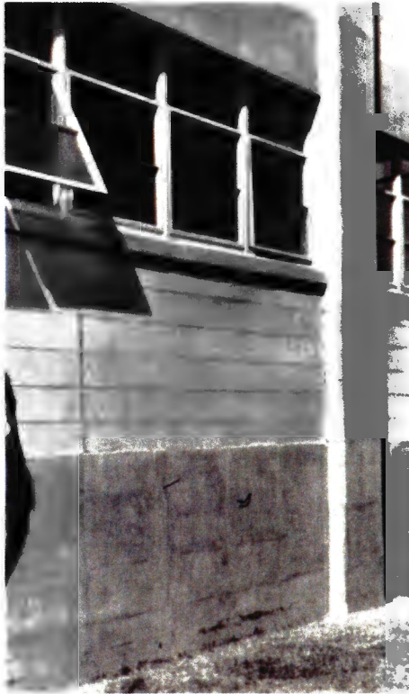
Original unpainted exposed concrete and concrete block with original steel awning windows
