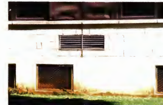
Building 1480 - newer air conditioner vent placed in the concrete block wall of the south elevation of the handle portion
