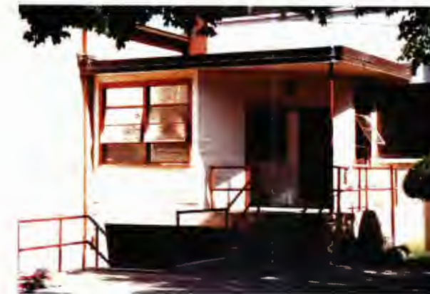
Building 1476 - south entrance between the head and handle portions, with original steel awning windows and asbestos siding
