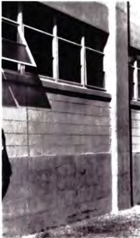
Original unpainted exposed concrete and concrete block with original steel awning windows
