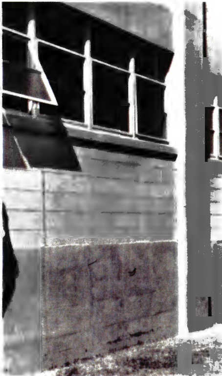
Original unpainted exposed concrete and concrete block with original steel awning windows
