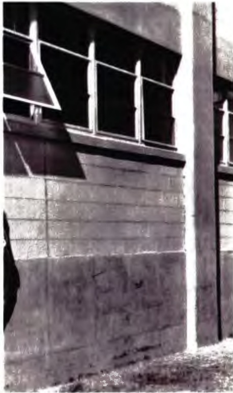
Original unpainted exposed concrete and concrete block with original steel awning windows
