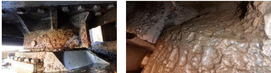
Figure 1. Pitting corrosion on a miter gate pintle.
