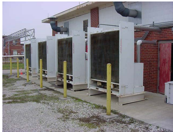
Figure H10. Inter and after coolers for compressors supplying Building #1.
