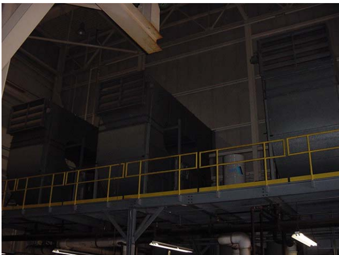
Figure J5. Compressor heat recovery ducts used for space heating during winter months.
