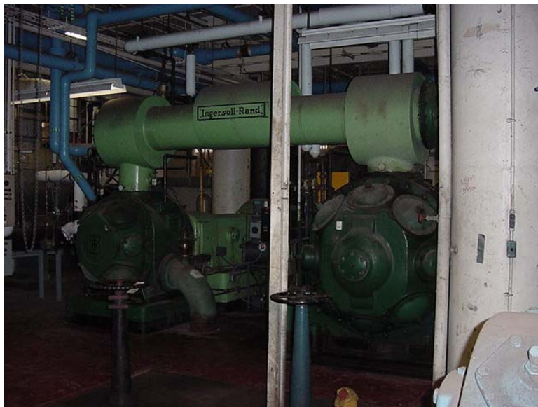
Figure J2. 4200 Ingersoll Rand reciprocating compressor.
