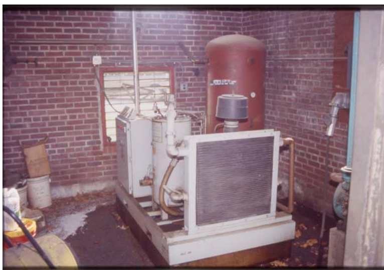
Figure G3. Building 315: 50 hp Rotary-Aire screw compressor.
