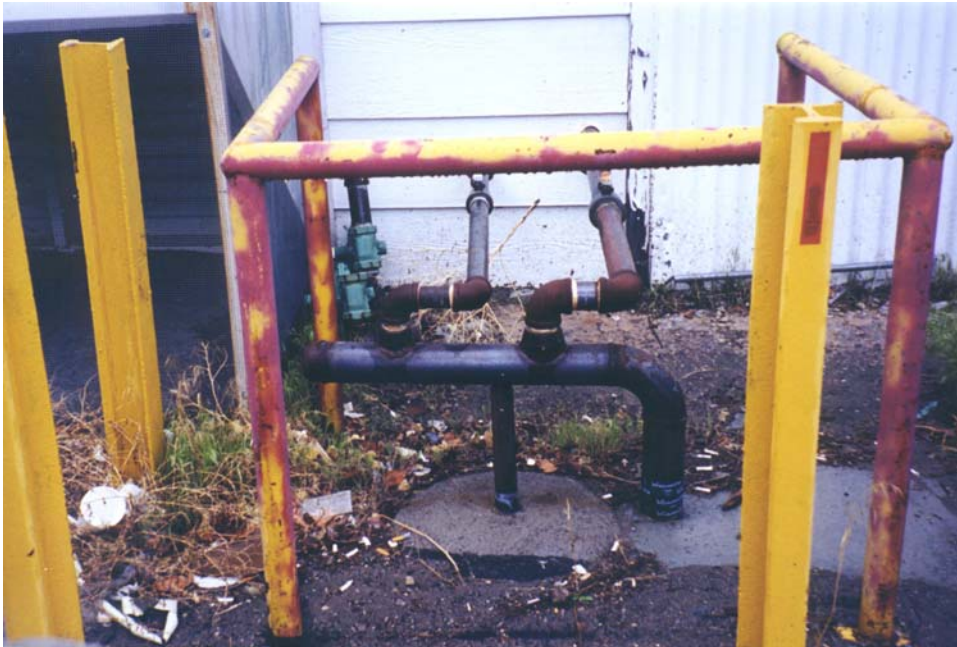
Figure K5. Stub-up for natural gas line.
