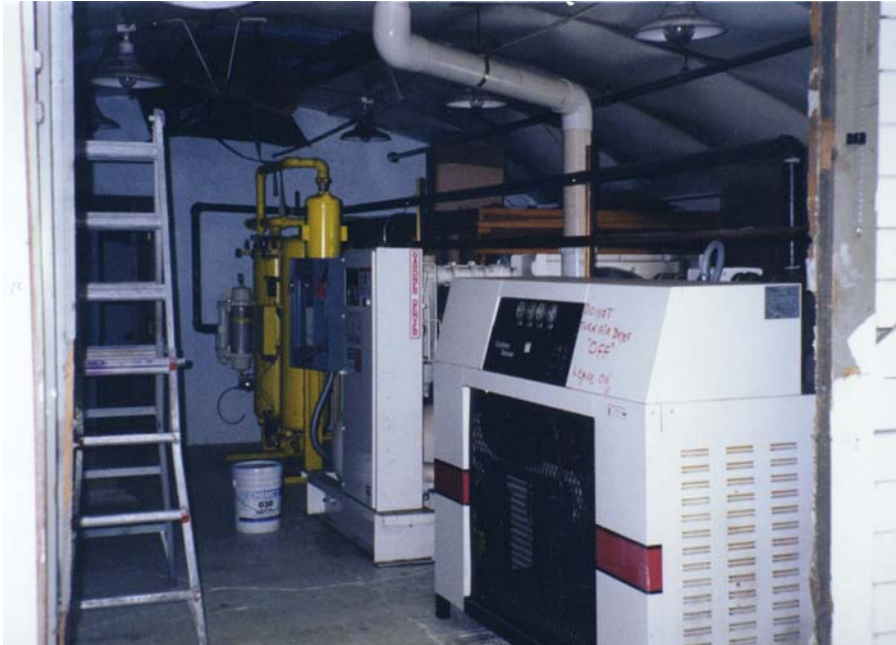
Figure K2. Building 210 Gardner Denver refrigerated dryer.
