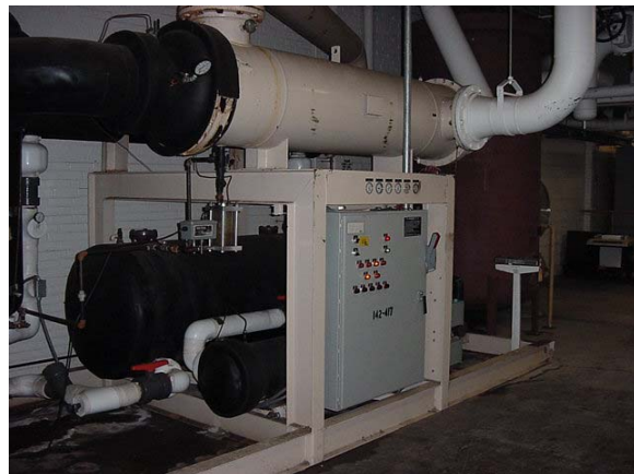
Figure H12. One of two refrigerated compressed air dryers for Building #1.
