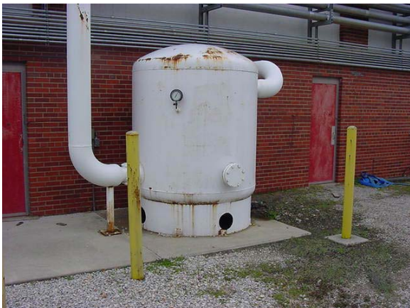
Figure H11. Air storage tank for Building #1 compressor room.
