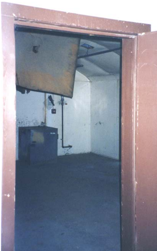
Figure K4. Second room in main compressor room enclosure: proposed NGEDAC location.
