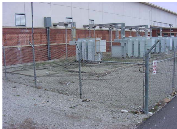
Figure H14. Potential outdoor site for natural gas engine driven air compressor.
