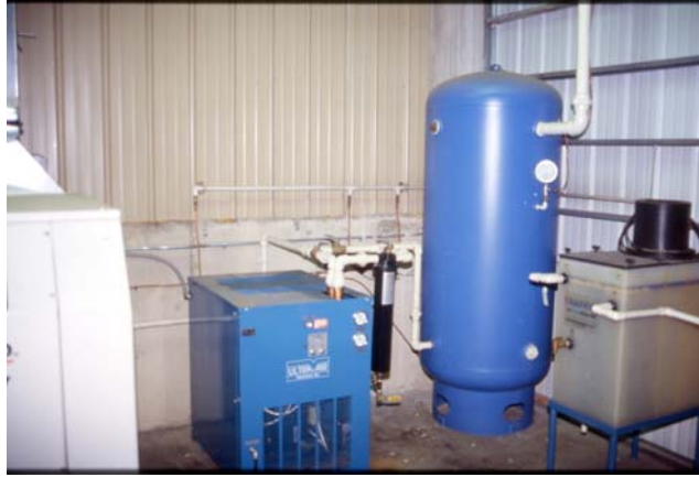
Figure G2. Building 525: dryer and receiver.
