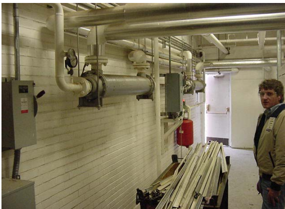
Figure H13. Oil heat recovery in Building #1 Compressor Room.
