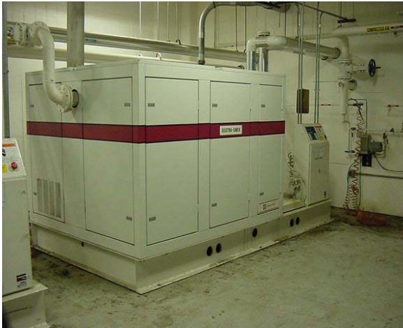
Figure H9. One of eight 500 hp screw compressors that supplies Building #1.
