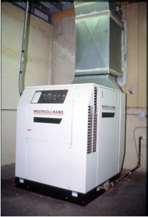
Figure G1. Building 525: 30 HP IR compressor.
