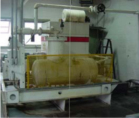
Figure H2. One of two 200 Hp screw compressors that supplies building #3.
