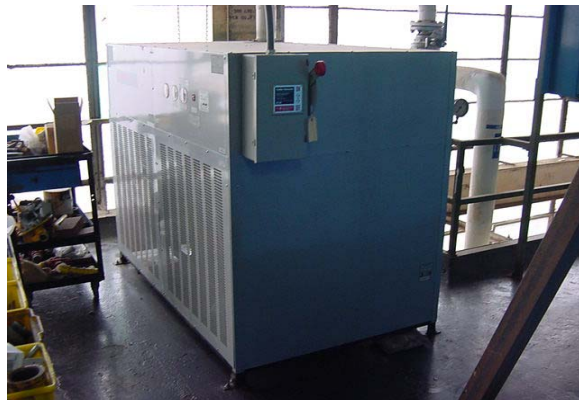
Figure H5. Refrigerated compressed air dryer located inside building #3.
