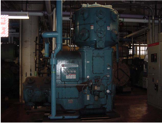
Figure J3. 2500 Ingersoll-Rand reciprocating compressor.
