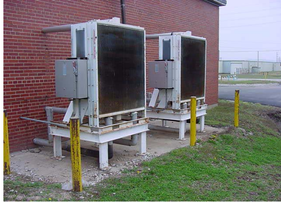
Figure H3. Inter and after coolers for compressors supplying building #3.
