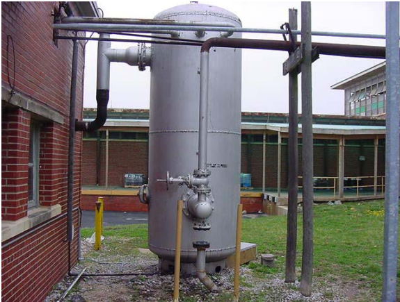
Figure H4. Building #3 air storage tank outside of compressor building.
