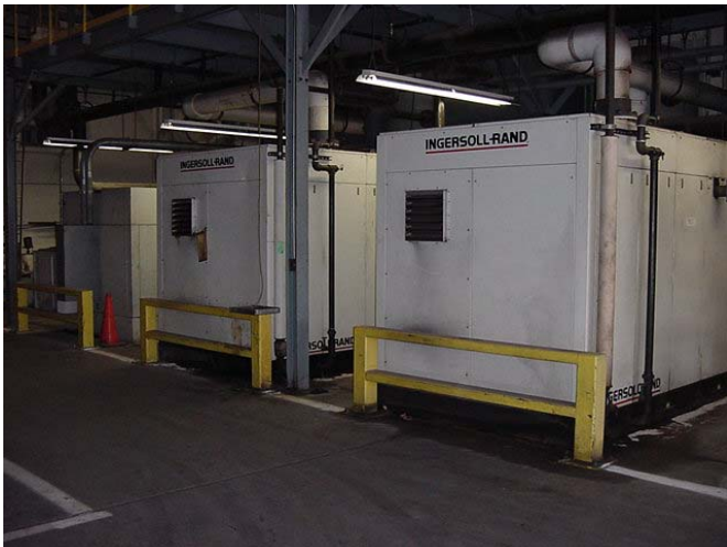
Figure J4. Three air compressors in building 222.
