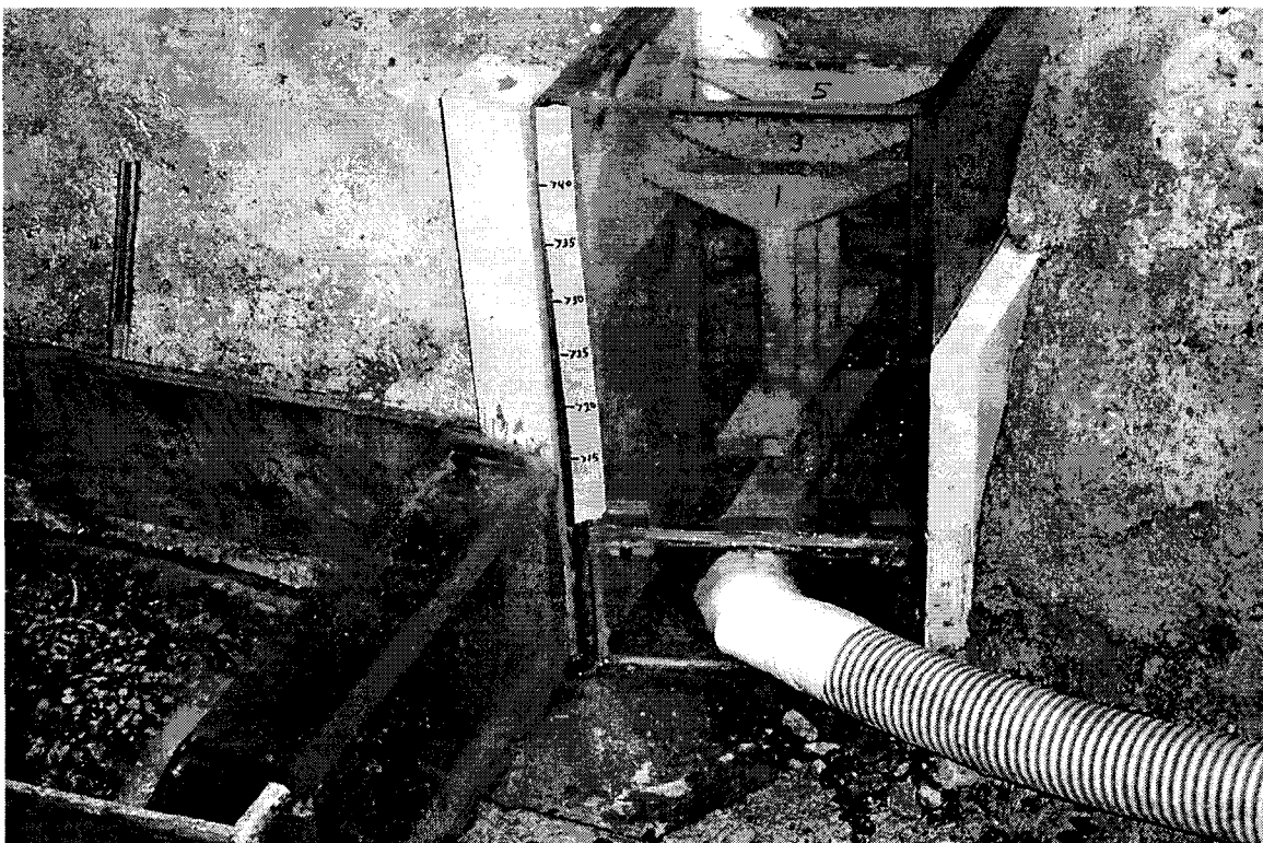
Figure 3. Intake wells for three fusegates (located on the right spillway abutment)
