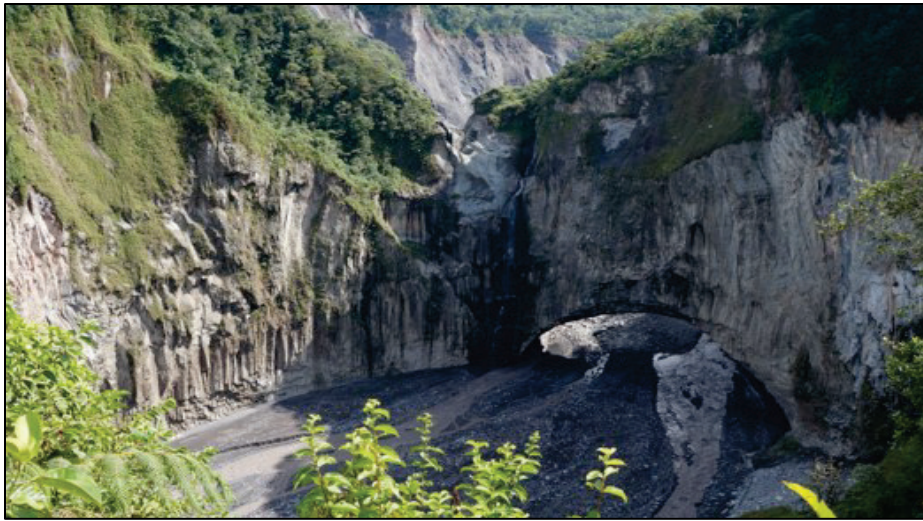
Figure 2. Piping failure conditions at the San Rafael Waterfall location (provided by US Army Corps of Engineers [USACE], Mobile District).
