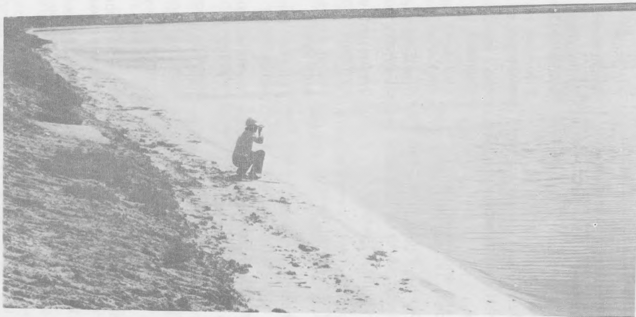
Figure 12. Shrimp culture pond in Containment Area No. 85 showing berm and beach caused by wave action. Such berms protect the levee from further erosion.
