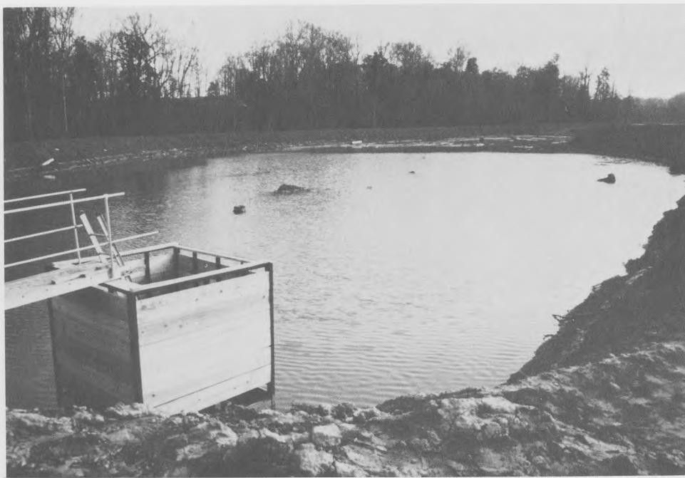
Photo 16. Vicksburg, Miss., disposal area; small ponded containment area with effluent sluice in foreground
