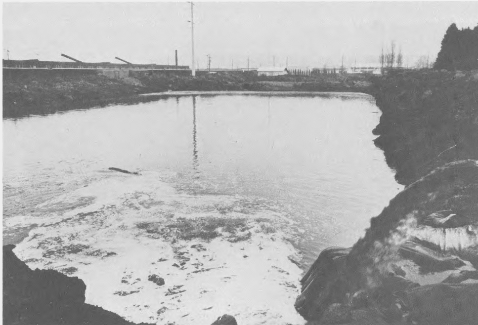
Photo 13. Seattle, Wash., disposal area; influent discharge from pneumatic pipeline dredge into compartment 1
