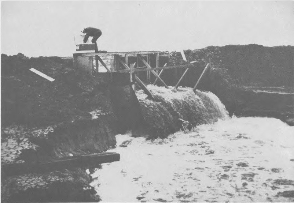
Photo 12. Lake Charles, La., disposal area; discharge over weir from disposal area No. 22
