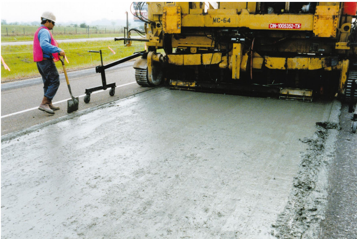
Figure 44. FRC as placed by a slipform paving machine on the USAEWES whitetopping test section
