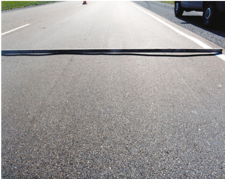
Figure 32. Typical rutting of HMA pavement on I-20 at the site of whitetopping demonstration project
