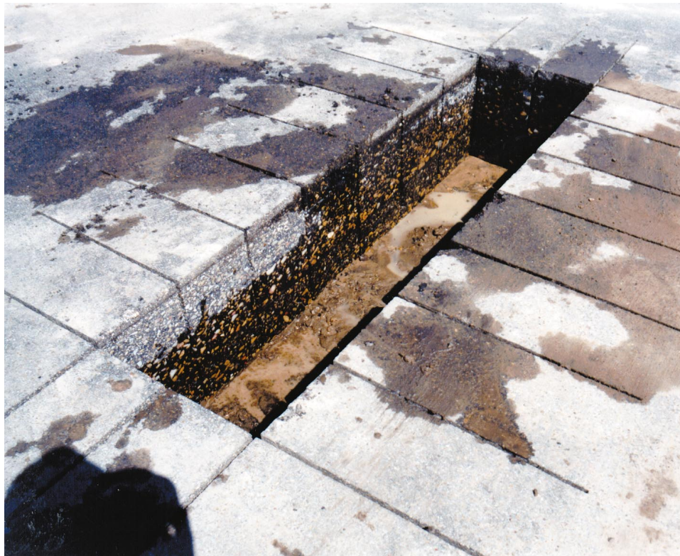
Figure 35. Blocks of HMA pavement sawed from I-20 at the site of the whitetopping demonstration project
