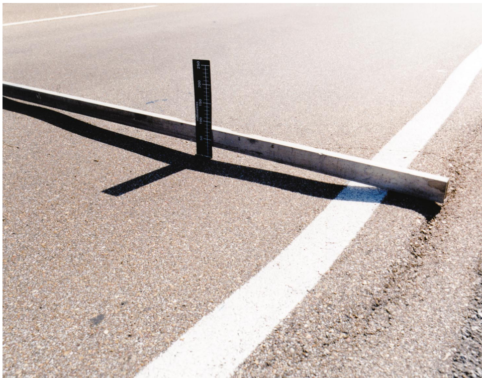
Figure 33. Closeup view of rutting
