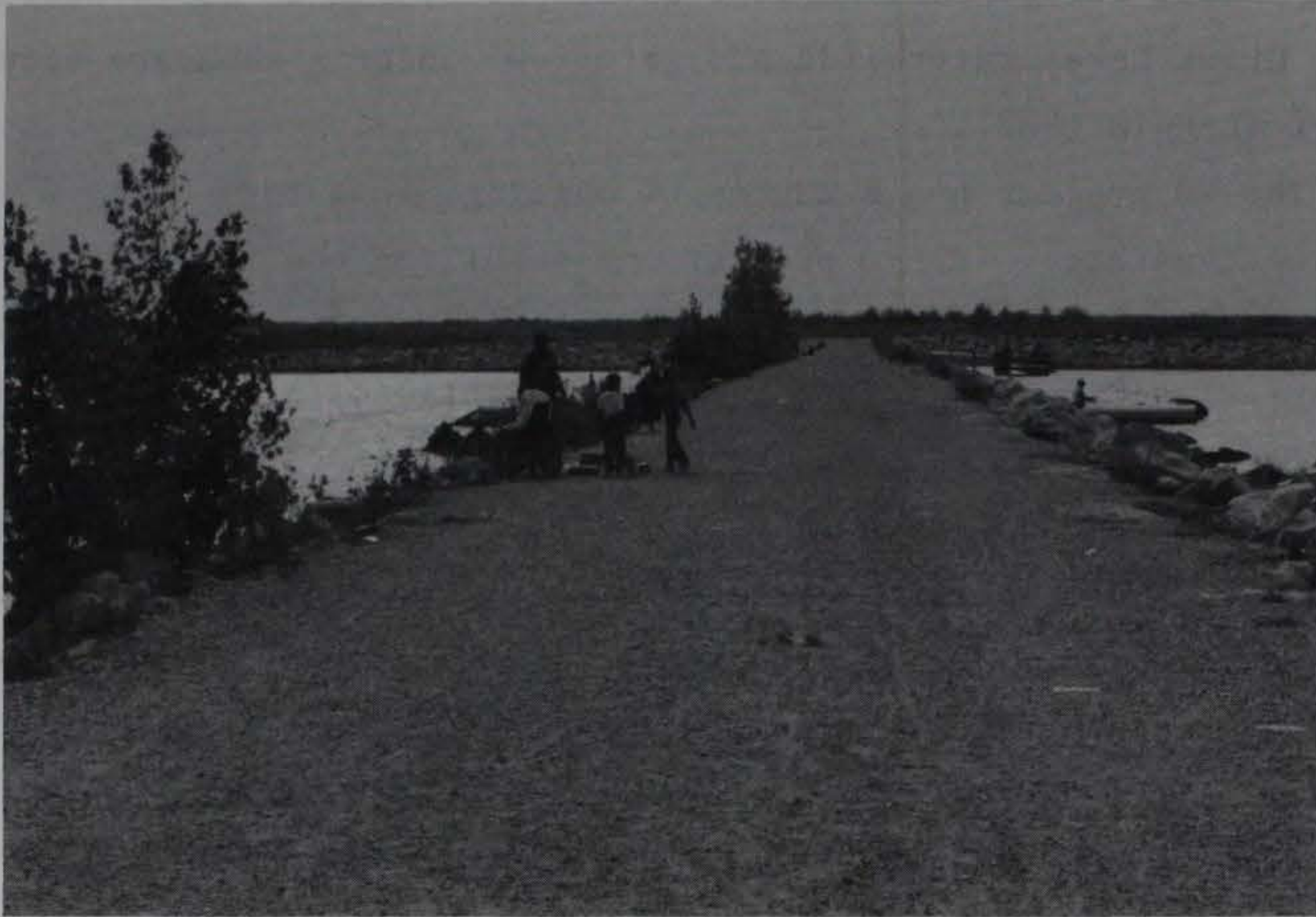
Figure 11. Exterior and interior of all dikes in the CDF and exterior of access crossdikes were armored with heavy stone underlain with erosion control fabric to prevent failure of the dikes
