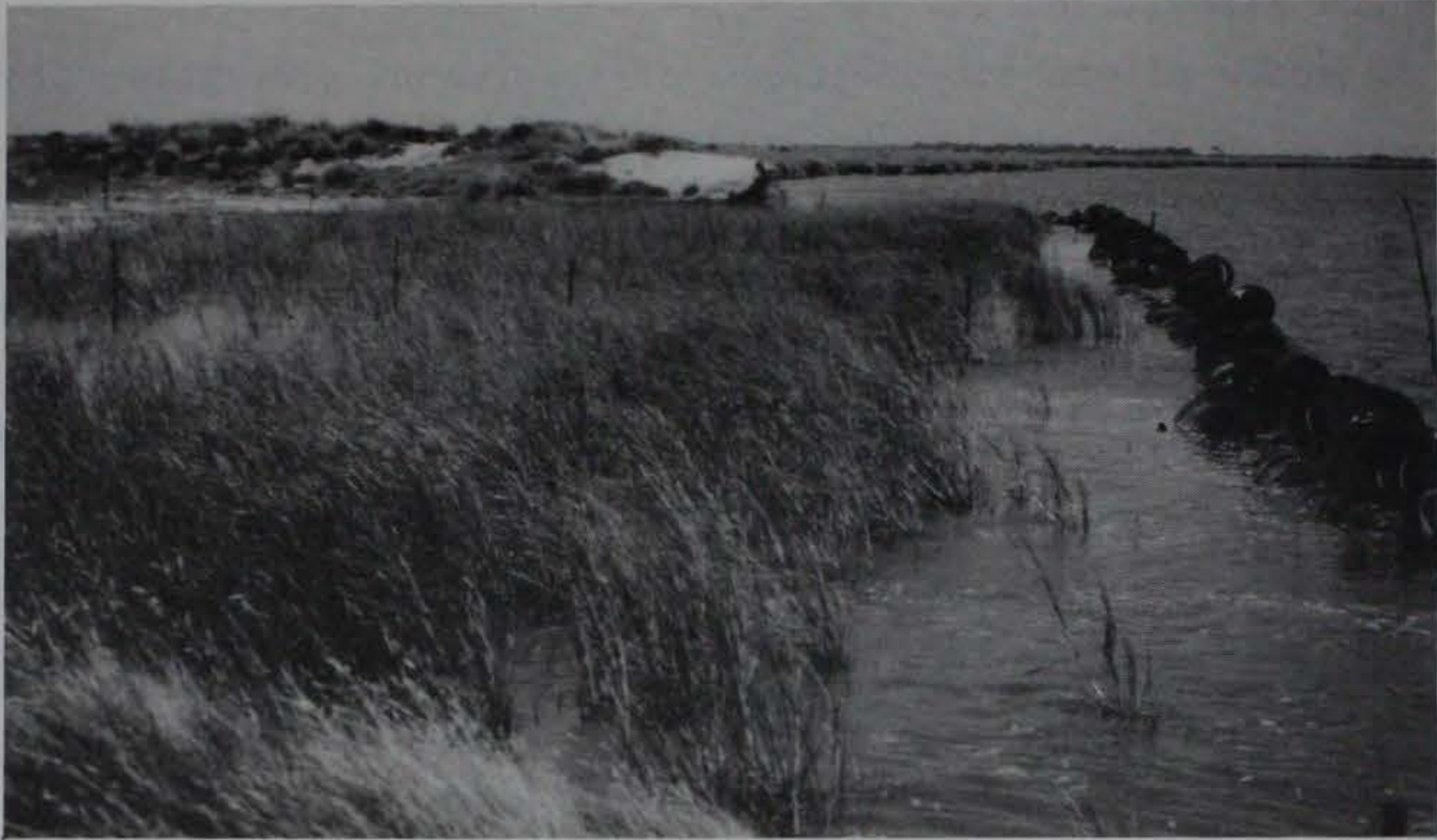
Figure 7. Planted saltmarsh at GI after two growing seasons, planted behind a floating-tire breakwater
