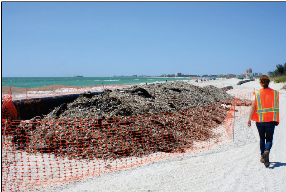
Figure 18. Oversized material separated by the FRS during a beach nourishment project on Treasure Island, Florida. Note Norfolk Dredging's 24 in. (610 cm) discharge diameter cutterhead dredge Charleston in far background, pumping ashore.
