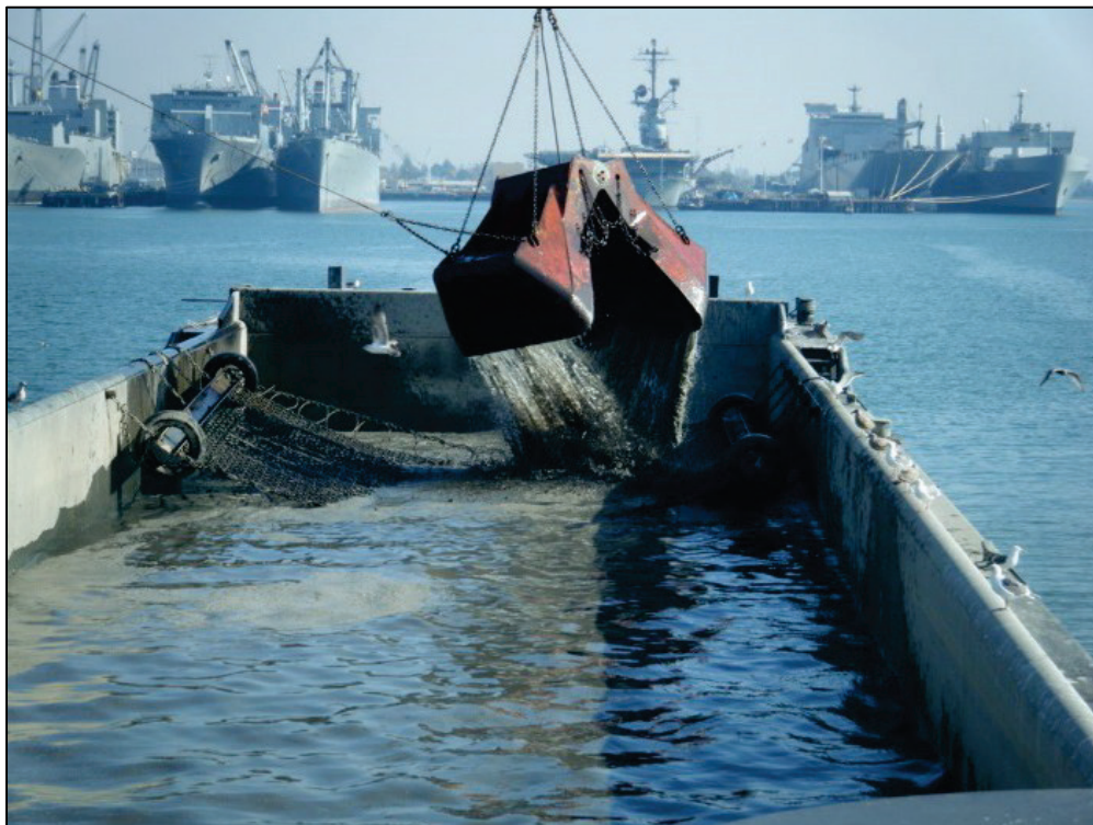
Figure 11. Barge screen constructed of chain used in a CA dredging project (Hoffman et al. 2015).
