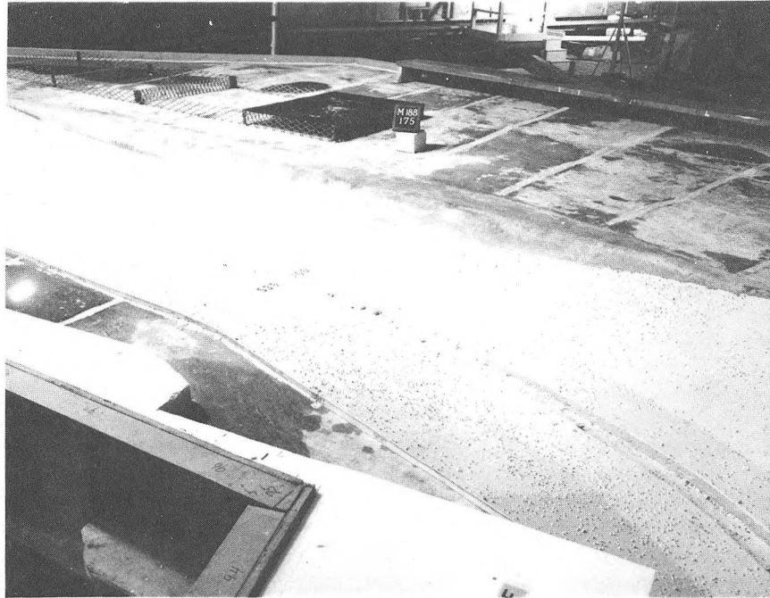
Photograph 12. Verified concrete channel at station 535+00, rolling mill building and flood wall in foreground
