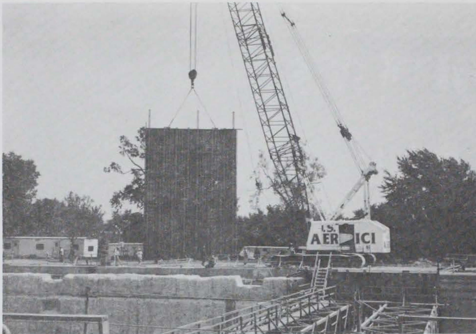
Figure 175. Concrete form being placed in position on the lock wall, Brandon Road Lock
