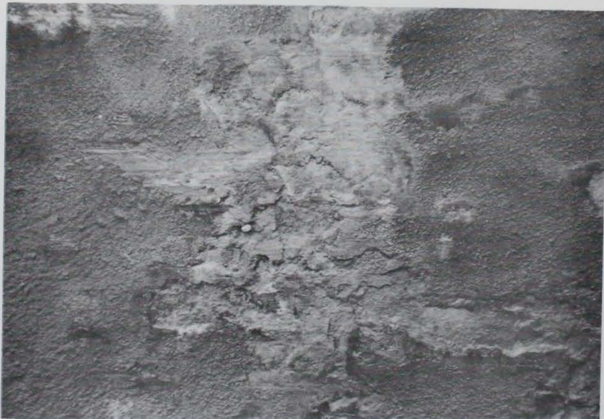
Figure 124. Typical examples of Fibercrete condition, February 1981, Emsworth Locks
