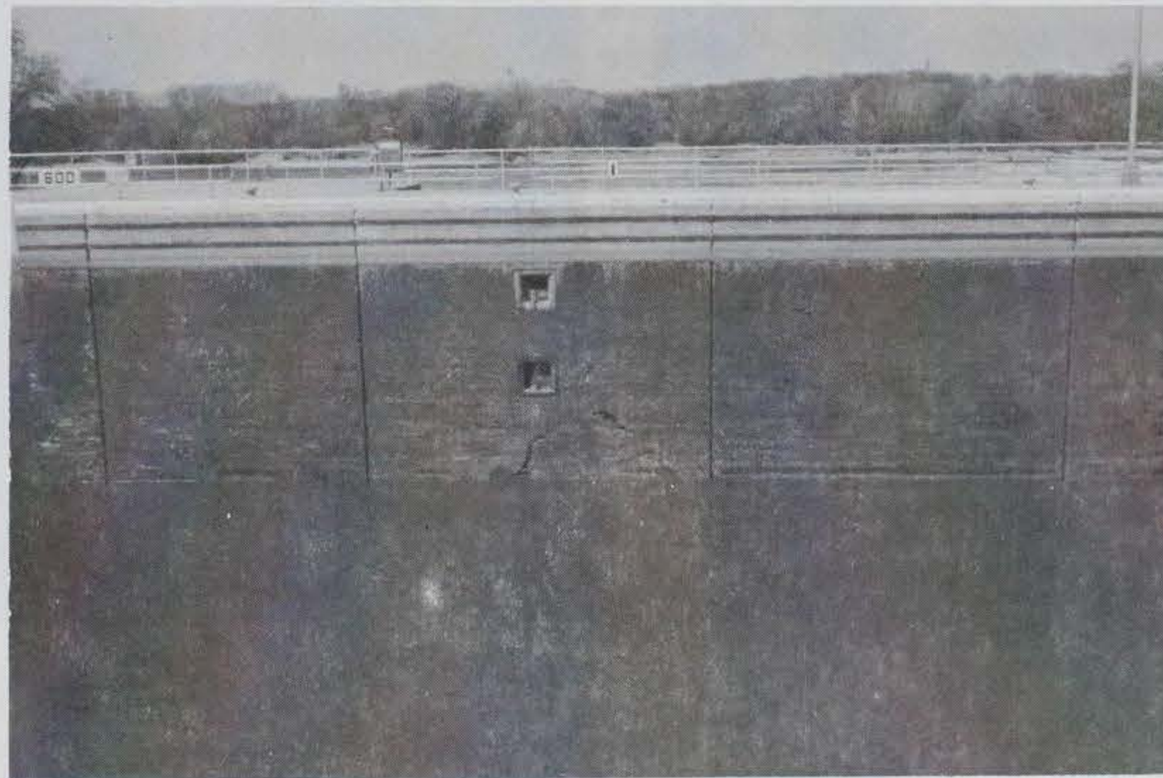
Figure 42. Condition of replacement concrete, 1986 Dresden Island Lock
