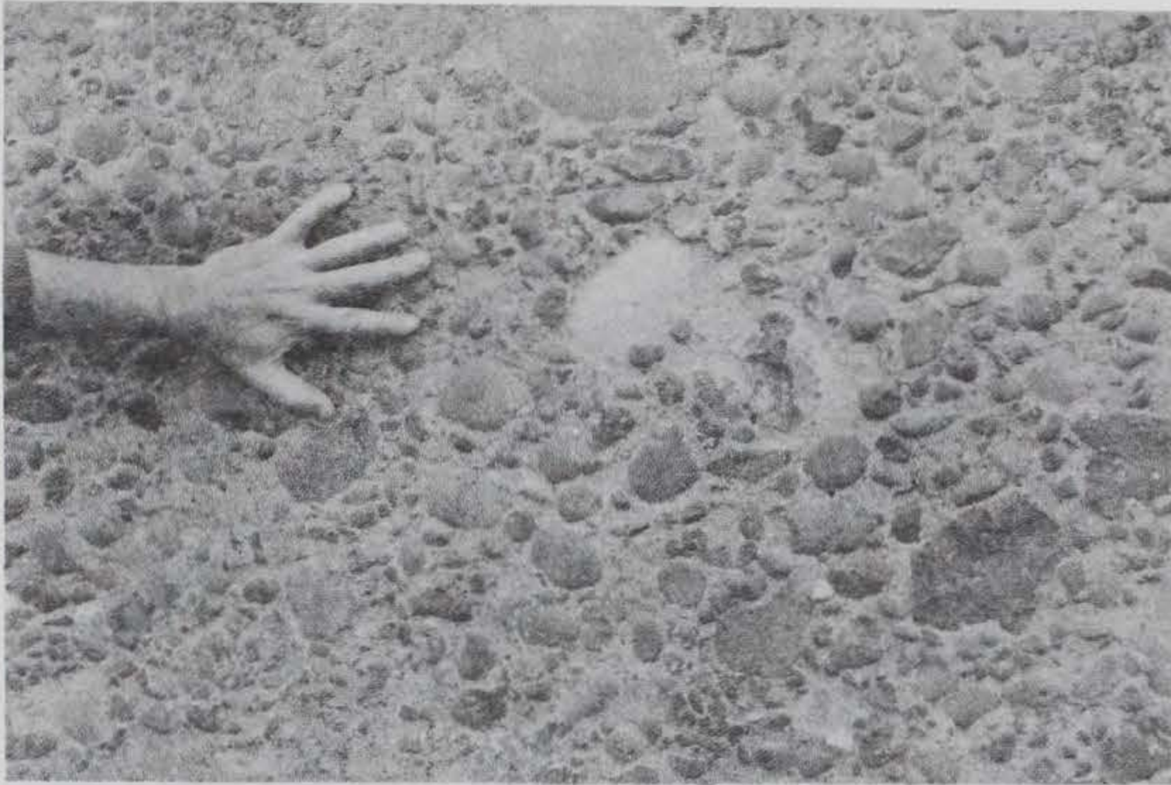
Figure 114. Typical condition of the wall following acceptable surface preparation, Lower Monumental Lock
