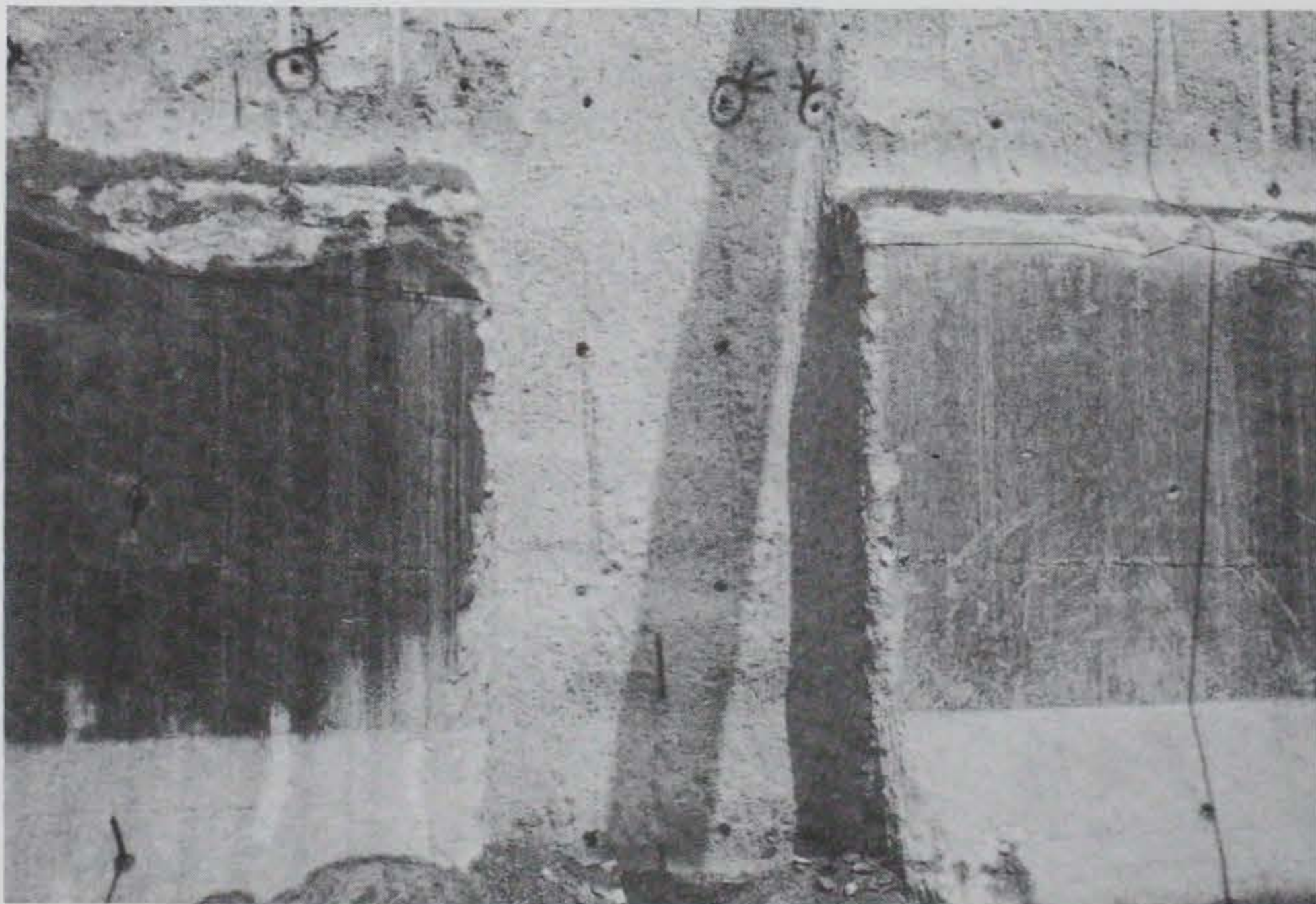
b. Lock chamber exit ladder cut
