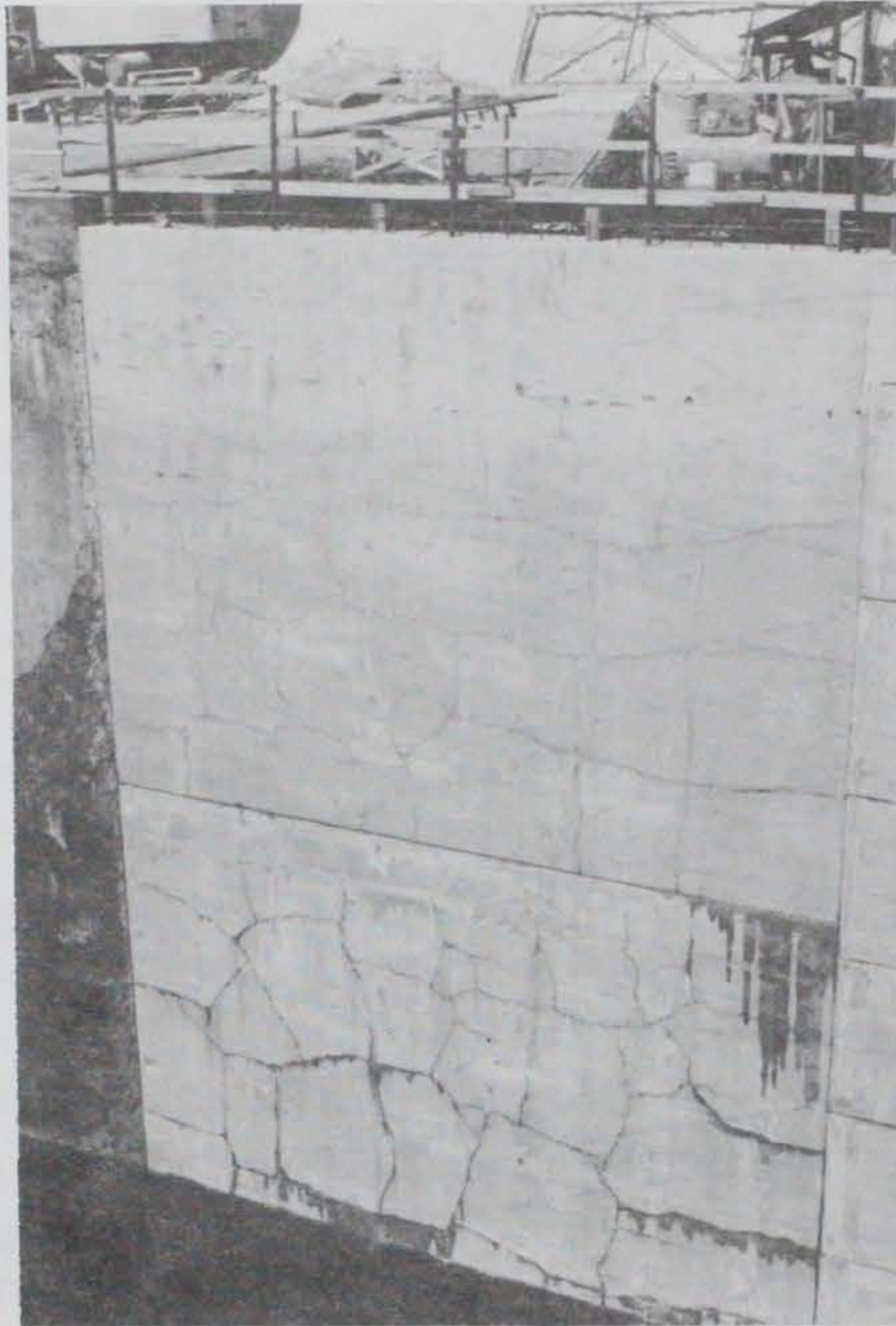
Figure 89. Cracking in replacement concrete, trial resurfacing monolith, 10 June 1980, Lock No. 1, Mississippi River
