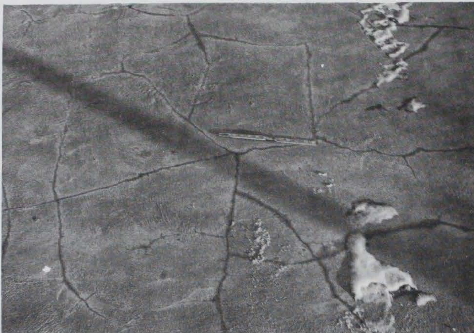
a. Pattern cracking, top surface
