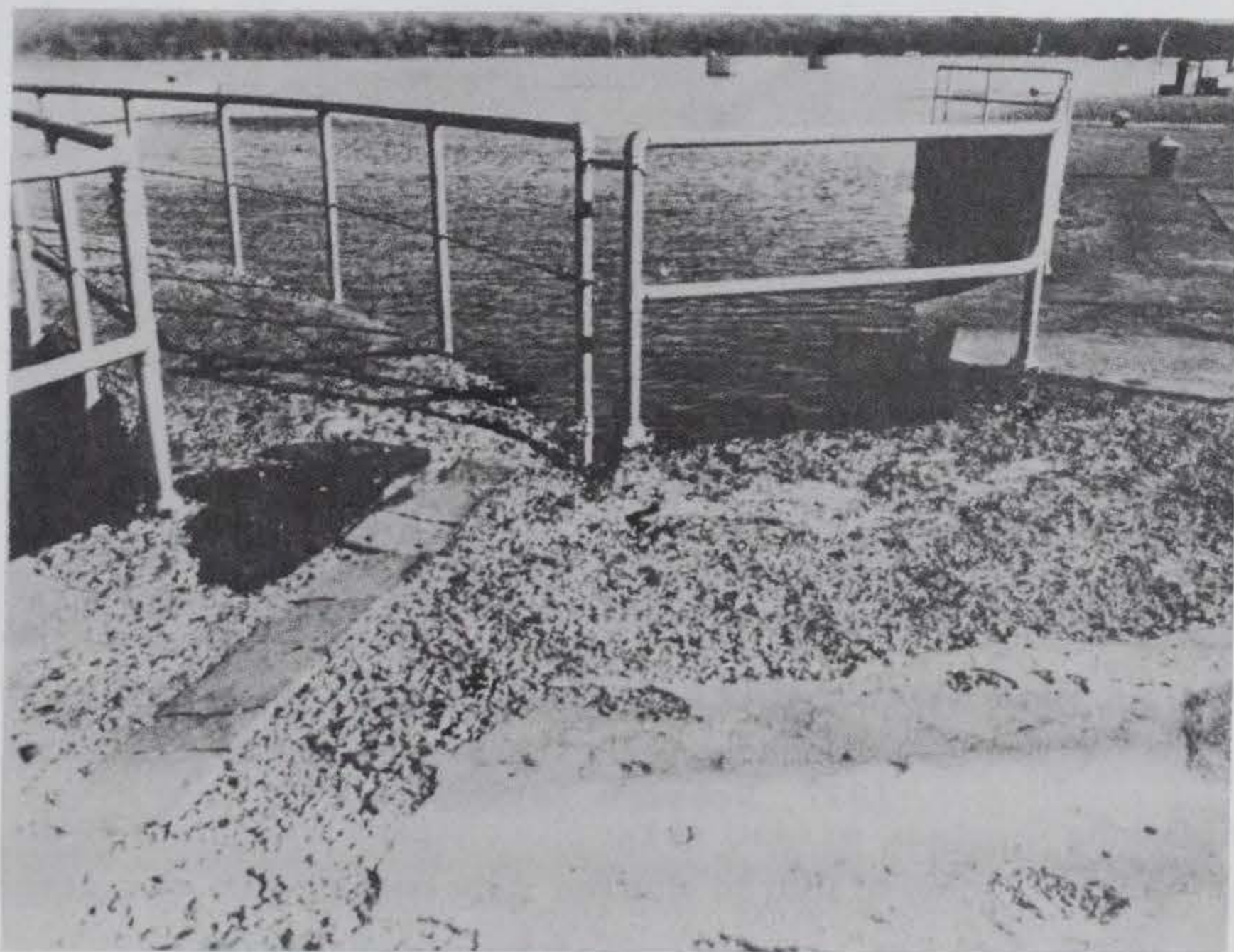
Figure 29. Typical concrete deterioration on tops of lock walls, 1961, Dresden Island Lock and Dam
