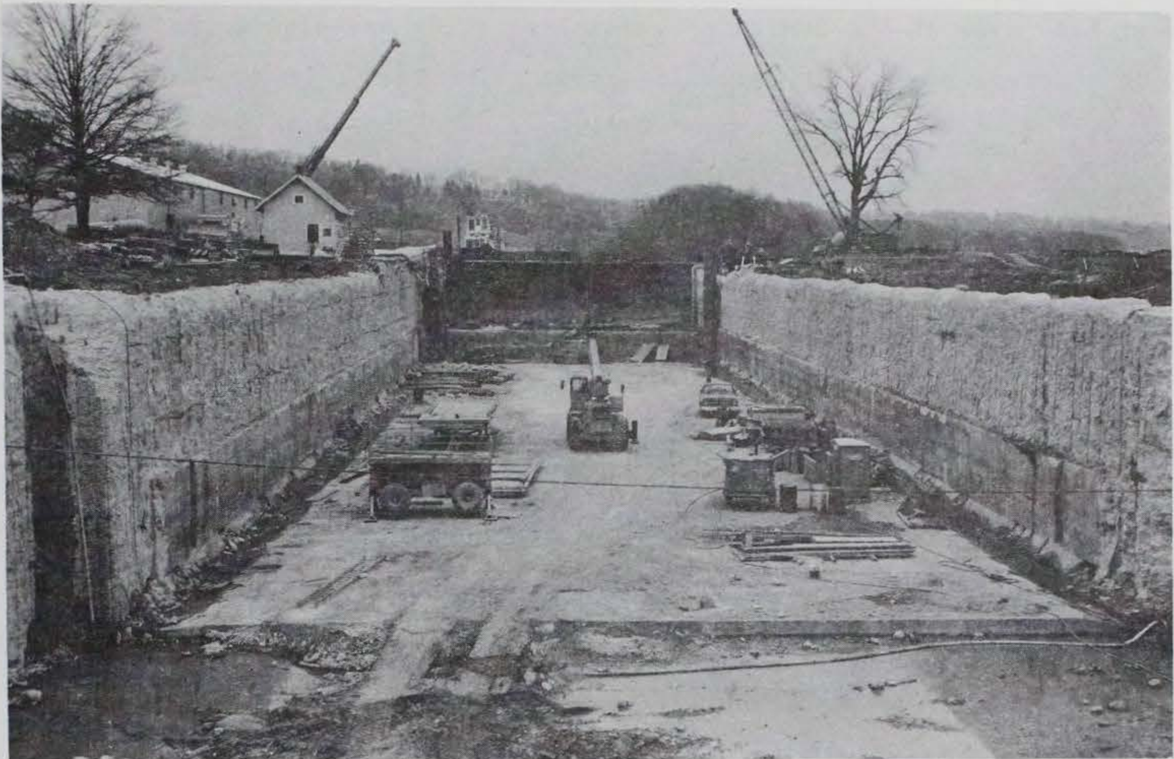
Figure 22. Lock walls following removal of deteriorated concrete, April 1980, Old Lock No. 14, Mississippi River
