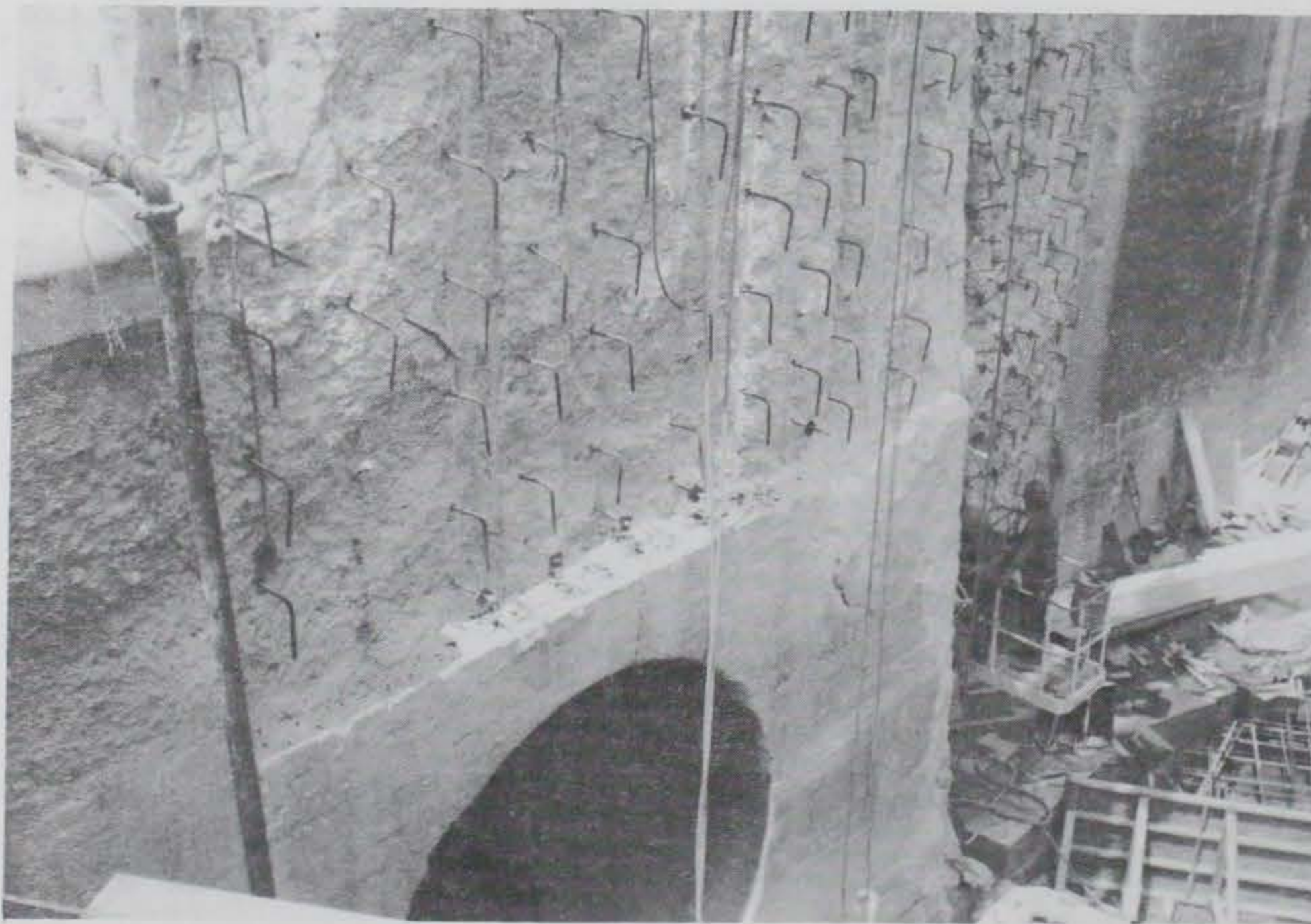
b. Crack in top of culvert to be grouted
