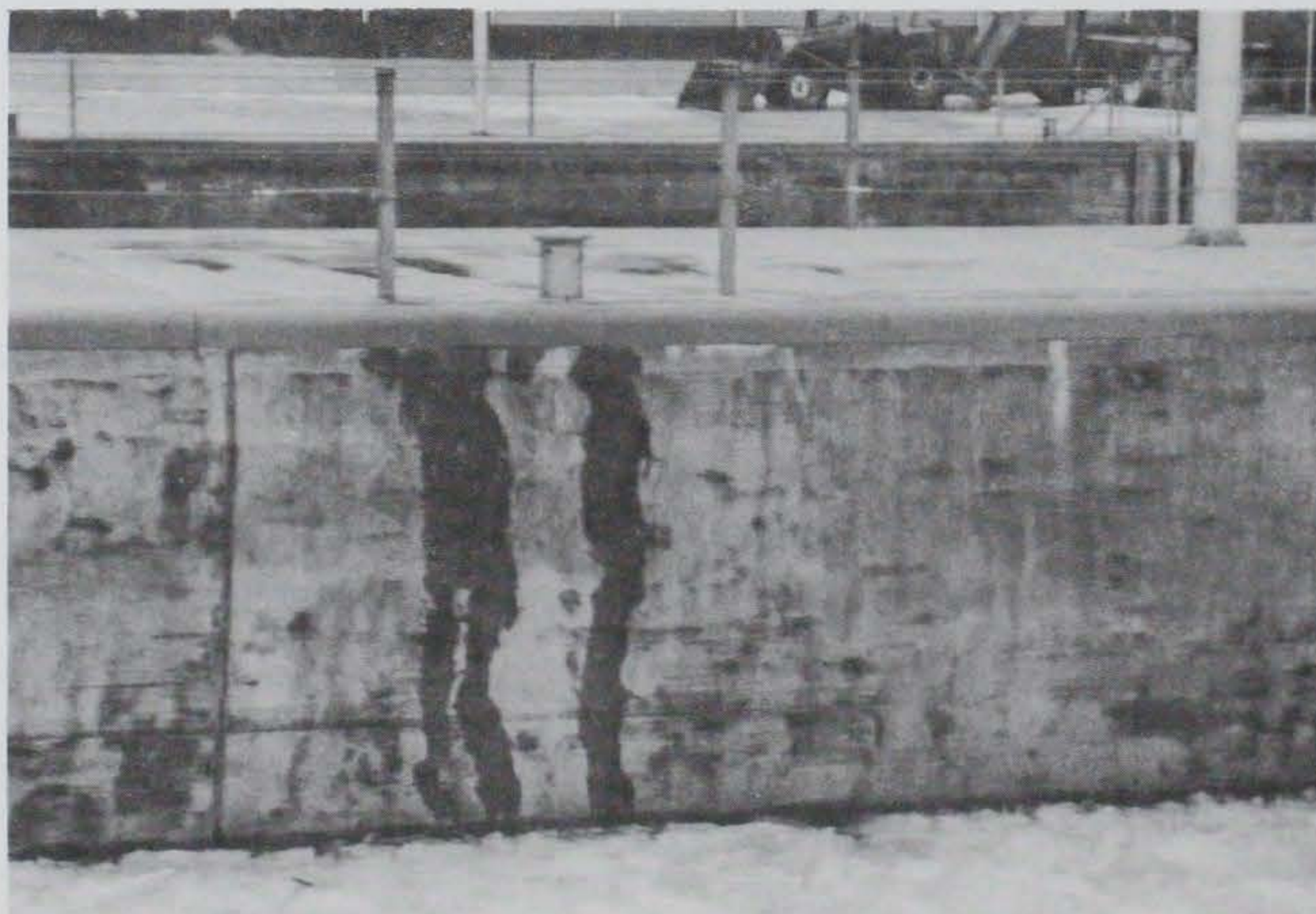
b. Seepage on chamber face as a result of water ponding on top surface
