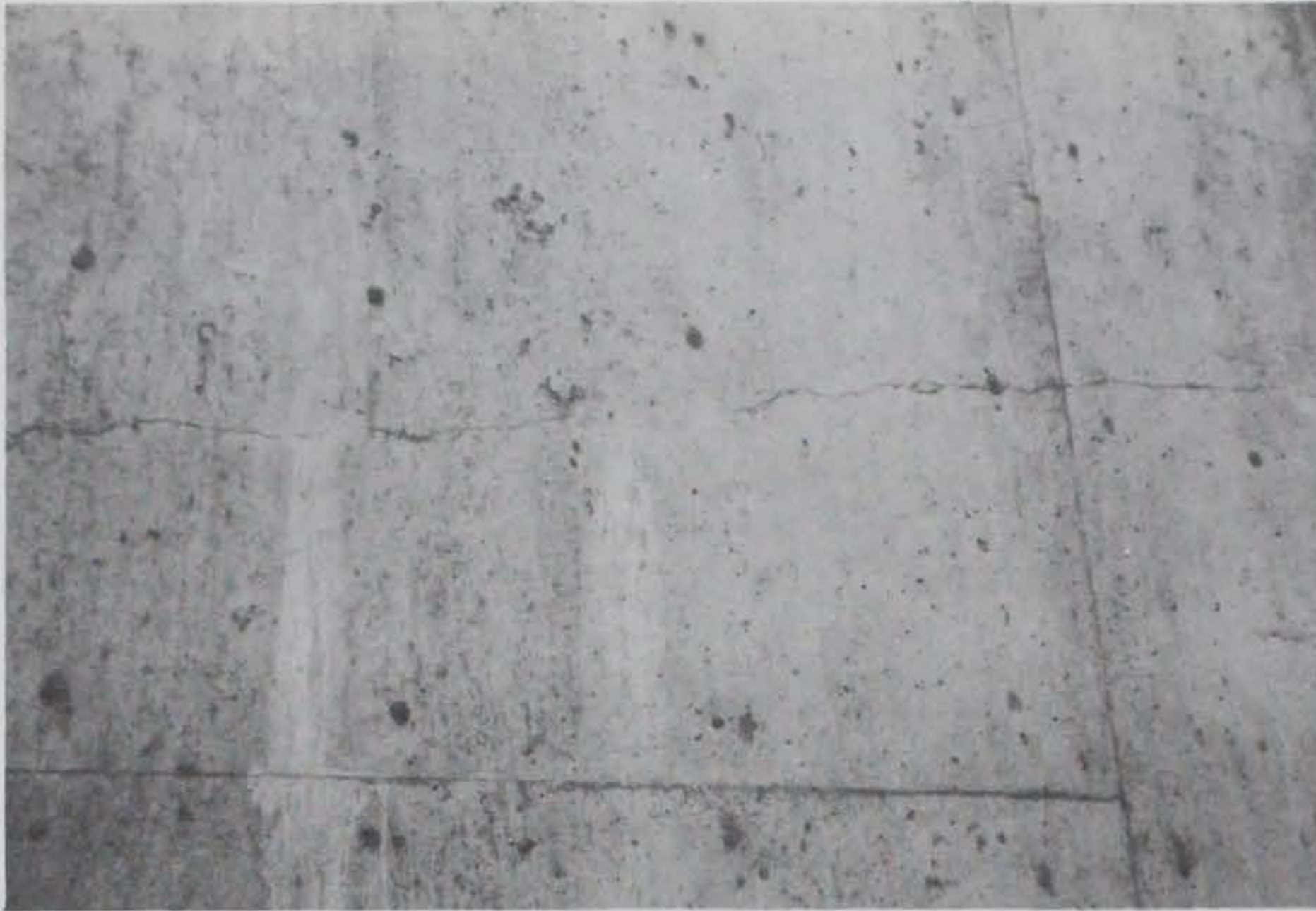
Figure 180. Typical crack in replacement concrete, August 1984, Brandon Road Lock
