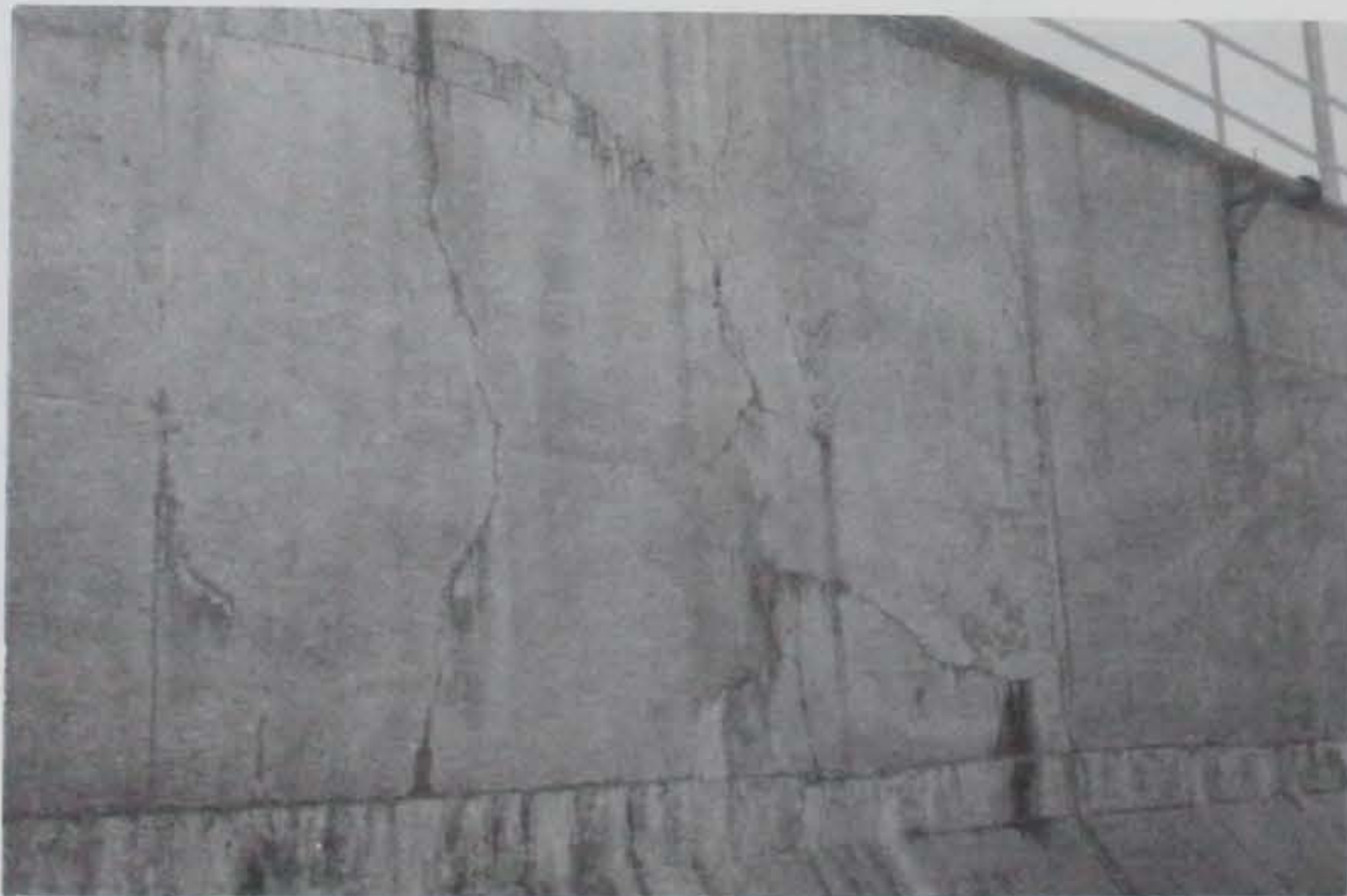
Figure 43. Typical condition of concrete overlay on back side of river wall, 1986, Dresden Island Lock
