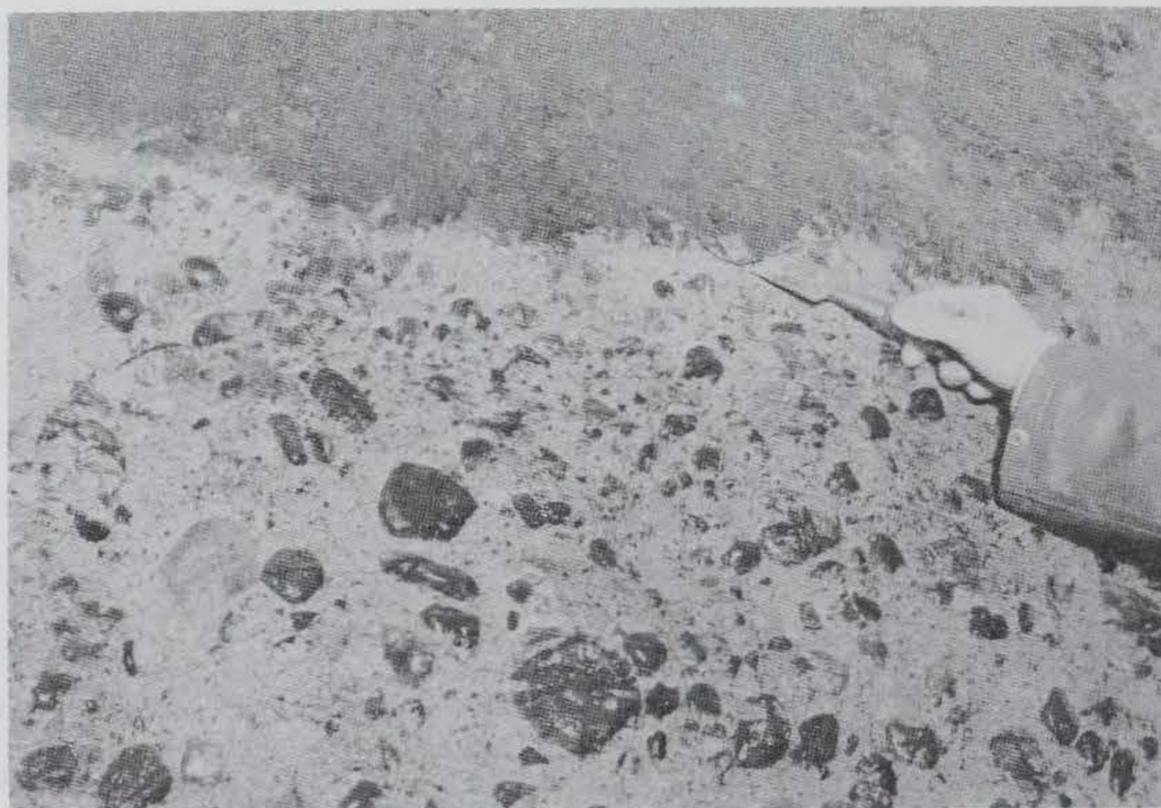
Figure 113. Examples of how easily the unsound surface mortar could be removed, Lower Monumental Lock
