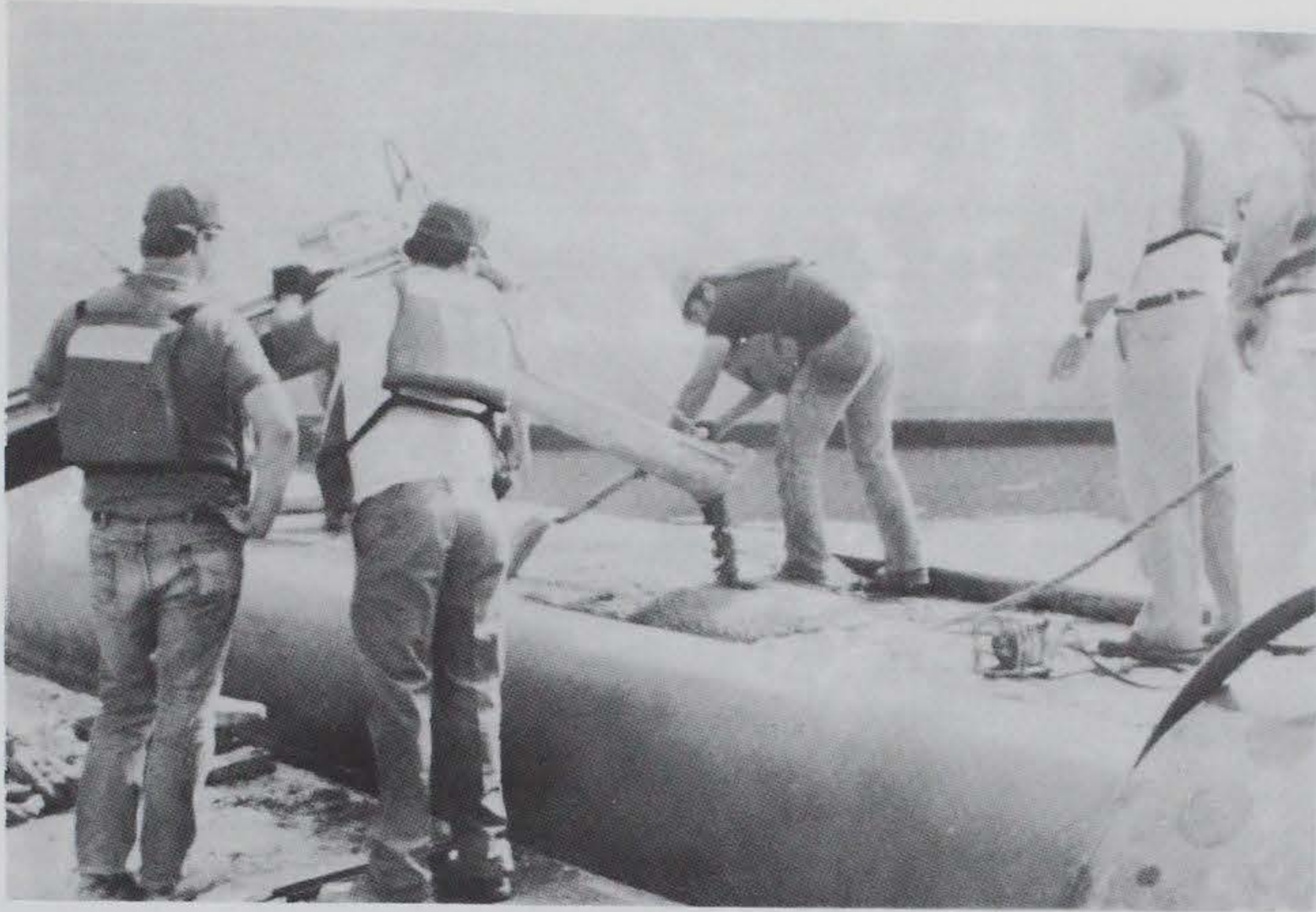
Figure 187. Resurfacing top of the upper guide wall with latex-modified concrete, Brandon Road Lock
