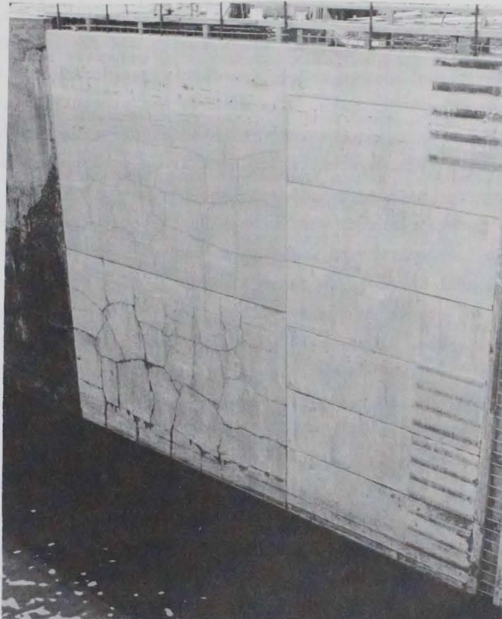
Figure 107. Concrete cracking in a resurfaced monolith (left) compared to reconstructed monolith, Lock No. 1, Mississippi River
