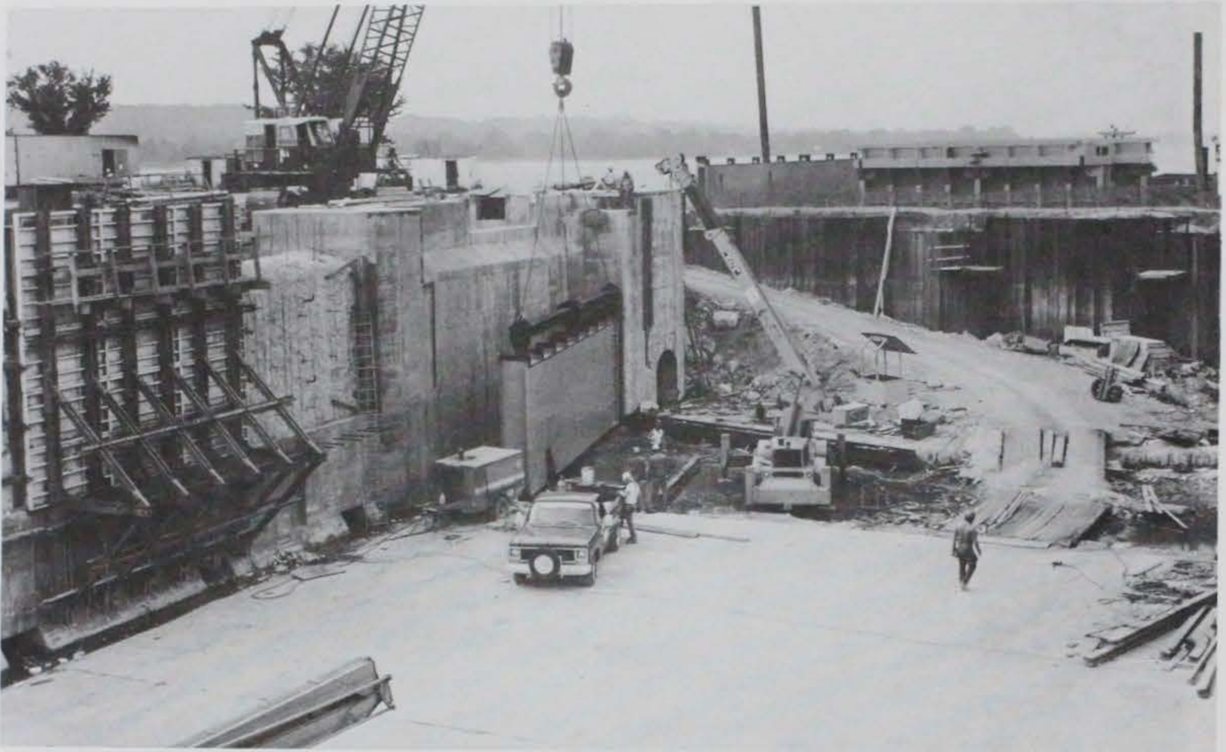
Figure 23. Concrete forming system and gate installation, August 1980, Old Lock No. 14, Mississippi River
