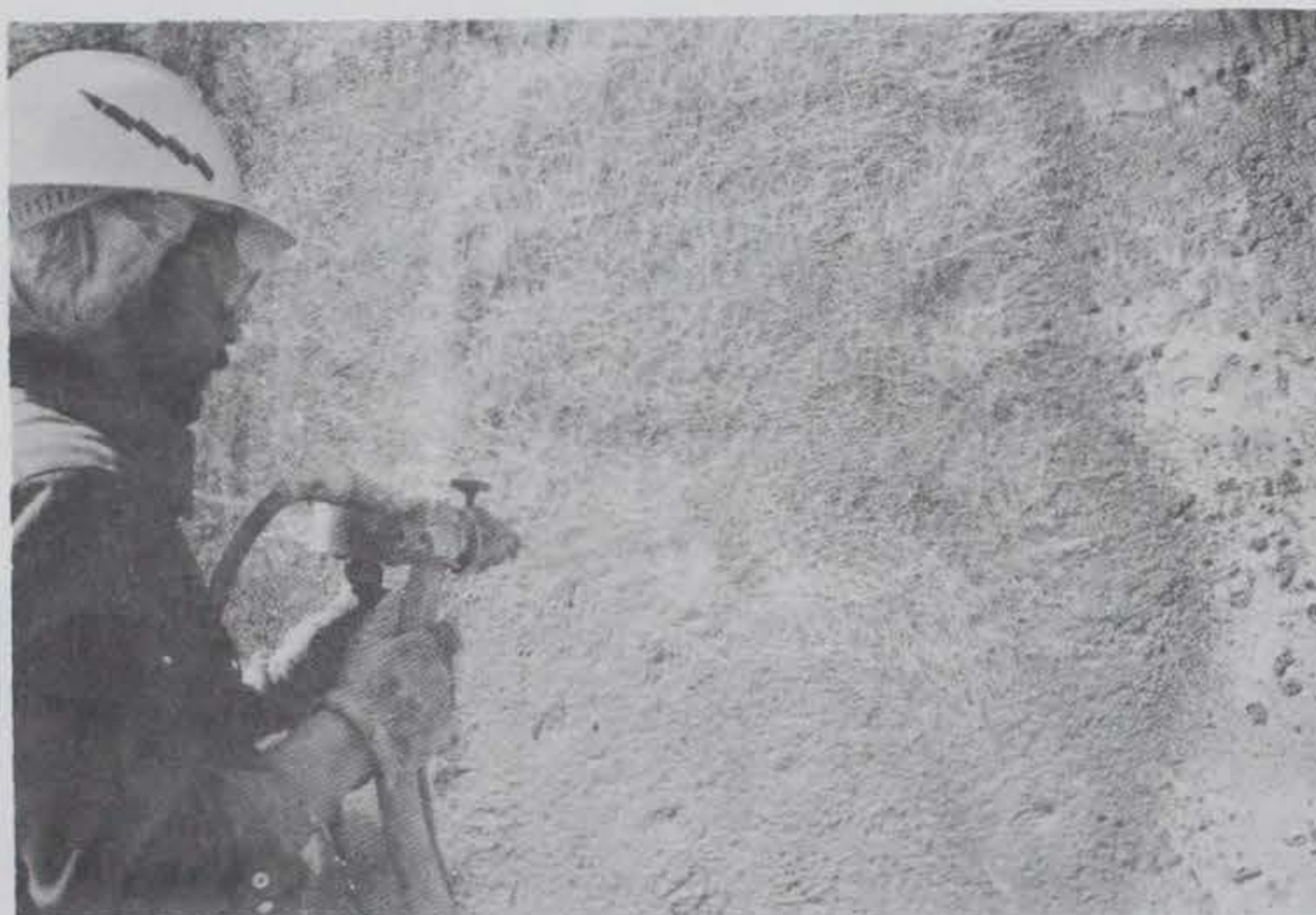
Figure 117. Coating application in an area of minimal scaling near the top of the lock, Lower Monumental Lock
