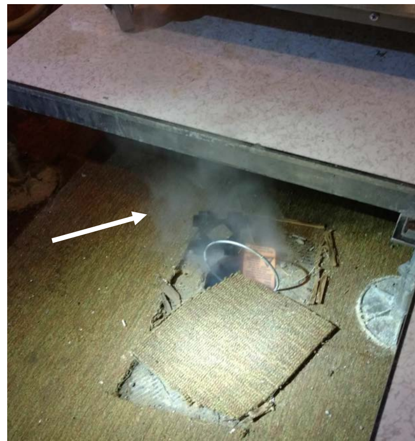
Open Pipe Beneath Raised Floor
