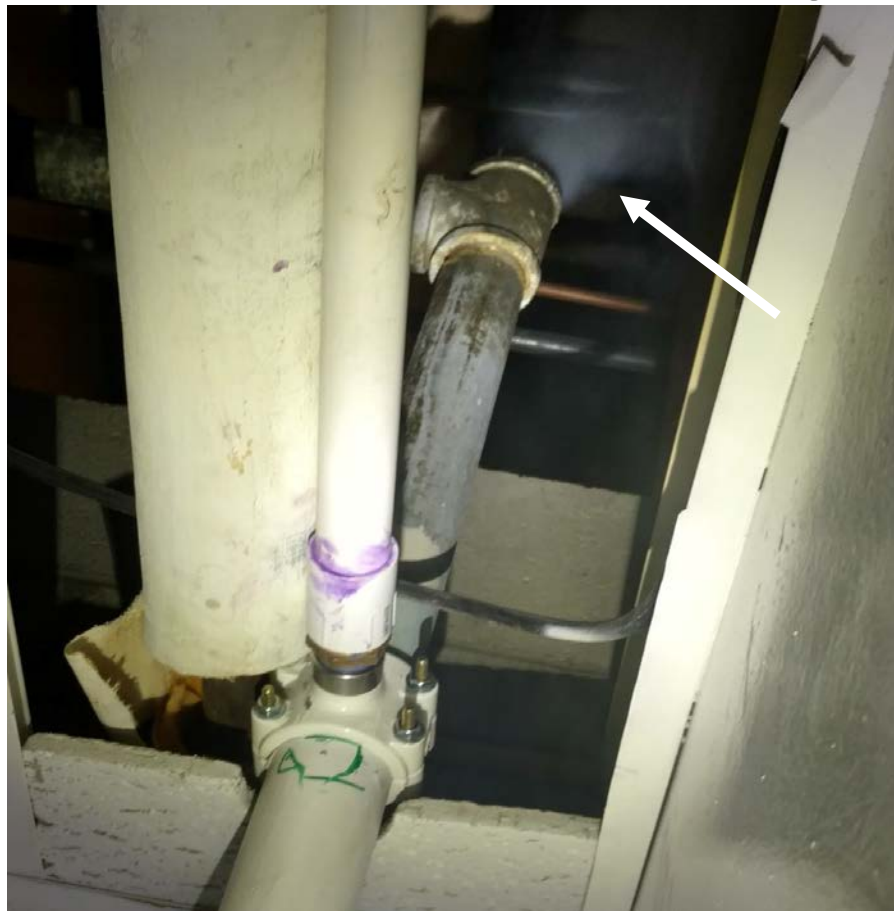
Sanitary Sewer Line Above Suspended Ceiling
