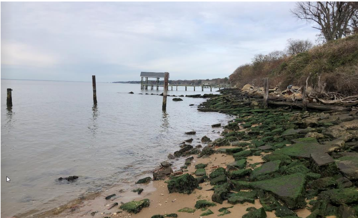
Figure 3.4 Shoreline erosion and existing debris from the toe of the slope in the southern end of the project area
