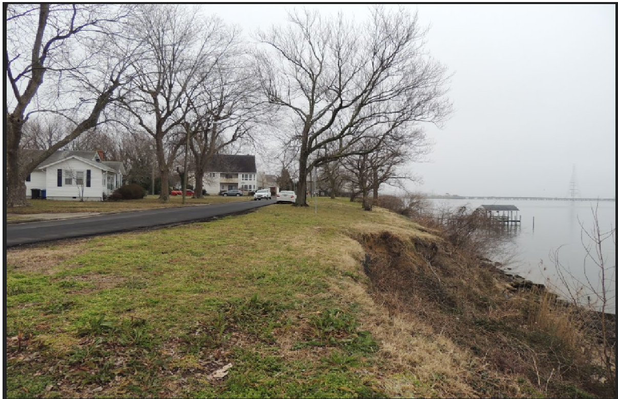
Figure 1-4. View facing southeast of project site and crack in ground surface along James River
