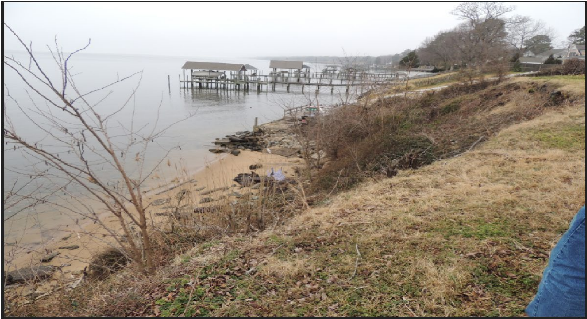
Figure 1-3. View facing northwest of eroding shoreline at project site along James River
