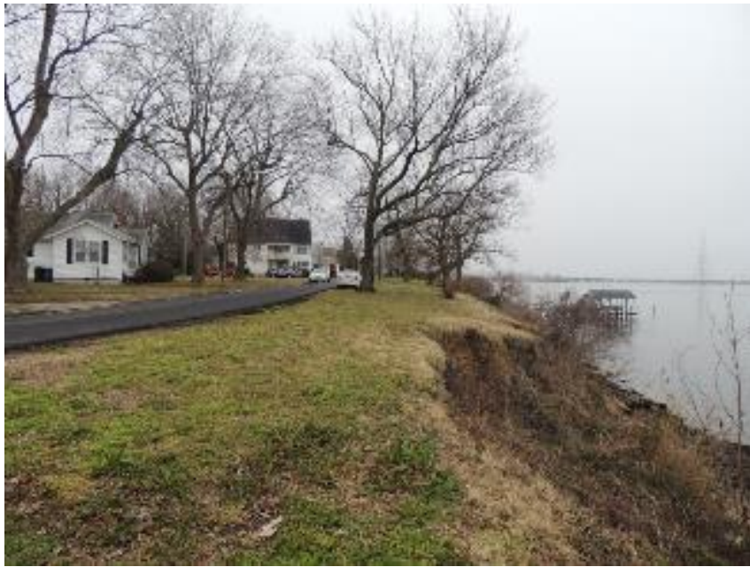
Figure 3.5 Shoreline erosion from the top of the bank in the northern end of the project area
