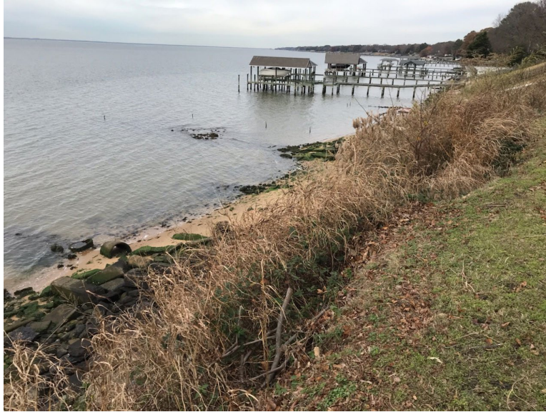
View of James River at northern extent of project site. Image taken 12/06/2019.
