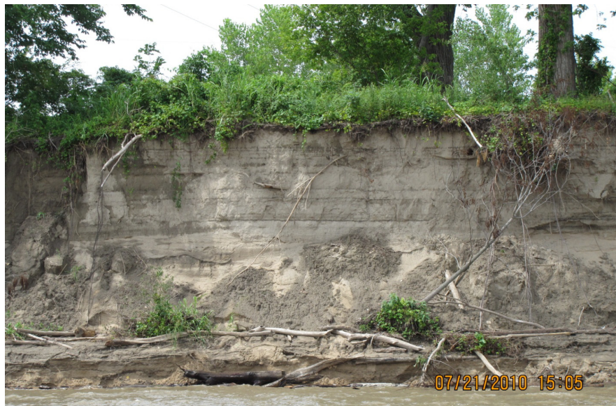
Figure 3. 21. Vertical eroding bank just downstream of the Johnson County Water One Weir.
