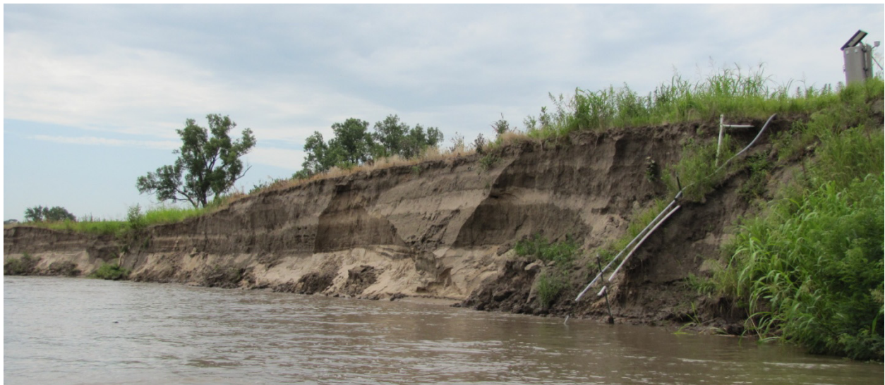
Figure 3. 2. An eroding, vertical bank. RM 167.8.
