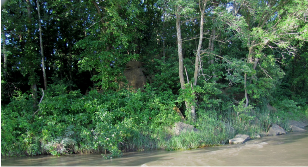
Figure 3. 6. Riprap on banks is overgrown with vegetation. RM 102.2.
