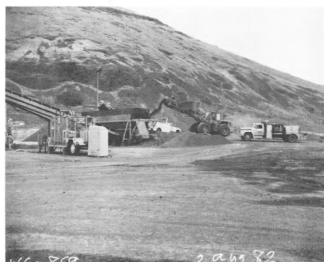
CHARGING AGGREGATES USING A FRONT END LOADER AND CONVEYOR THAT FEEDS THE WEIGH BINS.
