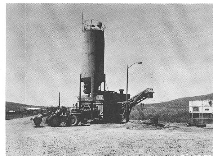
CEMENT SILO AND CHARGING BELT FROM WEIGH BINS TO MIXER TRUCKS.
