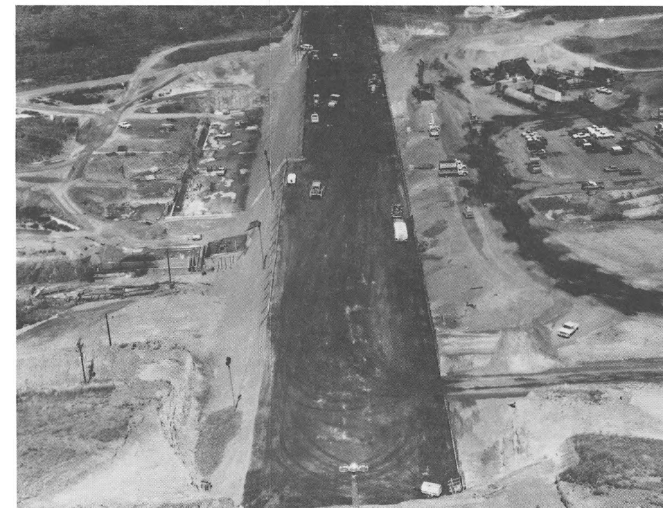
OVERALL VIEW OF THE EQUIPMENT SPREAD. JULY 20, 1982. NOTE THE UNDESIRABLE EQUIPMENT TIRE TRACKS. ALSO NOTE THE MINIMAL EQUIPMENT AND PERSONNEL REQUIREMENTS DURING PEAK PRODUCTION.
