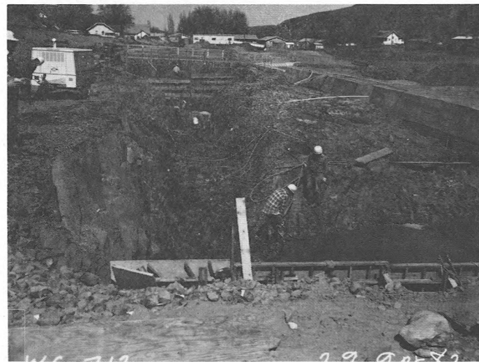
DIVERSION PIPE ENCASED IN CONCRETE TO THE RIGHT. EXCAVATION FOR PERMANENT OUTLET TO THE LEFT.
