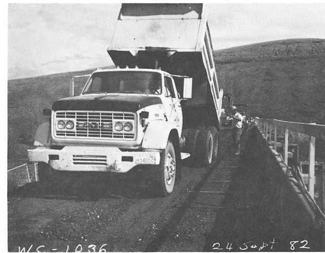
DUMP TRUCK USED IN NARROW AREAS AT THE TOP OF THE DAM.
