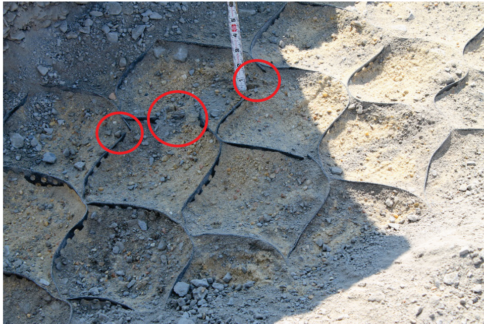
Figure 6-2. Damage to the 8-in.-height geocells in Repair 1-A after 13 passes.
